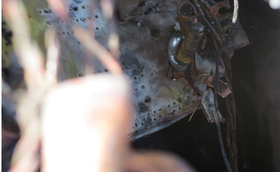
Figure 7: Photograph of fire damaged ECM circuit board.
