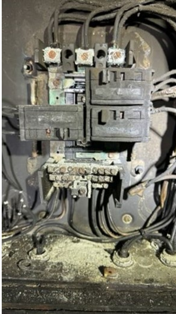
Photograph 1. Circuit breaker box at bottom of rear quarters stairs, port side. Circuit breaker/s and wires associated with the two failed outlets along some other wires were removed by owner's insurance company representatives.
