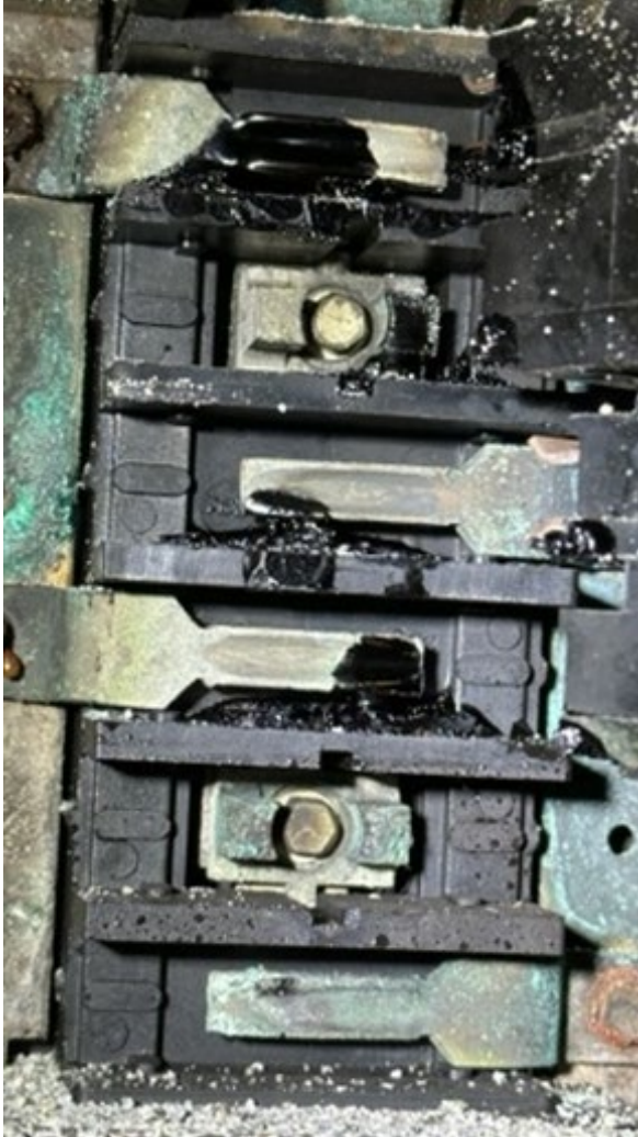
Photograph 2. Portside circuit breaker box, breakers removed. Upper left mounting position had melted plastic from the breakers at the box/breaker contact points.
