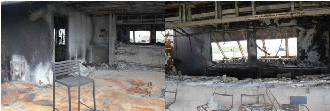
Third Deck Damage
