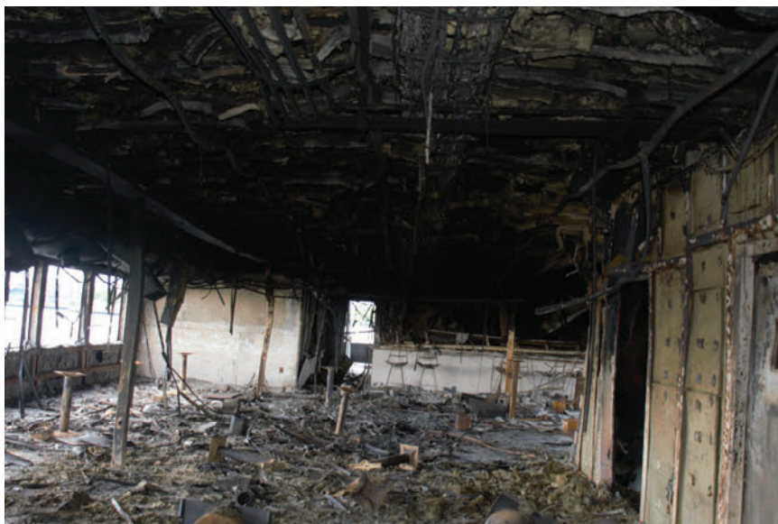
Second Deck Interior Damage
