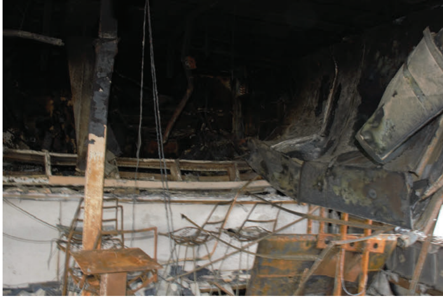
Second Deck Bar Area Damage
