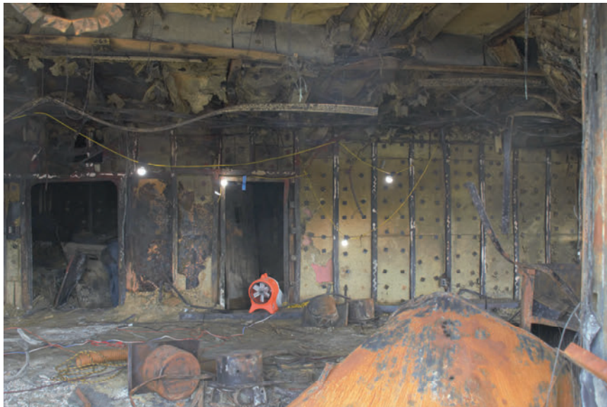
Main/First Deck Cabin Damage
