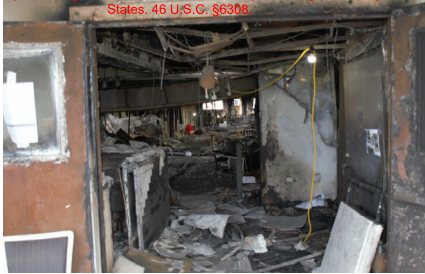
Rear Interior Damage
