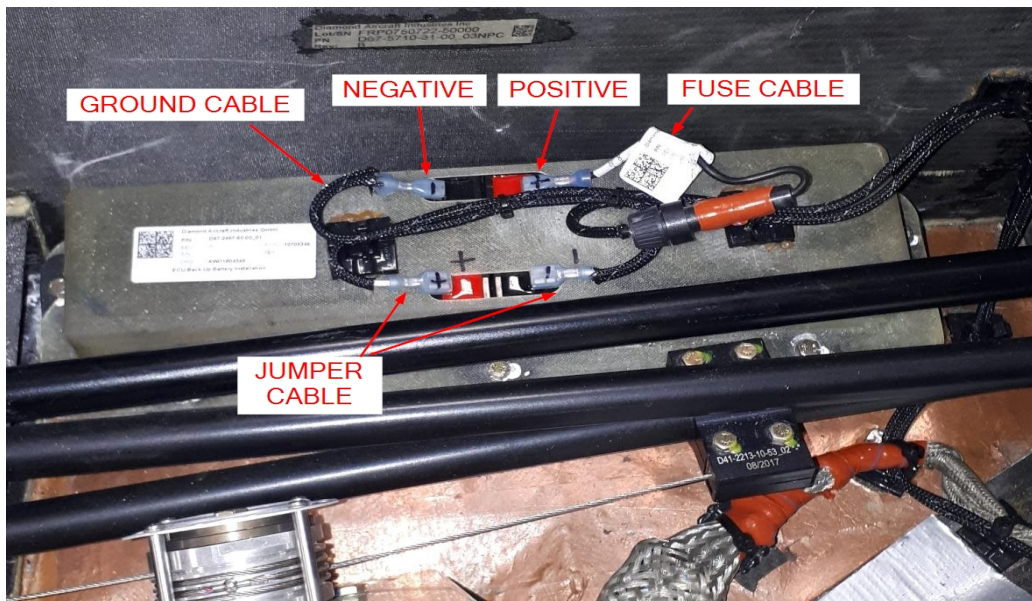
Figure 5. RH battery (cables connected).
