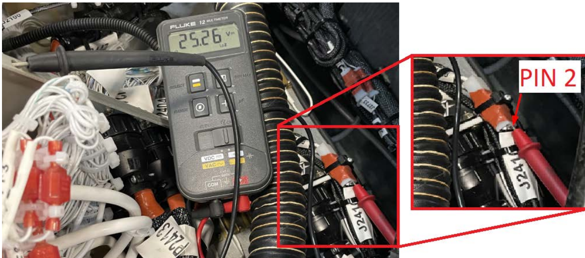
Figure 2. Voltage check of pin 2.
