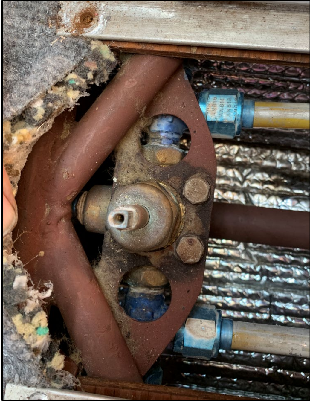
Figure 1 – View of the installed fuel selector.
