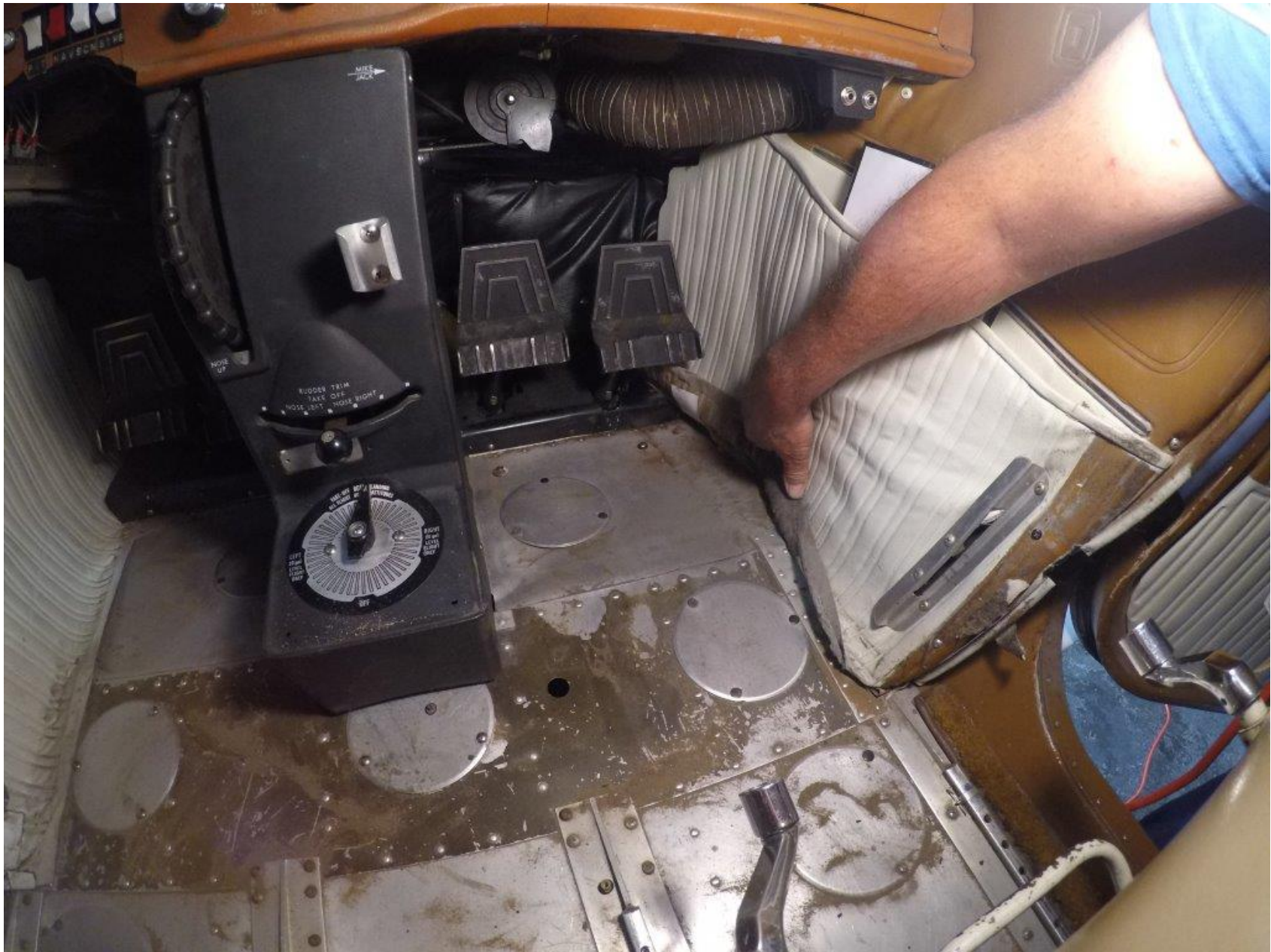
Photo 2 – Damage to Interior Floorboards on Passenger Side
