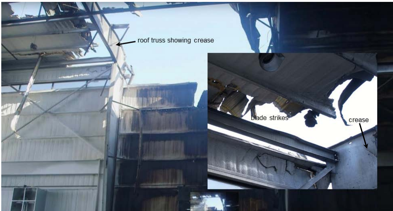
Figure 5. View of the entry hole orienting the location of the crease in the roof truss
