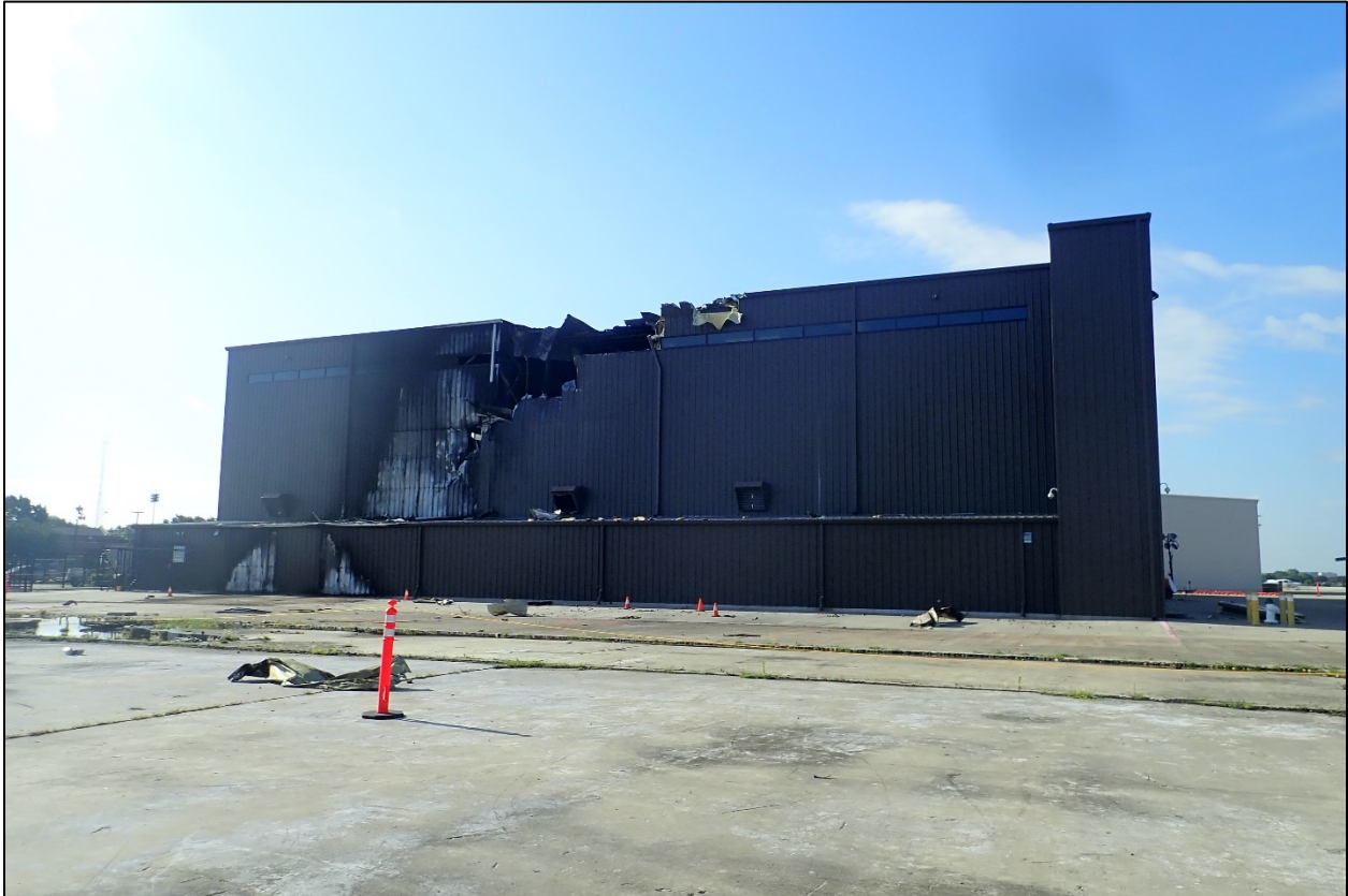
Figure 2 - Side of hangar with initial impact site (at top of wall).
