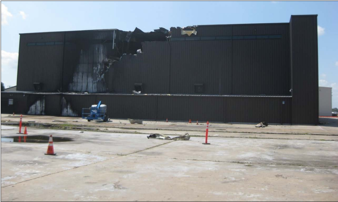
Figure 5 - Ramp area outside hangar, with airplane debris.
