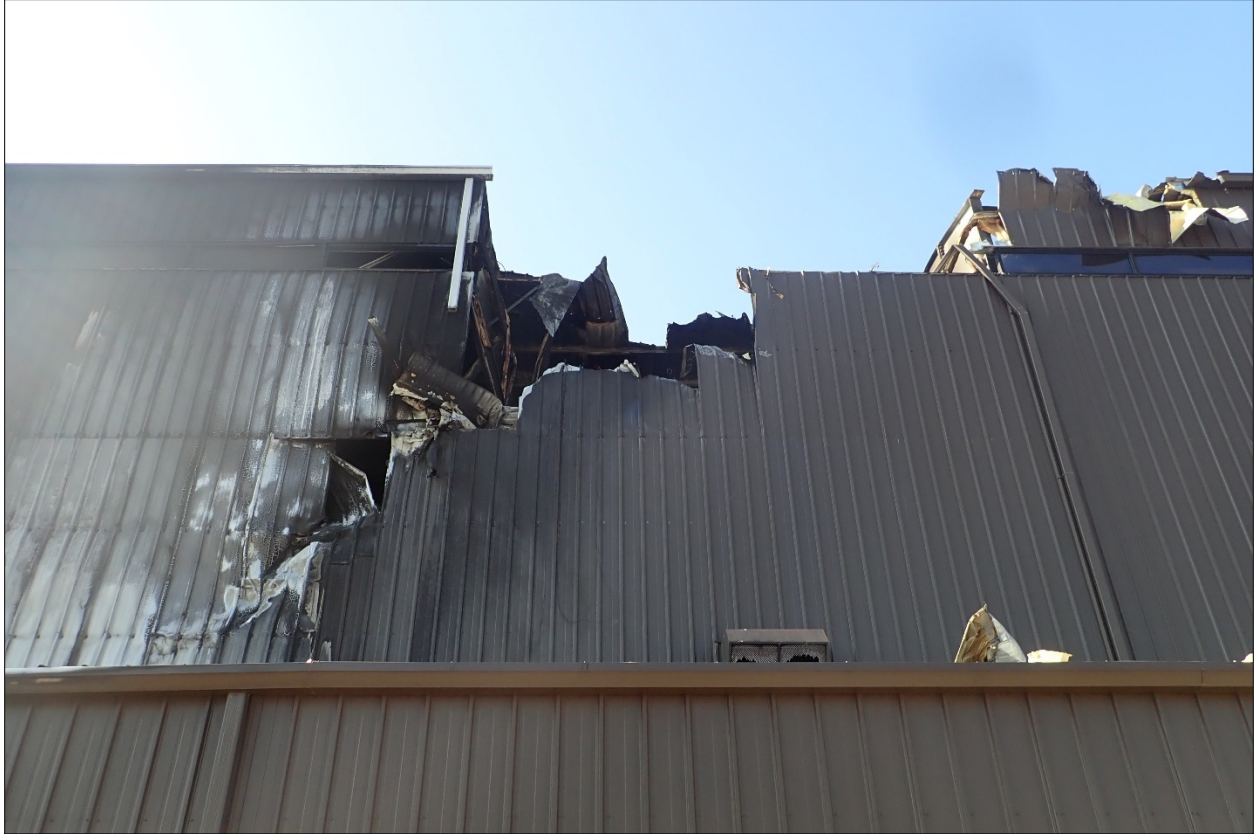
Figure 3 - Close up detail of initial impact location.
