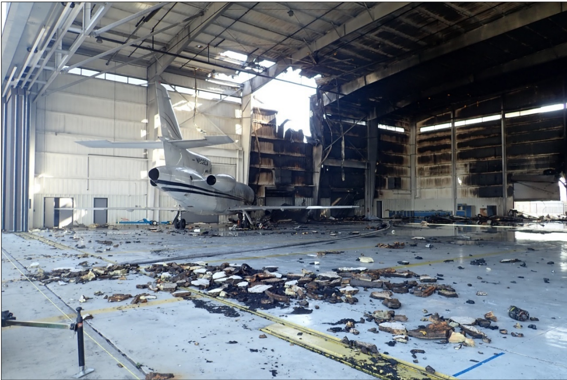
Figure 7 - Airplane and hangar debris located inside hangar.
