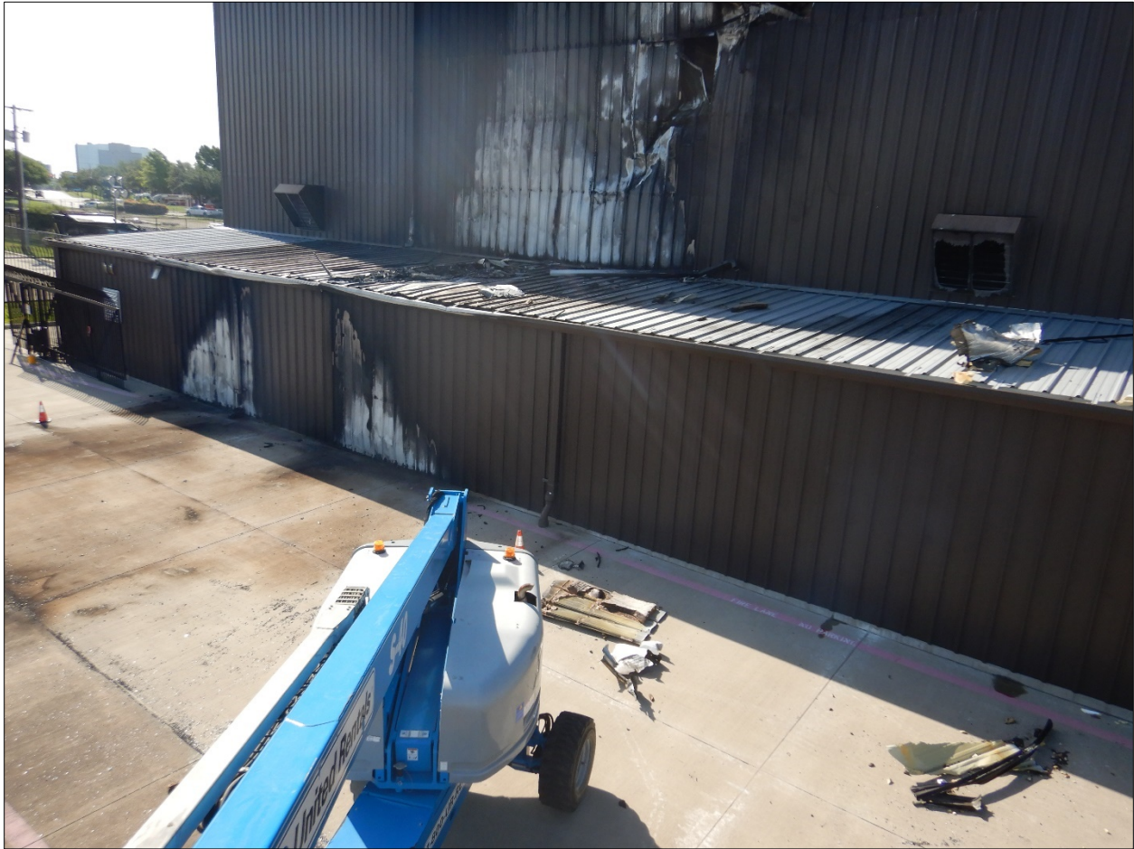
Figure 4 - Lower roof area with airplane debris.
