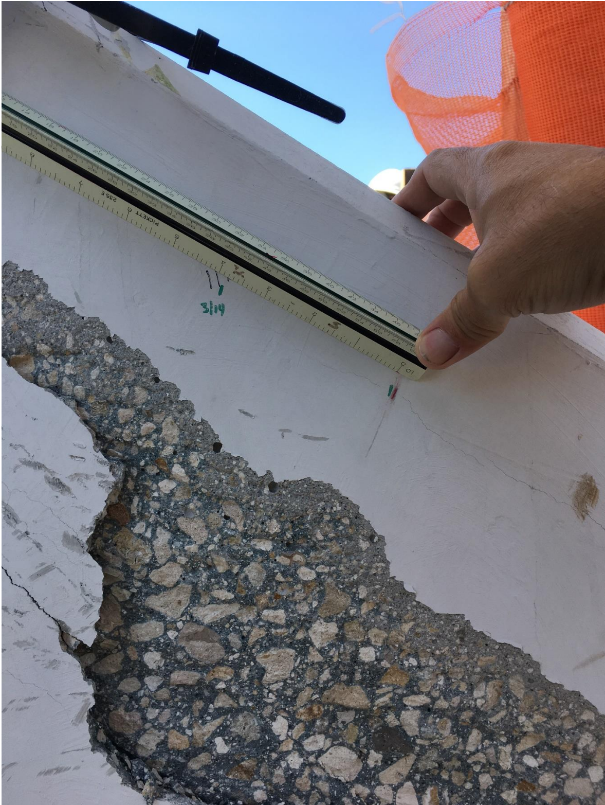
Bridge Factors Photo 89 – View of crack being monitored at the bottom of diagonal support #11 on east side looking to the west on 3/14/18 at 1:42 p.m. (Source: Bolton – Perez and Associates, BPA)
