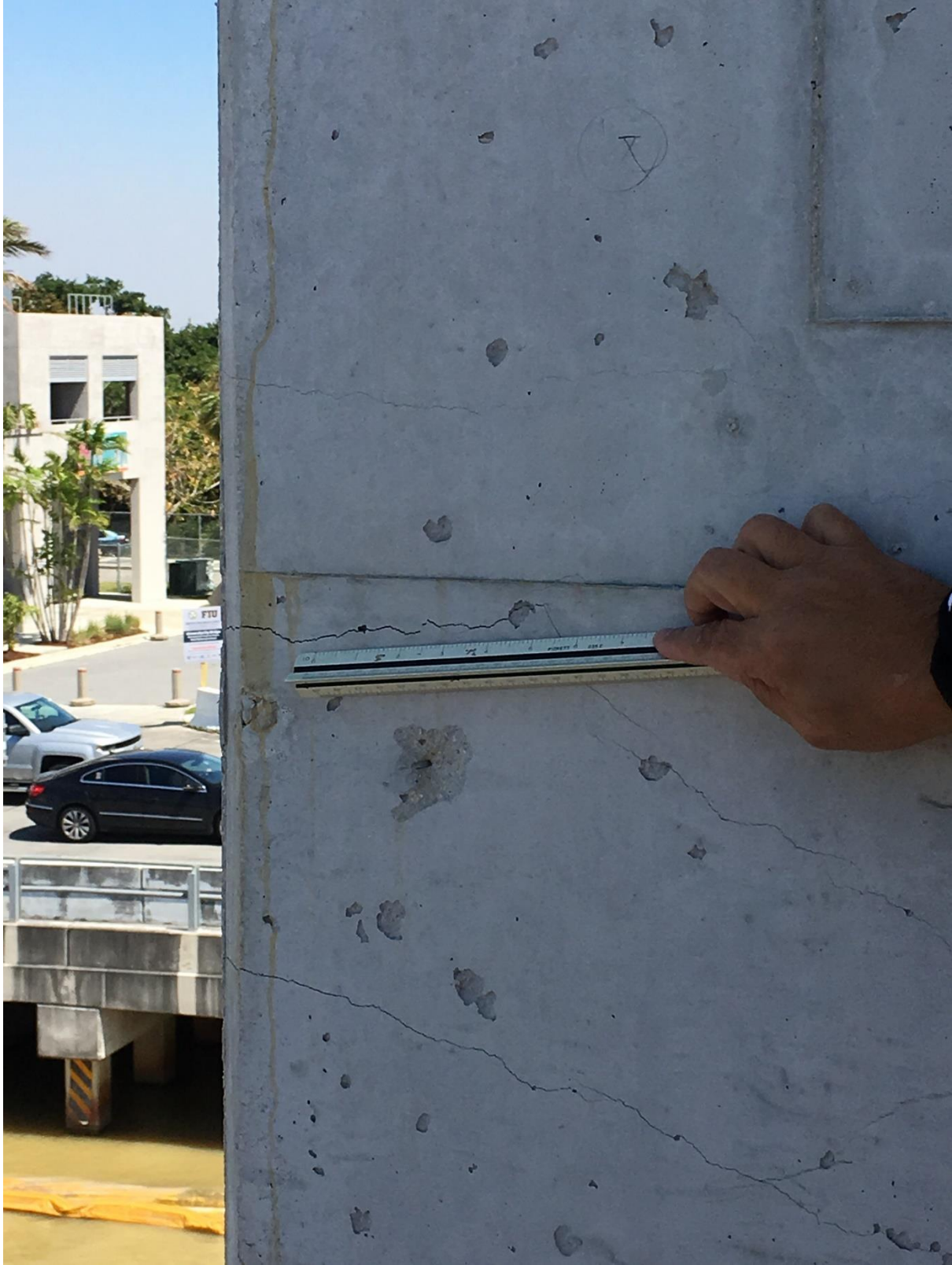
Bridge Factors Photo 101 – View of crack being monitored on the west side of vertical support #12 looking to the east on 3/14/18 at 1:51 p.m. (Source: Bolton – Perez and Associates, BPA)
