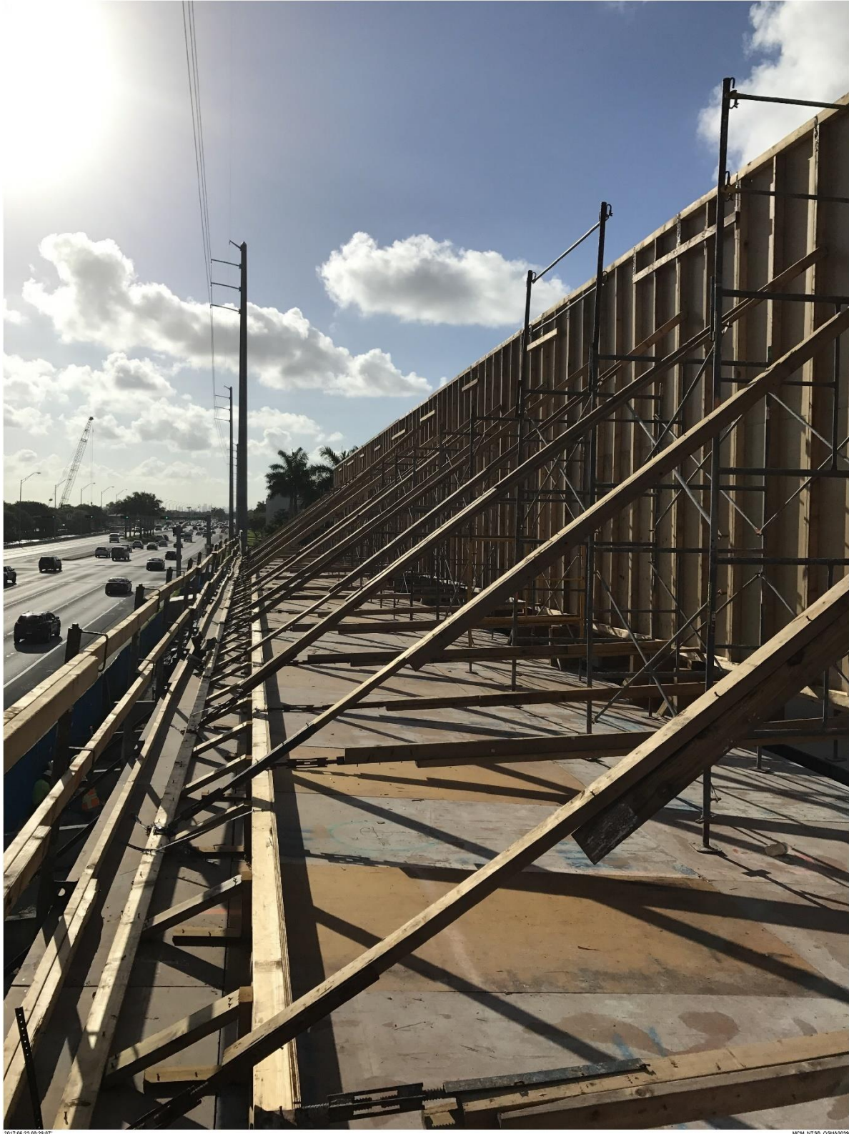
Bridge Factors Photo 5 – View of initial formwork being set up for diagonal supports of main span on 6/23/17 at 8:29:07 a.m. (Source: Munilla Construction Management, MCM)
