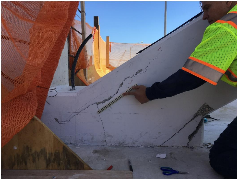
Bridge Factors Photo 83 – View of cracks at the bottom of diagonal support #11 on west side looking to the east on 3/13/18 at 1:17:46 p.m. (Source: Munilla Construction Management, MCM)
