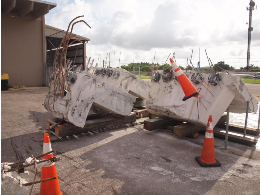
Bridge Factors Photo 110 – View of bridge deck in the vicinity of Node #11 and #12 with center section cut and slid forward for viewing of sample’s internal areas looking to the northeast in FDOT South Dade Maintenance Yard
