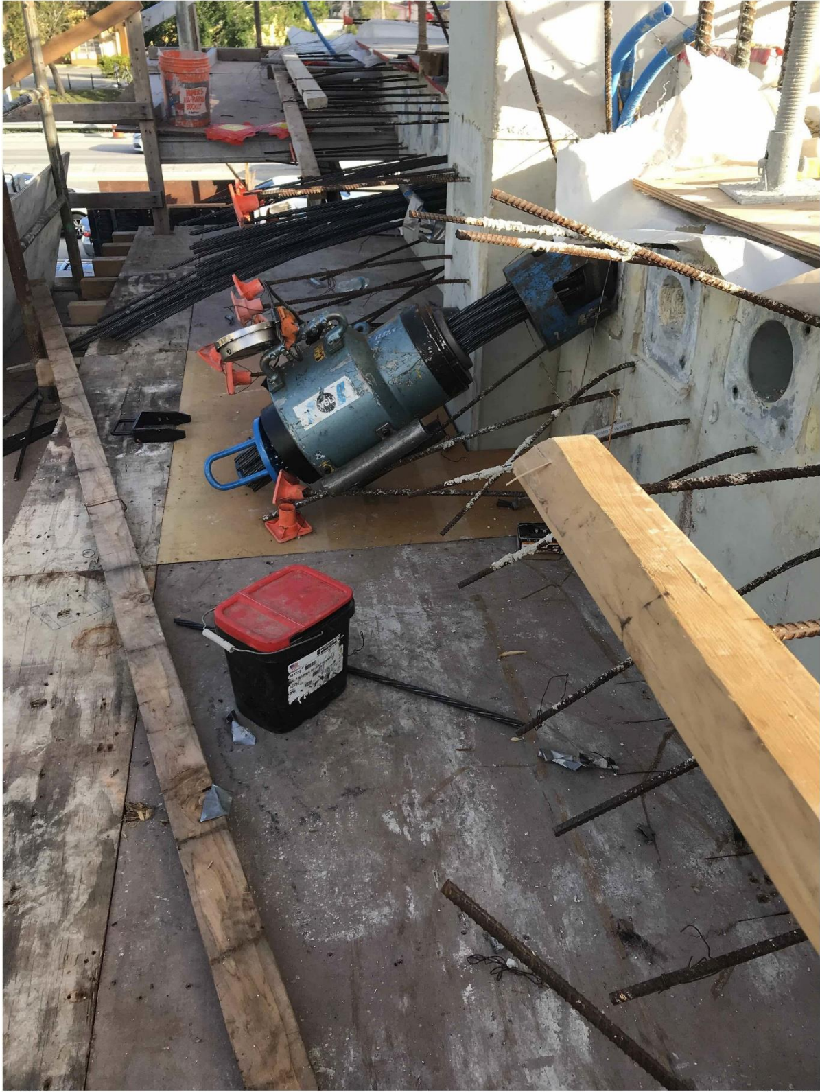
Bridge Factors Photo 27 – View of stressing deck longitudinal tendons D1 on 1/16/18 at 8:35:52 a.m. (Source: Munilla Construction Management, MCM)
