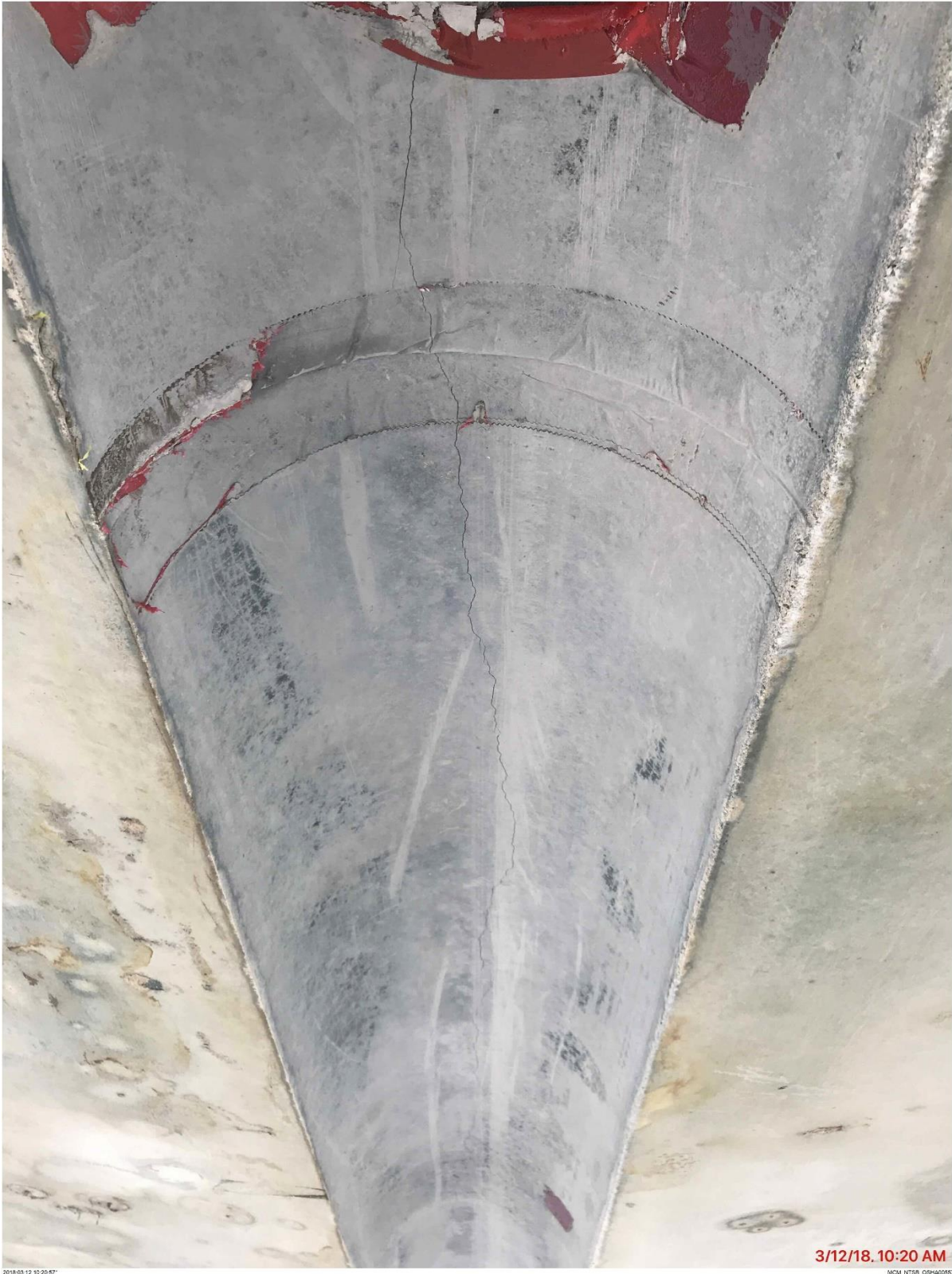
Bridge Factors Photo 71 – View of crack in cut-out for drain pipe under deck on 3/12/18 at 10:20 a.m. (Source: Munilla Construction Management, MCM)
