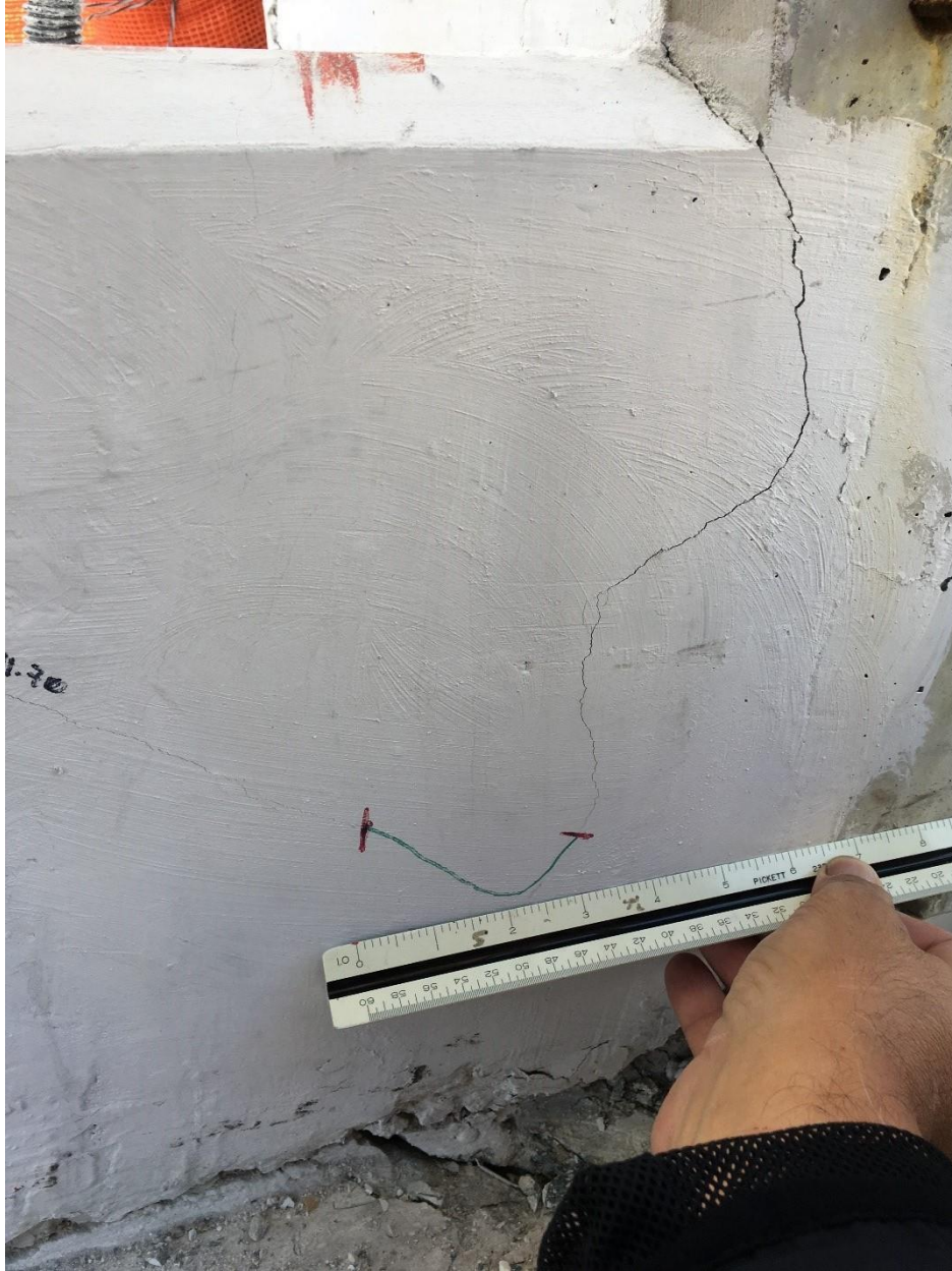
Bridge Factors Photo 91 – View of crack being monitored at the bottom of diagonal support #11 and vertical support #12 on east side looking to the west on 3/14/18 at 1:42 p.m. (Source: Bolton – Perez and Associates, BPA)
