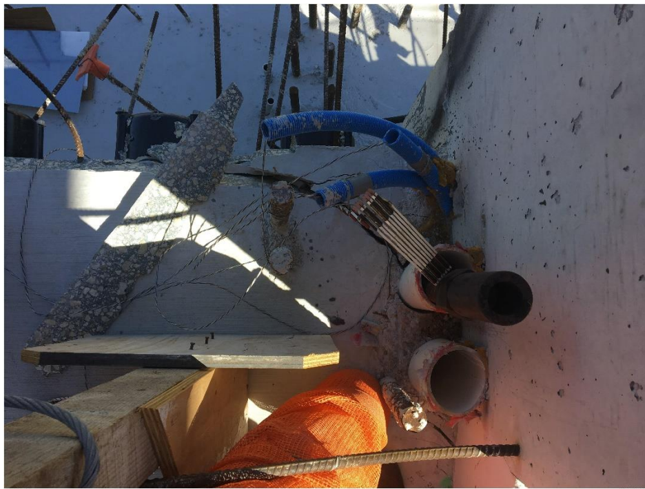
Bridge Factors Photo 75 – Top view of cracks along west side of Diaphragm II on 3/13/18 at 11:17:04 a.m. (Source: Munilla Construction Management, MCM)
