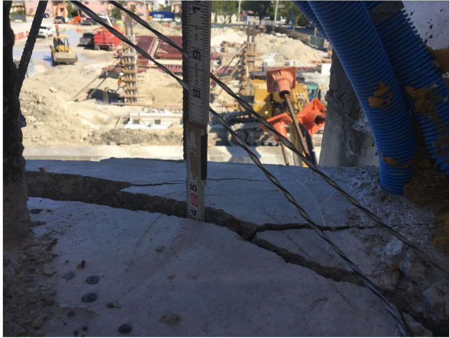
Bridge Factors Photo 74 – View of cracks along west side of Diaphragm II looking to the north showing crack is approximately 4 inches deep on 3/13/18 at 11:16:50 a.m. (Source: Munilla Construction Management, MCM)
