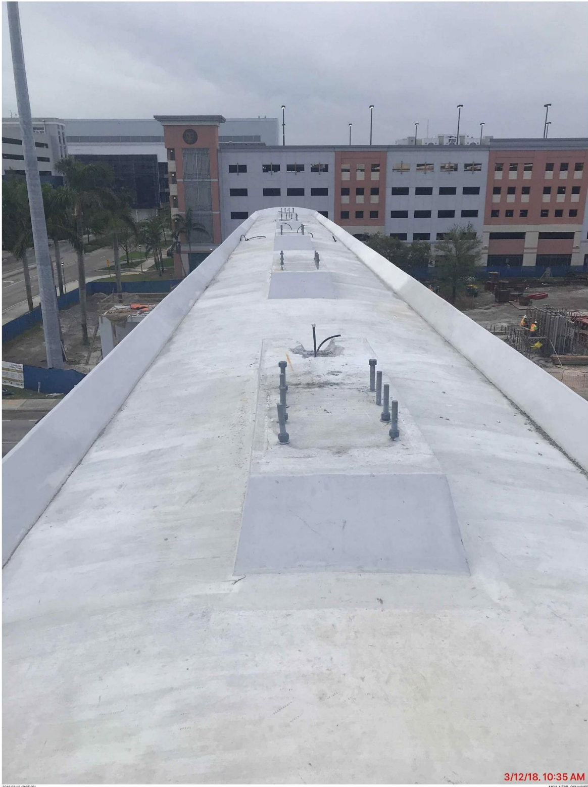
Bridge Factors Photo 73 – View of top of canopy looking to the south and chiseled concrete in blister for destressing diagonal support #11 on 3/12/18 at 10:35 a.m. (Source: Munilla Construction Management, MCM)
