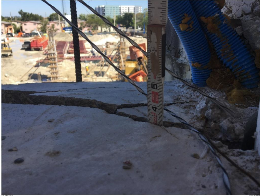
Bridge Factors Photo 76 – View of cracks along west side of Diaphragm II looking to the north showing crack is approximately 3 inches deep on 3/13/18 at 11:17:57 a.m. (Source: Munilla Construction Management, MCM)
