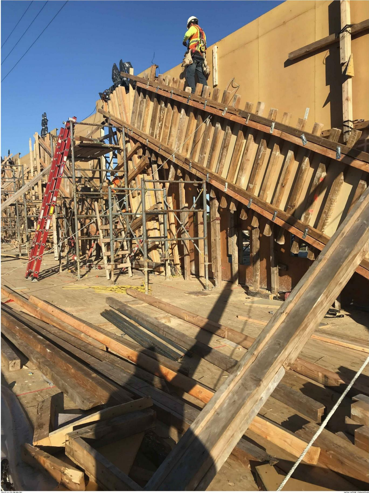
Bridge Factors Photo 13 – View of setting forms for diagonal supports prior to pouring of concrete on 11/3/17 at 8:59:28 a.m. (Source: Munilla Construction Management, MCM)
