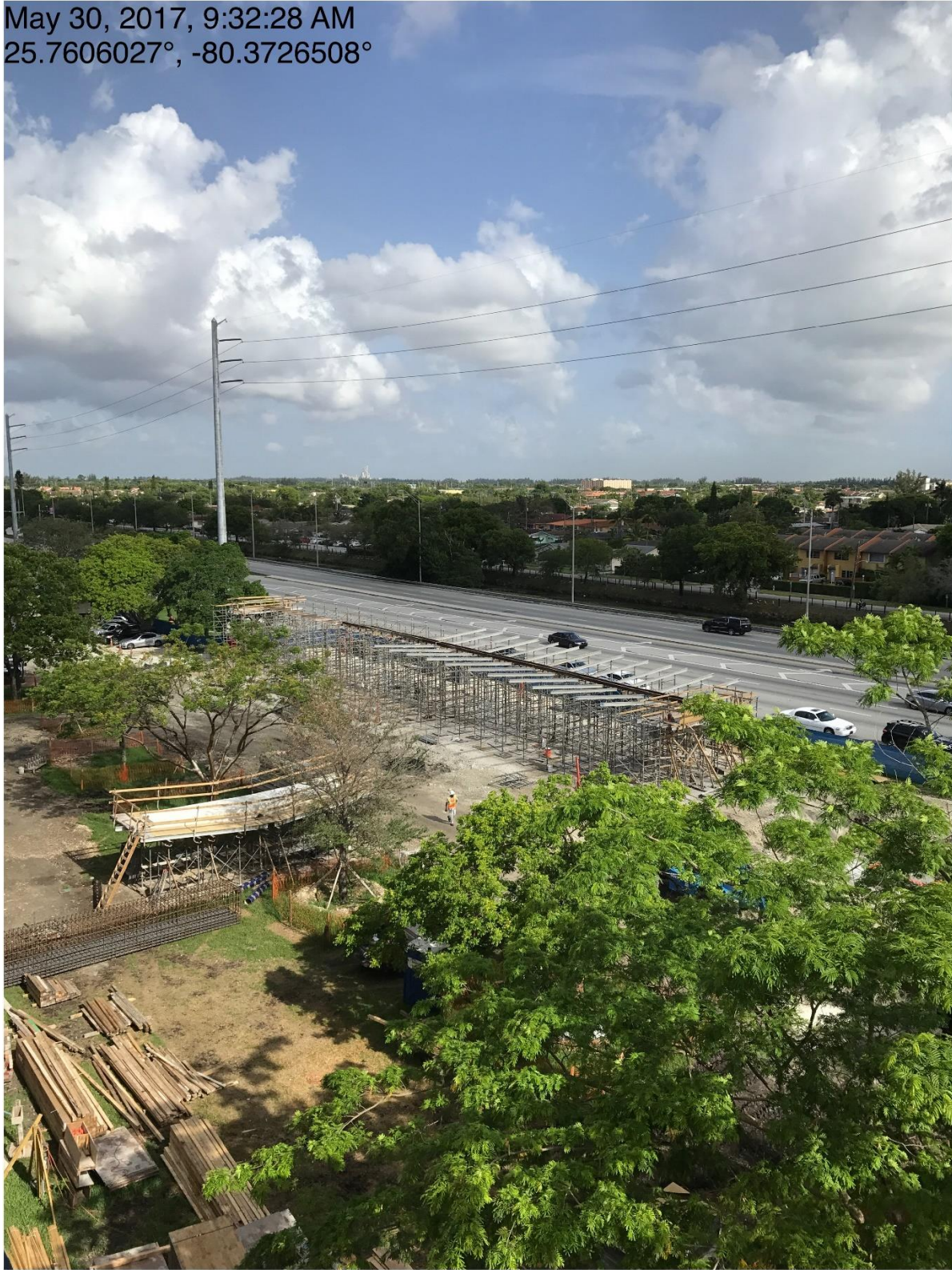
Bridge Factors Photo 3 – View of falsework being set up in adjacent casting yard for construction of main span on 5/30/17 at 9:32:28 a.m. (Source: Munilla Construction Management, MCM)
