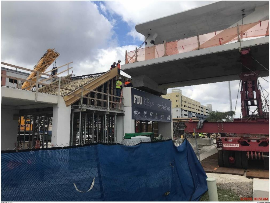
Bridge Factors Photo 57 – View of Diaphragm I, south end of main span, just prior to placement on south pier looking to the west on 3/10/18 at 10:23 a.m. (Source: Munilla Construction Management, MCM)
