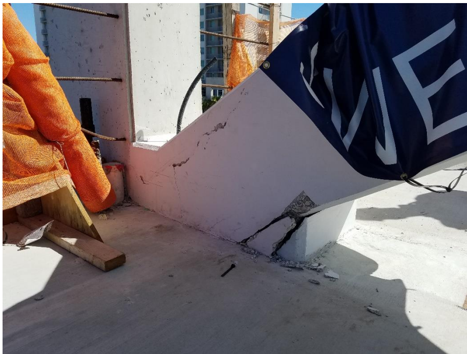
Bridge Factors Photo 103 – View of cracks at the bottom of diagonal support #11 on west side looking to the northeast on 3/15/18 at 10:55 a.m. (Source: FIU Associate Vice-President of Facilities Management)
