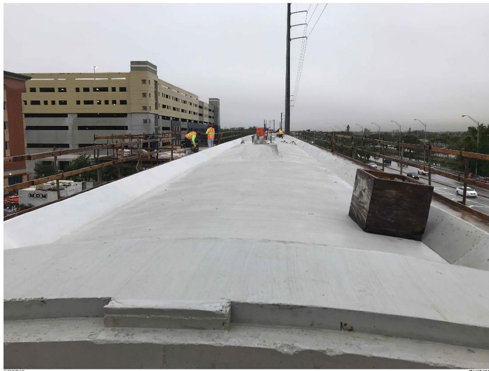
Bridge Factors Photo 26 – View of finished poured concrete section of canopy on 1/3/18 at 7:49:26 a.m. (Source: Munilla Construction Management, MCM)
