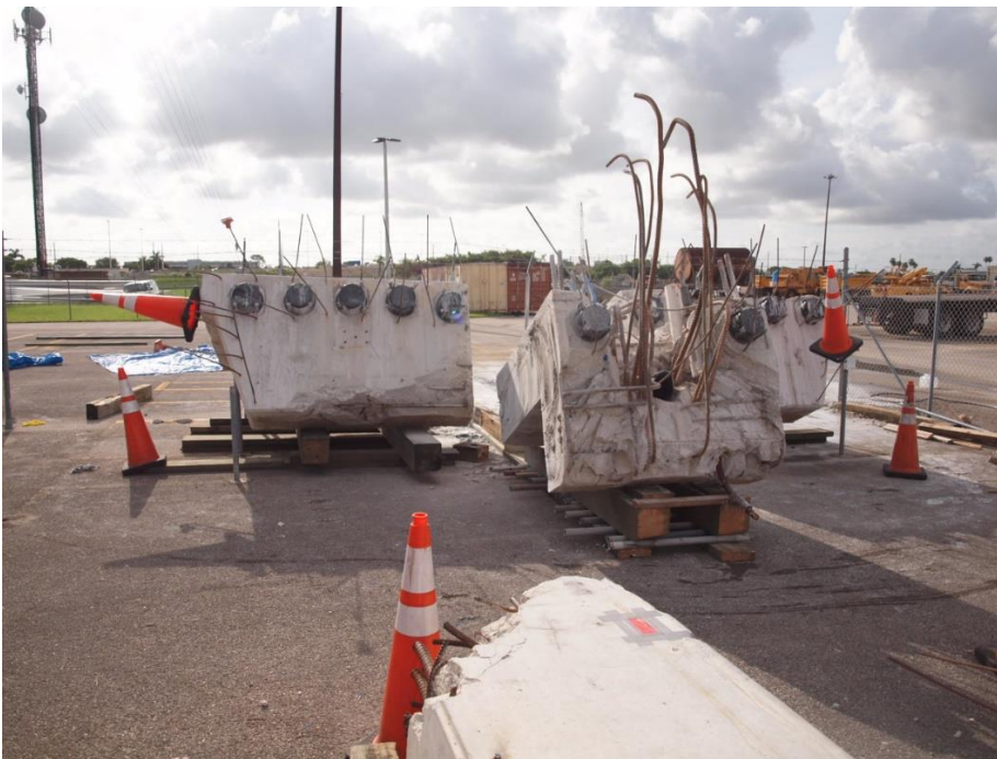
Bridge Factors Photo 111 – View of bridge deck in the vicinity of Node #11 and #12 with center section cut and slid forward for viewing of sample’s internal areas looking to the east in FDOT South Dade Maintenance Yard
