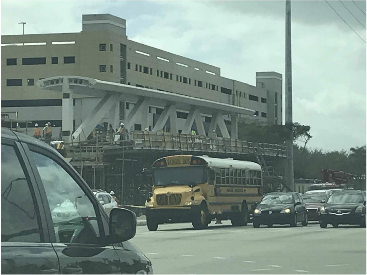
Bridge Factors Photo 34 – View of falsework removed under canopy on 2/22/18 at 2:23:44 p.m. (Source: Munilla Construction Management, MCM)
