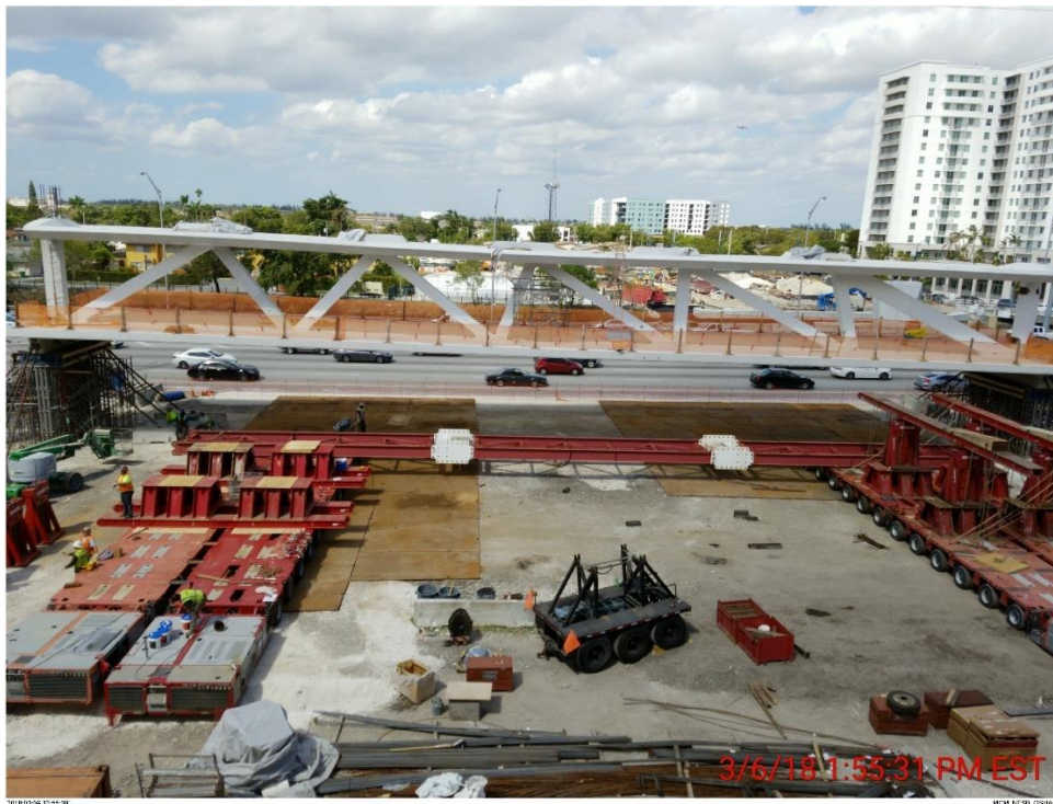
Bridge Factors Photo 48 – View of main span with partial set up of SPMT units located in foreground on 3/6/18 at 1:55:31 p.m. (Source: Munilla Construction Management, MCM)
