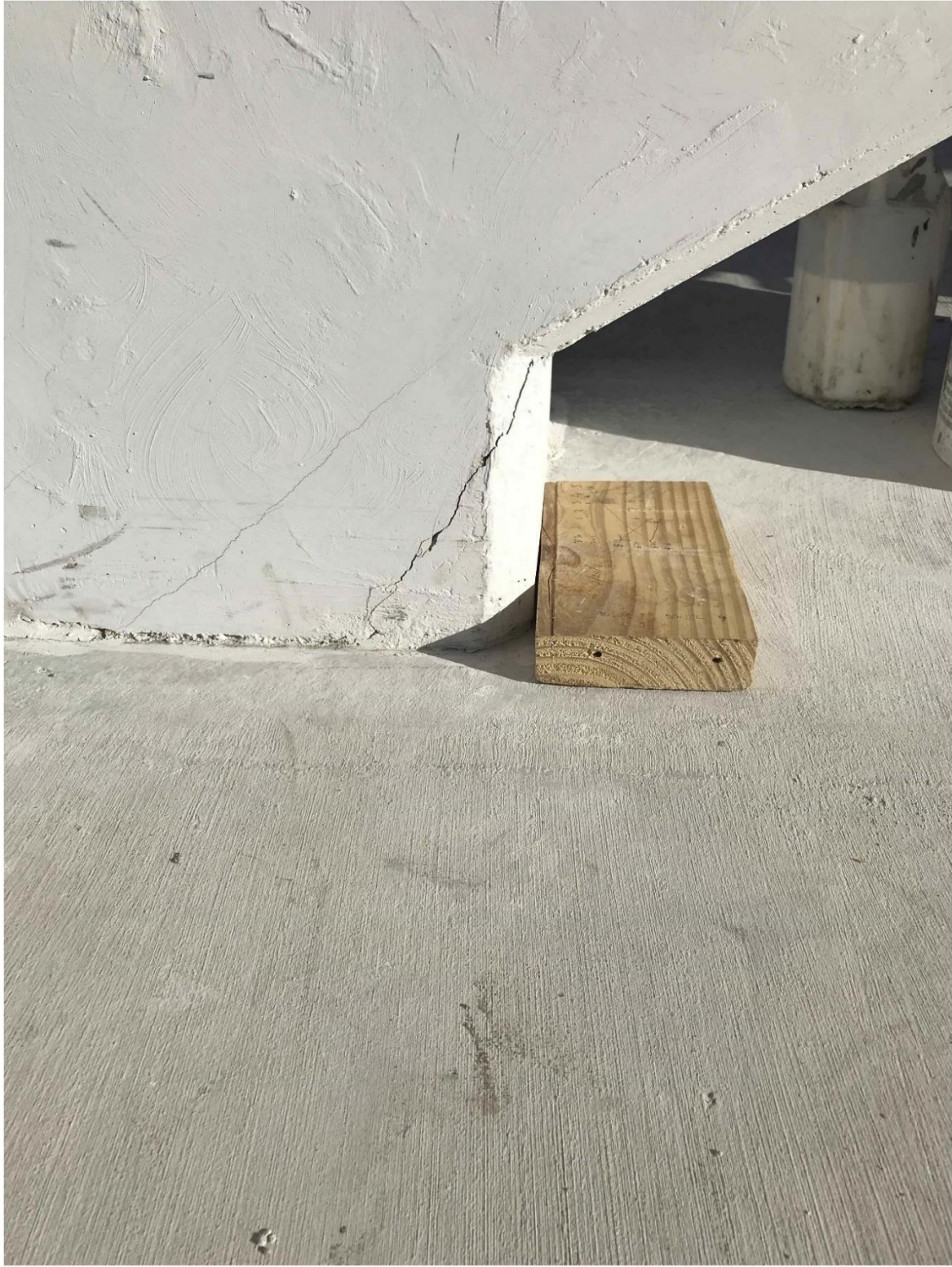
Bridge Factors Photo 43 – View of crack at the bottom of diagonal support #11 on south side looking to the north in casting yard on 2/26/18 at 8:38:58 a.m. (Source: Munilla Construction Management, MCM)
