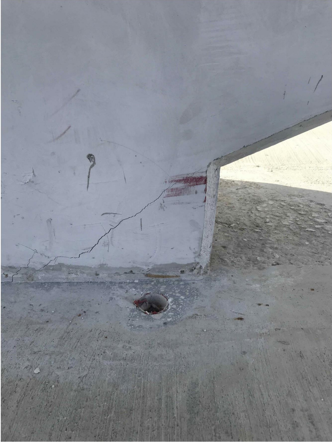
Bridge Factors Photo 45 – View of crack at the bottom of diagonal support #2 on north side looking to the south in casting yard on 2/26/18 at 8:40:08 a.m. (Source: Munilla Construction Management, MCM)
