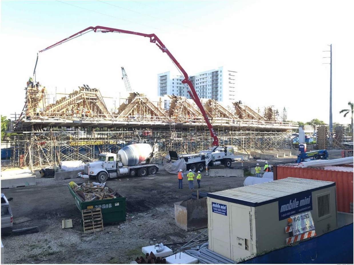
Bridge Factors Photo 14 – View of pouring of concrete in vertical #12 support on 11/6/17 at 7:47:01 a.m. (Source: Munilla Construction Management, MCM)
