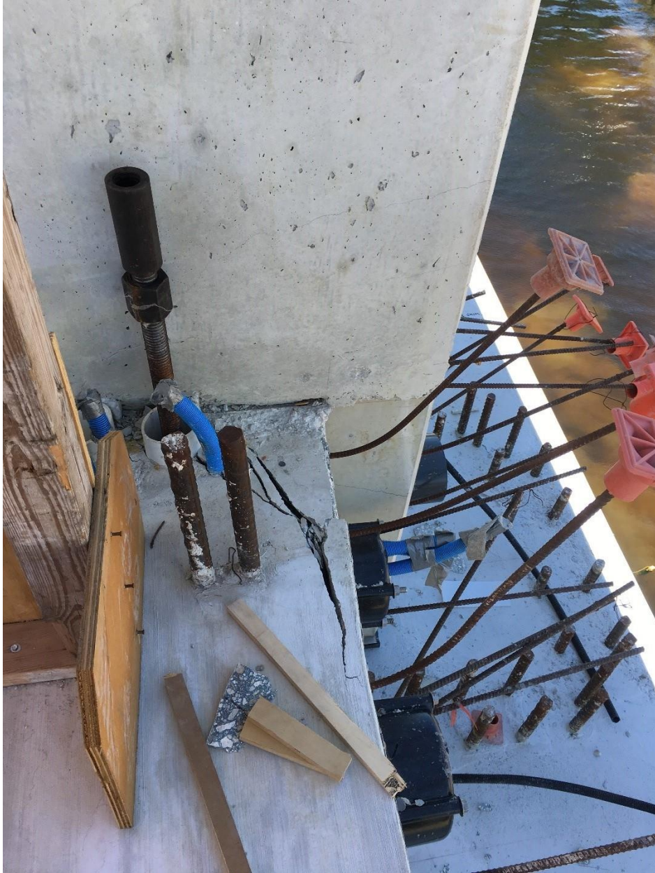
Bridge Factors Photo 96 – Top view of cracks along east side of Diaphragm II on 3/14/18 at 1:50 p.m. (Source: Bolton – Perez and Associates, BPA)
