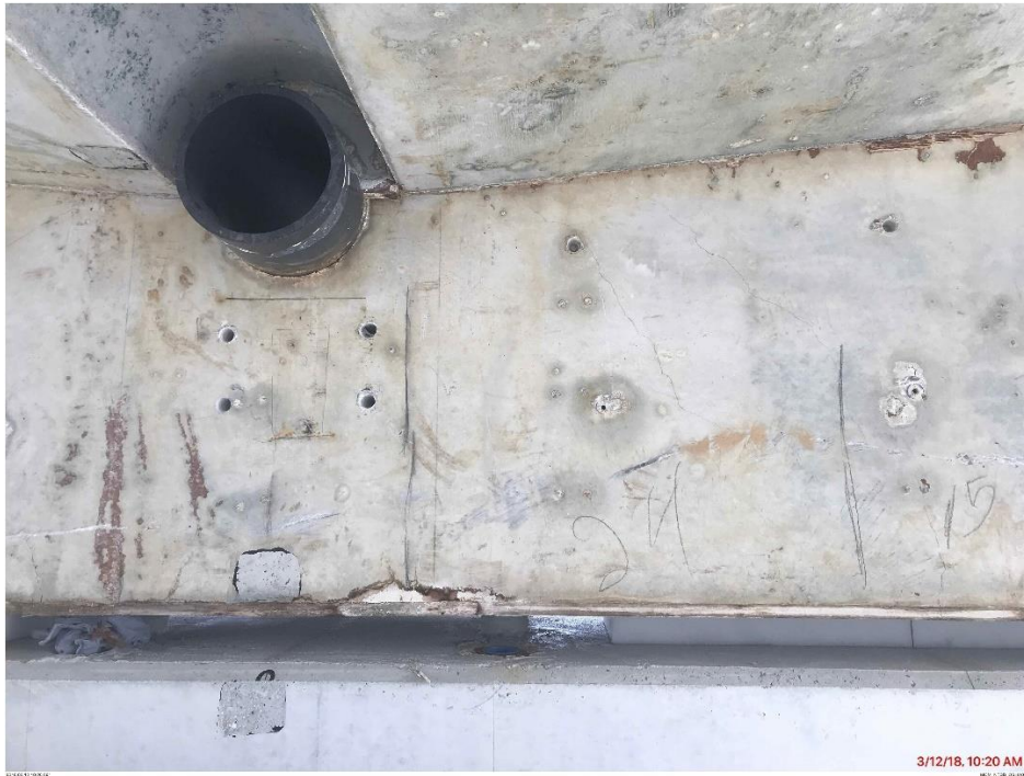
Bridge Factors Photo 70 – View of cracks on south face of Diaphragm II on east side on 3/12/18 at 10:20 a.m. (Source: Munilla Construction Management, MCM)
