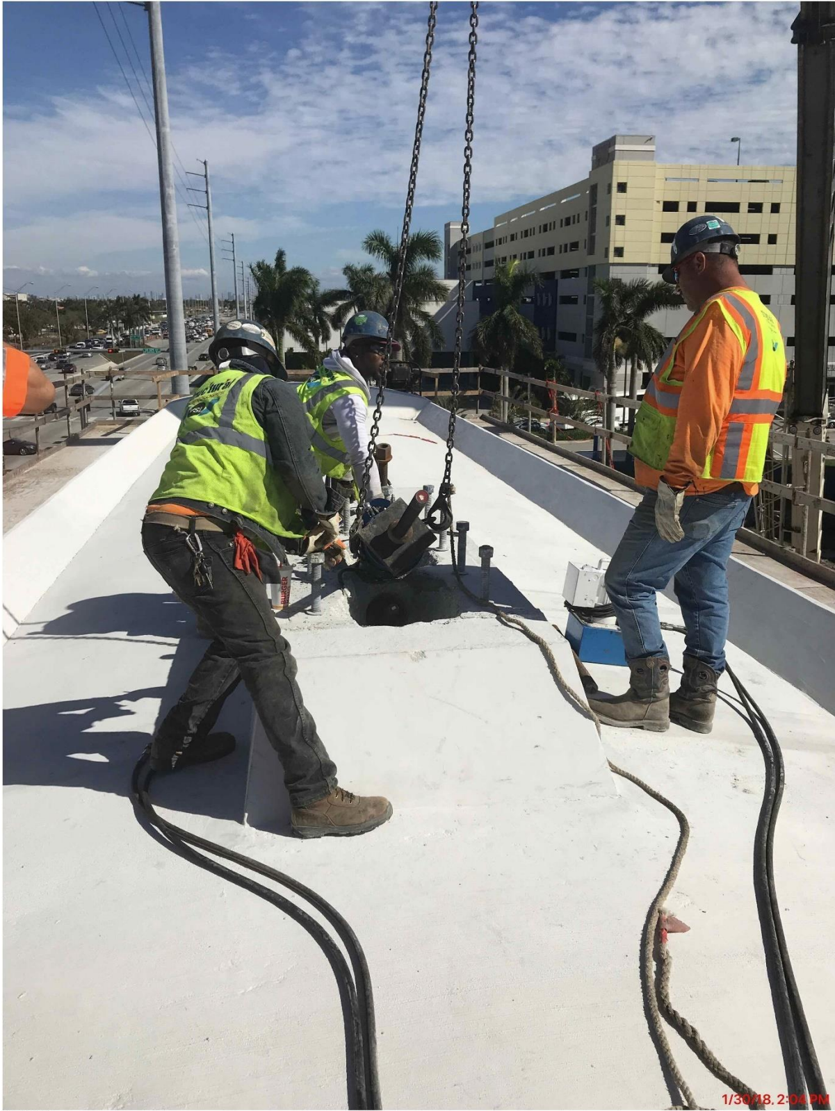
Bridge Factors Photo 28 – View of stressing post tensioning bar in diagonal support #2 on top of canopy on 1/30/18 at 2:04 p.m. (Source: Munilla Construction Management, MCM)
