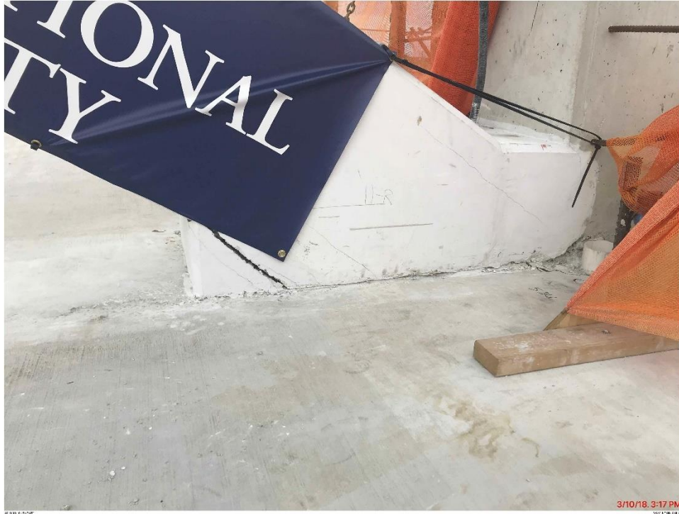
Bridge Factors Photo 64 – View of cracks at the bottom of diagonal support #11 on east side looking to the west on 3/10/18 at 3:17 p.m. (Source: Munilla Construction Management, MCM)
