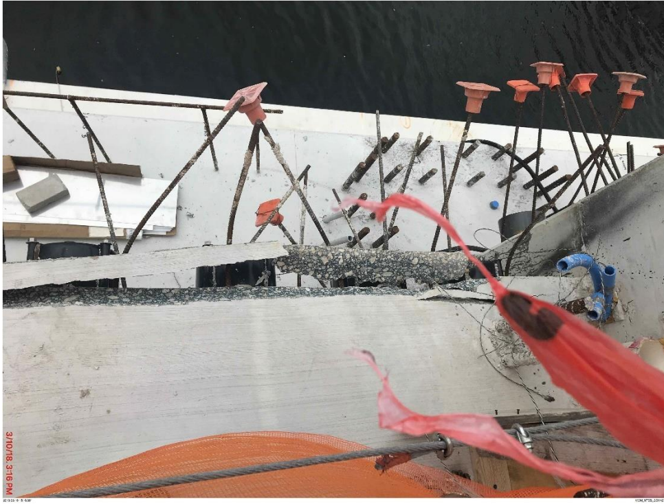
Bridge Factors Photo 63 – Top view of cracks along west side of Diaphragm II on 3/10/18 at 3:16 p.m. (Source: Munilla Construction Management, MCM)
