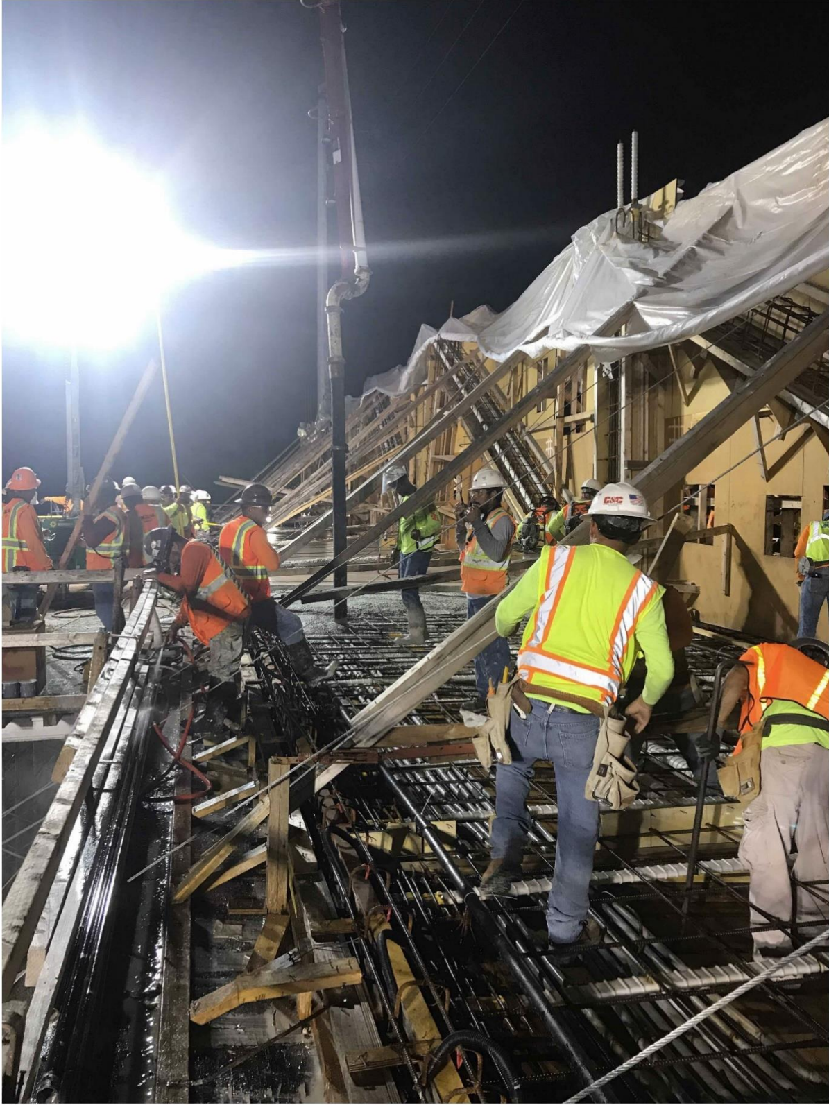
Bridge Factors Photo 11 – View of pouring the deck with concrete on 10/19/17 at 00:07:33 a.m. (Source: Munilla Construction Management, MCM)
