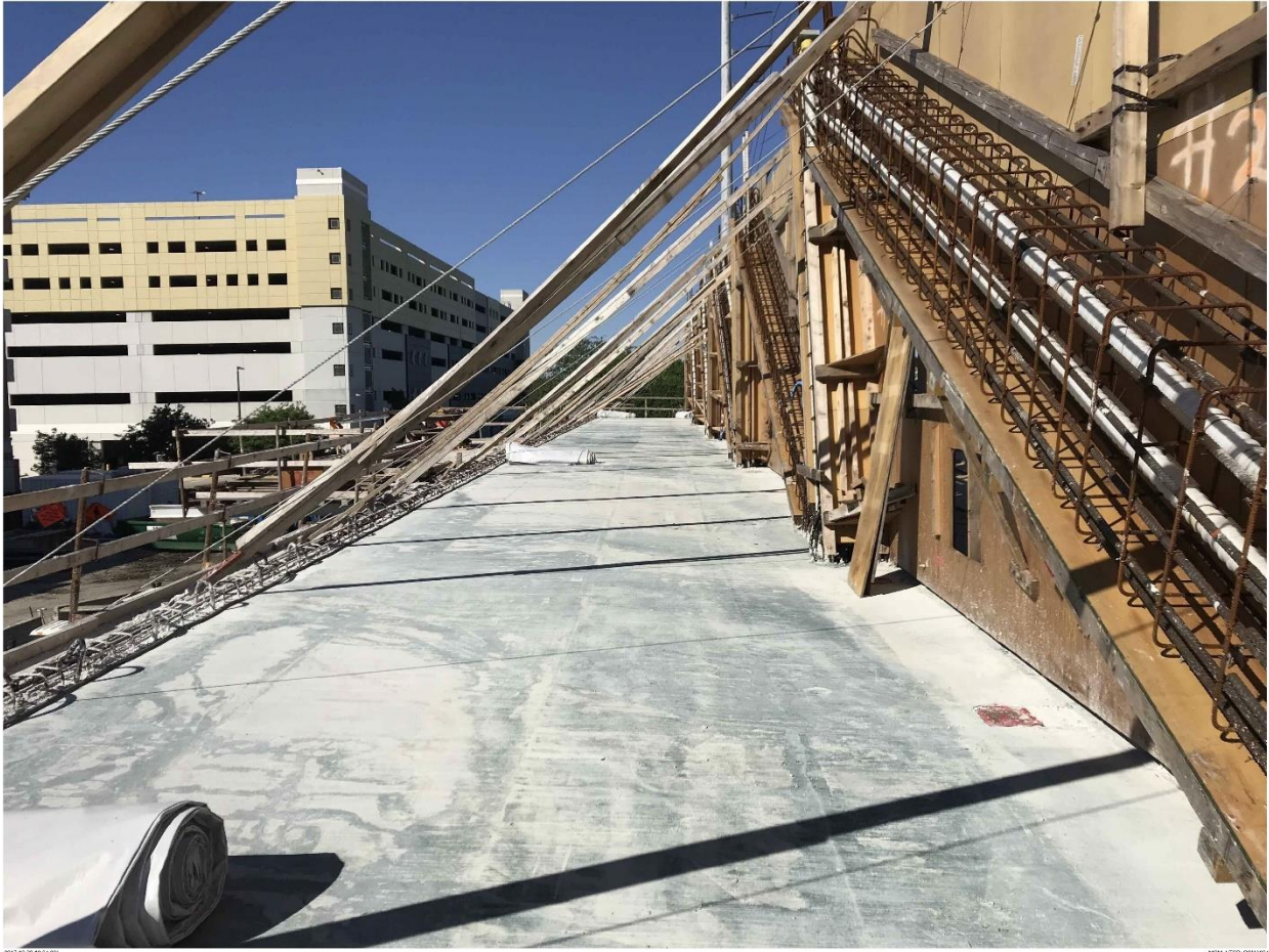
Bridge Factors Photo 12 – View of poured section of deck with concrete on 10/26/17 at 10:24:33 a.m. (Source: Munilla Construction Management, MCM)
