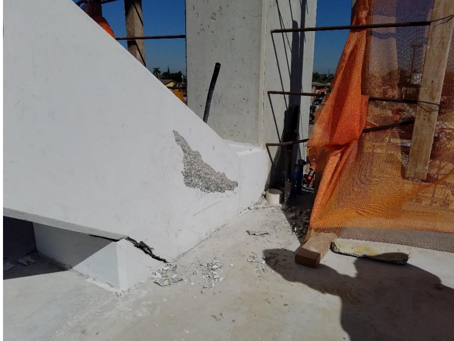
Bridge Factors Photo 102 – View of cracks and delamination at the bottom of diagonal support #11 on east side looking to the northwest on 3/15/18 at 10:53 a.m. (Source: FIU Associate Vice-President of Facilities Management)
