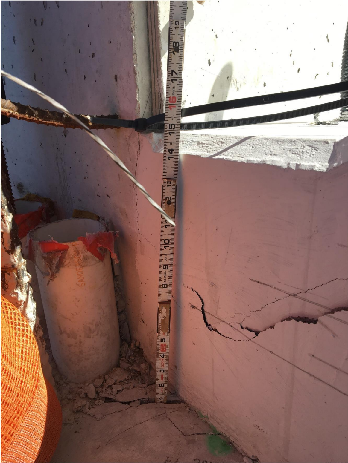
Bridge Factors Photo 79 – View of crack in Node #11/#12 region on west side showing crack is approximately 1 inch deep on 3/13/18 at 11:25:33 a.m. (Source: Munilla Construction Management, MCM)
