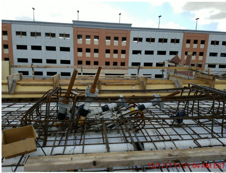
Bridge Factors Photo 24 – View of rebar for blister located on top of canopy on 12/1/17 at 11:21:04 a.m. (Source: Munilla Construction Management, MCM)
