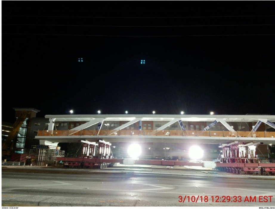
Bridge Factors Photo 52 – View of test move to transport main span on SPMT units on 3/10/18 at 12:29:33 a.m. Actual move began approximately 4:30 a.m. (Source: Munilla Construction Management, MCM)
