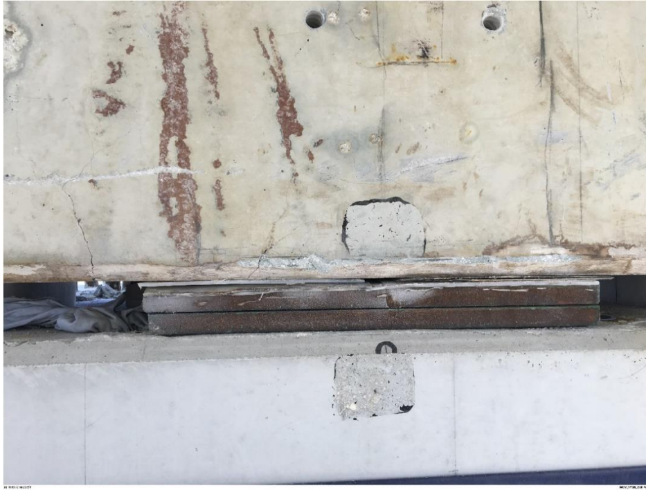
Bridge Factors Photo 87 – View of cracks on south face of Diaphragm II above shim plates on 3/13/18 at 4:32:54 p.m. (Source: Munilla Construction Management, MCM)
