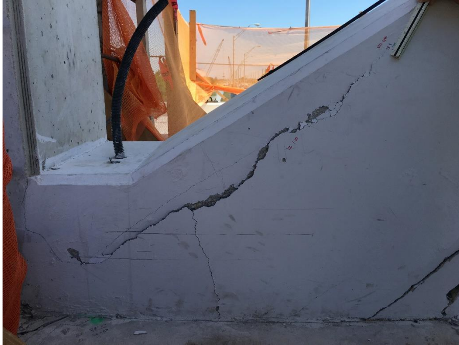
Bridge Factors Photo 94 – View of cracks being monitored at the bottom of diagonal support #11 on west side looking to the east on 3/14/18 at 1:47 p.m. (Source: Bolton – Perez and Associates, BPA)
