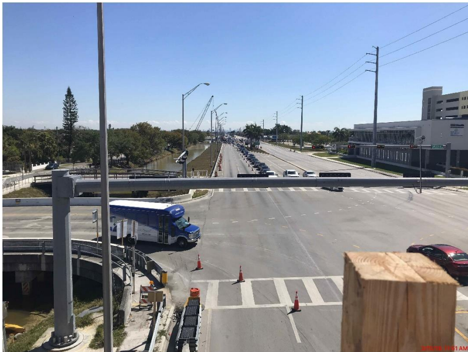
Bridge Factors Photo 105 – View of two of the three westbound lanes closed looking to the east to allow for a crane to be used during the restressing of diagonal support #11 on 3/15/18 at 11:51 a.m. (Source: Munilla Construction Management, MCM)
