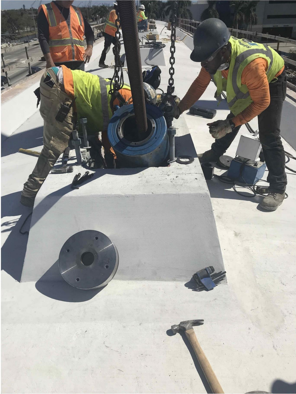
Bridge Factors Photo 32 – View of stressing post tensioning bars in diagonal supports on top of canopy on 2/16/18 at 12:00:28 p.m. (Source: Munilla Construction Management, MCM)
