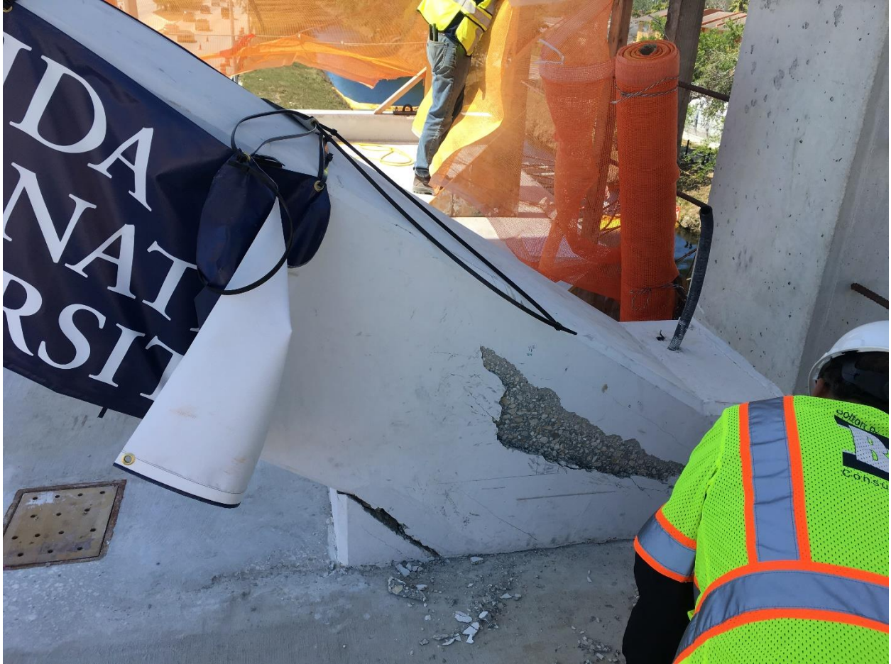
Bridge Factors Photo 90 – View of cracks and delamination at the bottom of diagonal support #11 on east side looking to the west on 3/14/18 at 1:42 p.m. (Source: Bolton – Perez and Associates, BPA)
