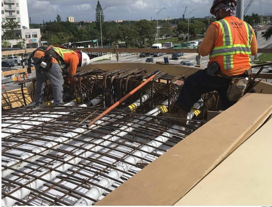
Bridge Factors Photo 23 – View of longitudinal tendons in canopy encased in white plastic duct and canopy end region including reinforcing and conduits before concrete placement on 11/30/17 at 11:14:35 a.m. (Source: Munilla Construction Management, MCM)
