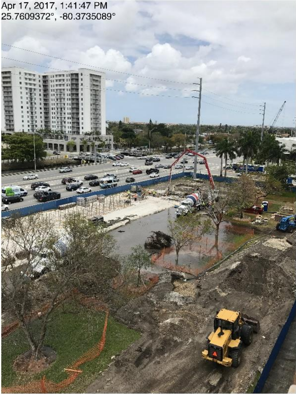
Bridge Factors Photo 2 – View of falsework being set up in adjacent casting yard for construction of main span on 4/17/17 at 1:41:47 p.m. Concrete footings being poured in background at south end (Source: Munilla Construction Management, MCM)
