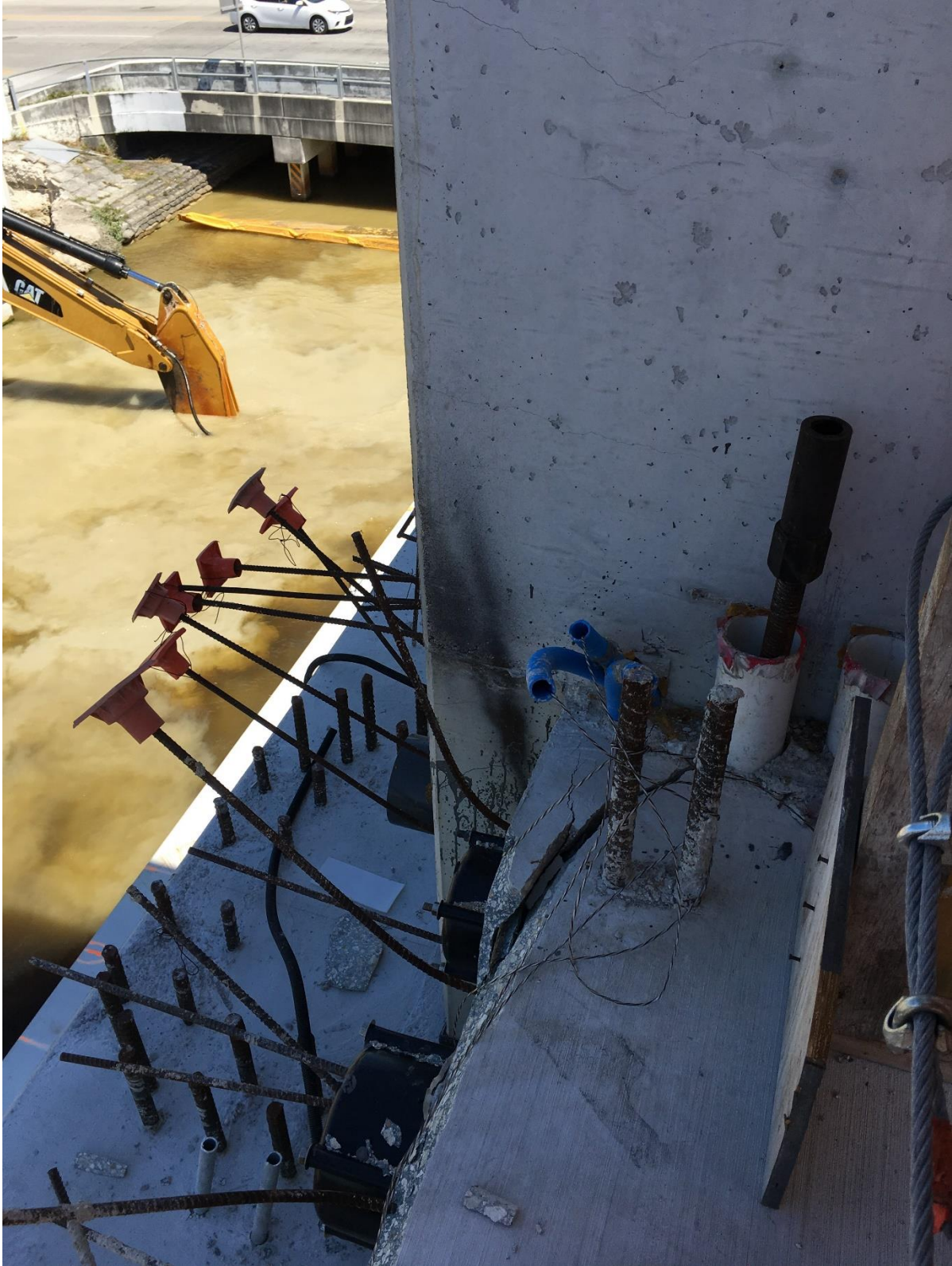
Bridge Factors Photo 98 – Top view of cracks along west side of Diaphragm II on 3/14/18 at 1:51 p.m. (Source: Bolton – Perez and Associates, BPA)
