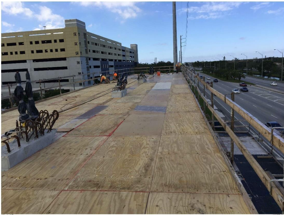
Bridge Factors Photo 19 – View of forms being set looking on top of canopy on 11/16/17 at 11:09:55 a.m. (Source: Munilla Construction Management, MCM)
