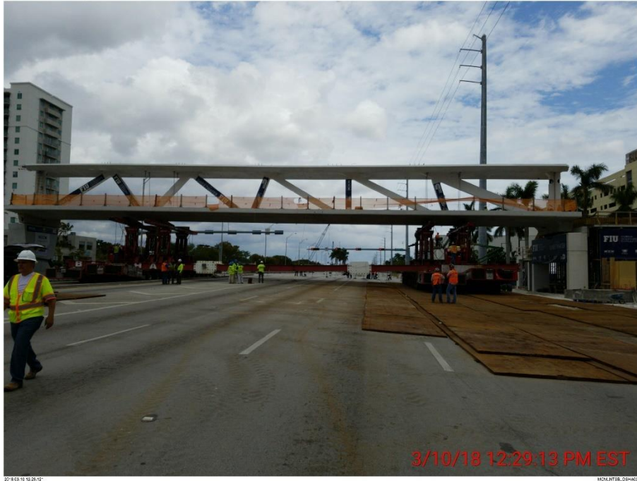
Bridge Factors Photo 60 – View of main span on permanent piers with chains detached from SPMT units on 3/10/18 at 12:29:13 p.m. Actual move complete approximately 12:30 p.m. (Source: Munilla Construction Management, MCM)
