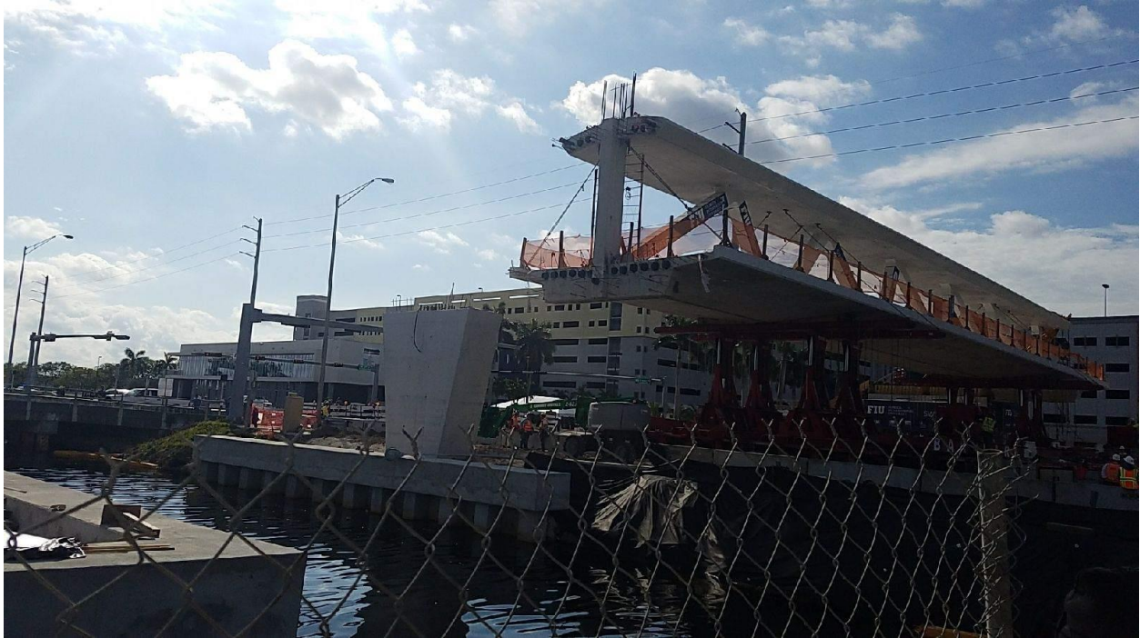
Bridge Factors Photo 56 – View of main span being transported on SPMT units immediately west of permanent piers looking to the southeast toward north face of Diaphragm II on 3/10/18 (Source: Structural Technologies, LLC)
