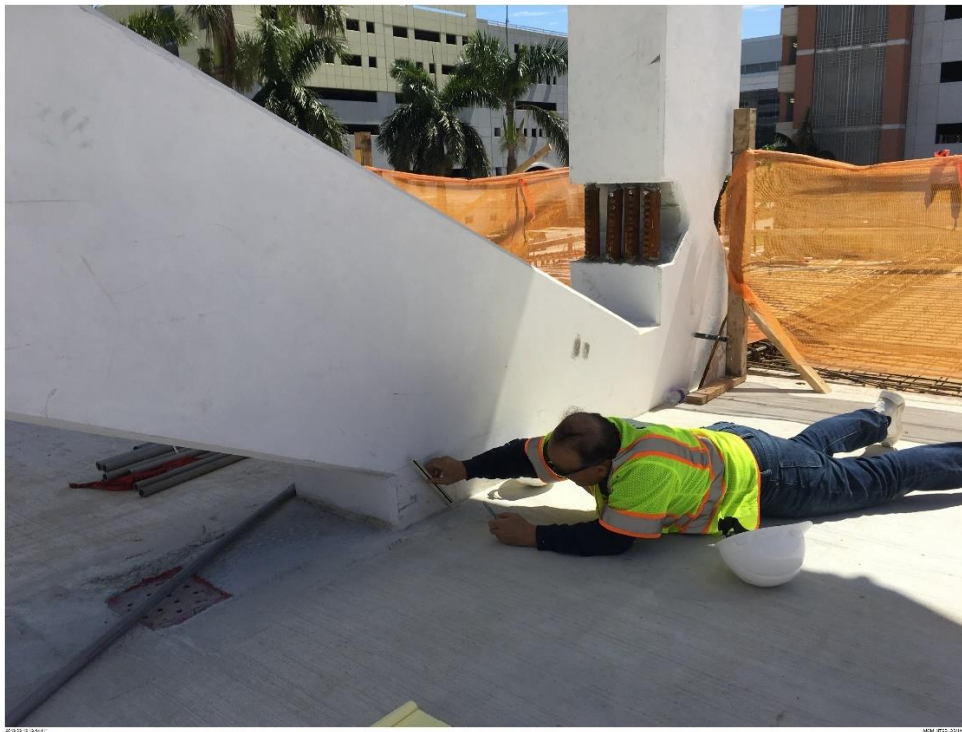
Bridge Factors Photo 85 – View of cracks at the bottom of diagonal support #2 on west side looking to the southeast on 3/13/18 at 1:44:41 p.m. (Source: Munilla Construction Management, MCM)
