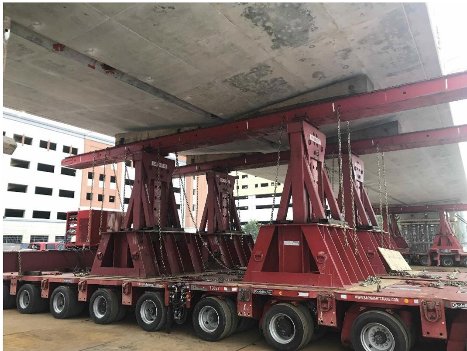
Bridge Factors Photo 50 – View of unattached SPMT with oak crane mats with a taper to match the profile of the bottom flange of the bridge span on 3/9/18 at 7:38:03 a.m. (Source: Munilla Construction Management, MCM)
