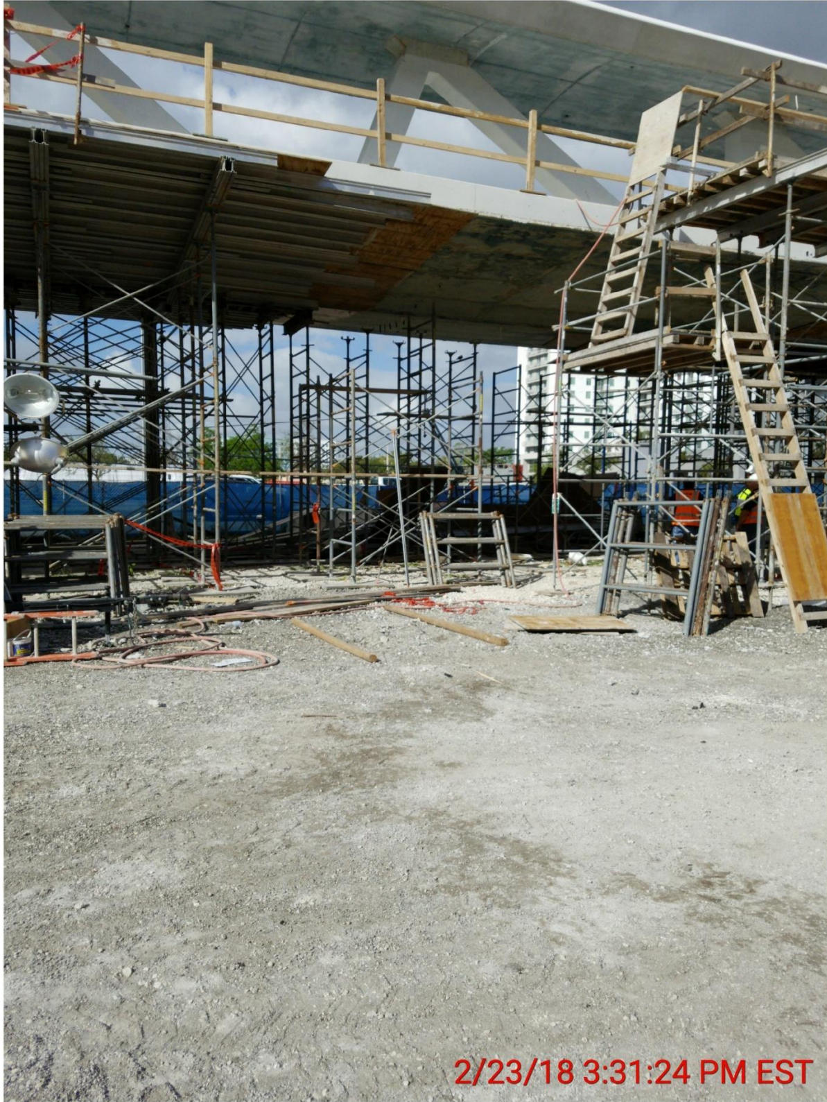
Bridge Factors Photo 35 – View of falsework being removed under deck from middle to outward megashores on 2/23/18 at 3:31:24 p.m. (Source: Munilla Construction Management, MCM)
