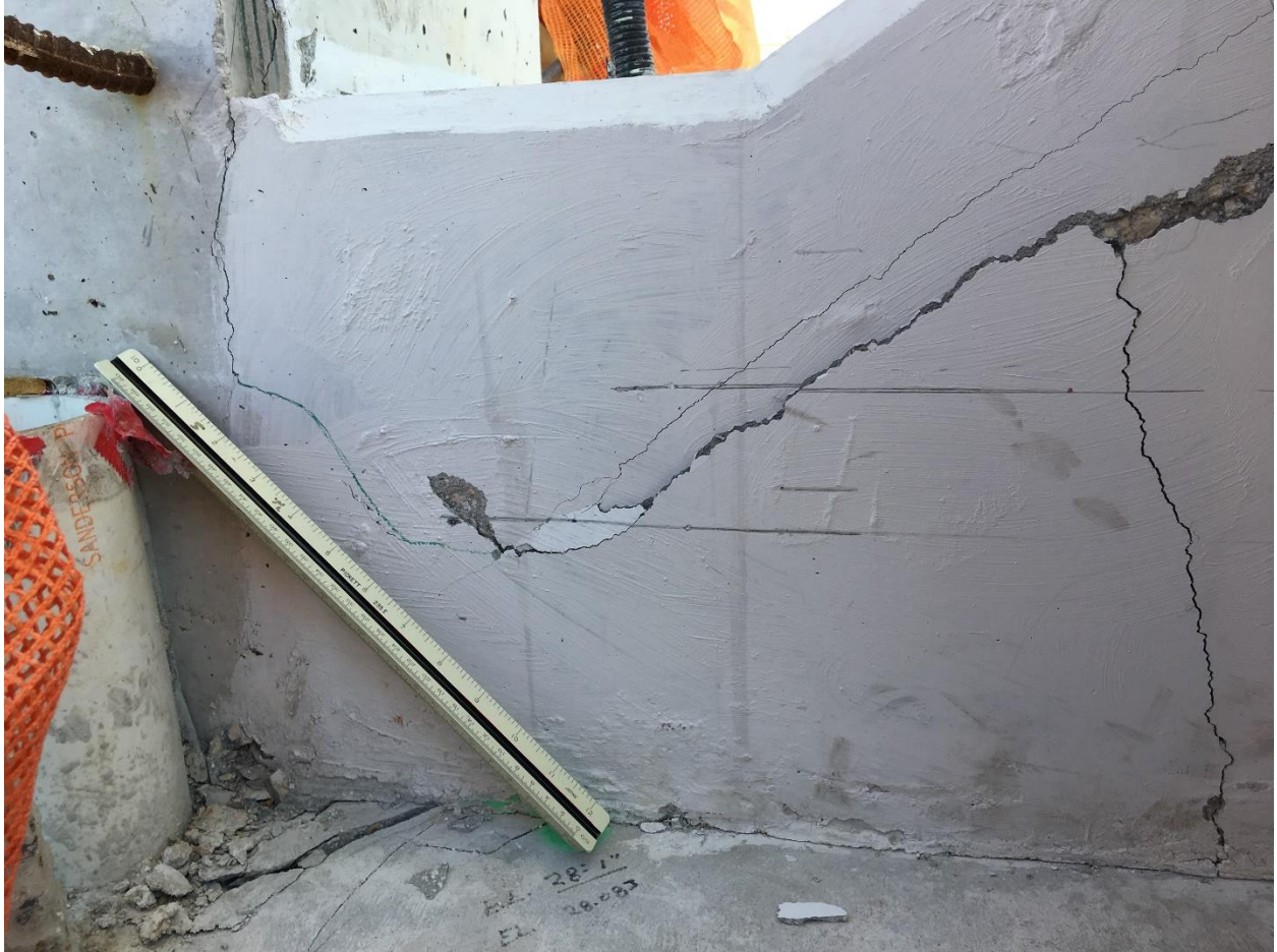
Bridge Factors Photo 92 – View of cracks being monitored at the bottom of diagonal support #11 and vertical support #12 on west side looking to the east on 3/14/18 at 1:45 p.m. (Source: Bolton – Perez and Associates, BPA)
