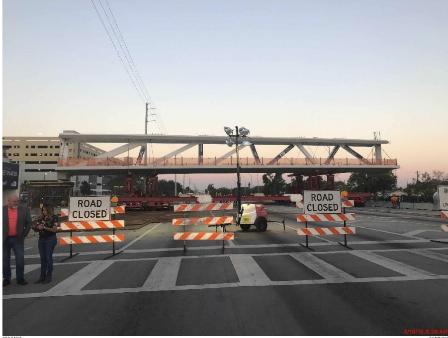
Bridge Factors Photo 54 – View of main span being transported on SPMT units west of permanent piers looking to the west on 3/10/18 at 6:38 a.m. (Source: Munilla Construction Management, MCM)
