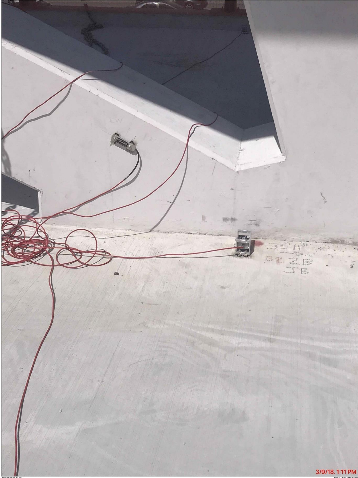
Bridge Factors Photo 51 – View of strain transducer and rotation sensor on main span during move on 3/9/18 at 1:11 p.m. (Source: Munilla Construction Management, MCM)
