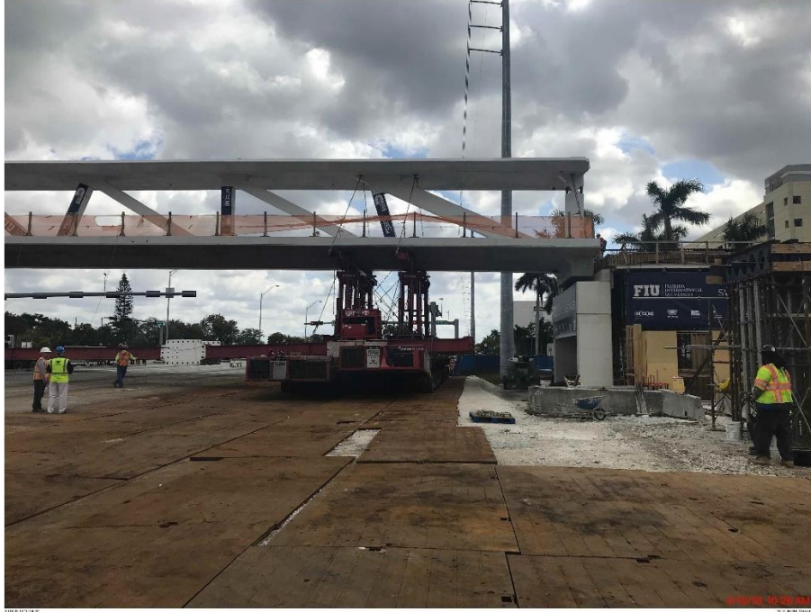
Bridge Factors Photo 58 – View of Diaphragm I, south end of main span, just prior to placement on south pier looking to the east on 3/10/18 at 10:26 a.m. (Source: Munilla Construction Management, MCM)
