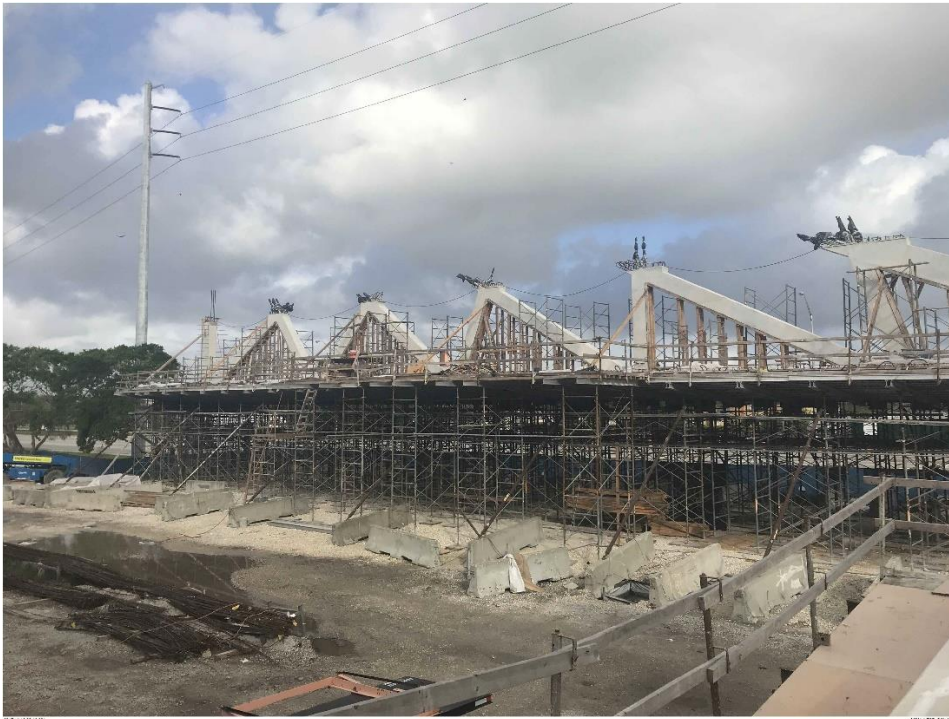
Bridge Factors Photo 17 – View of falsework being set up for construction of canopy on 11/12/17 at 8:41:12 a.m. (Source: Munilla Construction Management, MCM)
