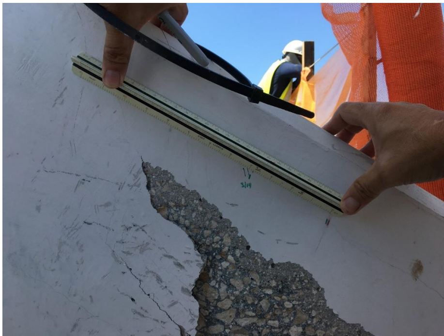
Bridge Factors Photo 88 – View of crack being monitored at the bottom of diagonal support #11 on east side looking to the west on 3/14/18 at 1:42 p.m. (Source: Bolton – Perez and Associates, BPA)
