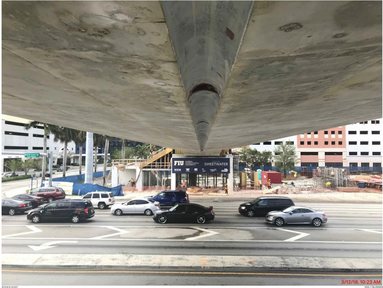
Bridge Factors Photo 72 – View of cut-out for drain pipe under deck looking to the south on 3/12/18 at 10:23 a.m. (Source: Munilla Construction Management, MCM)
