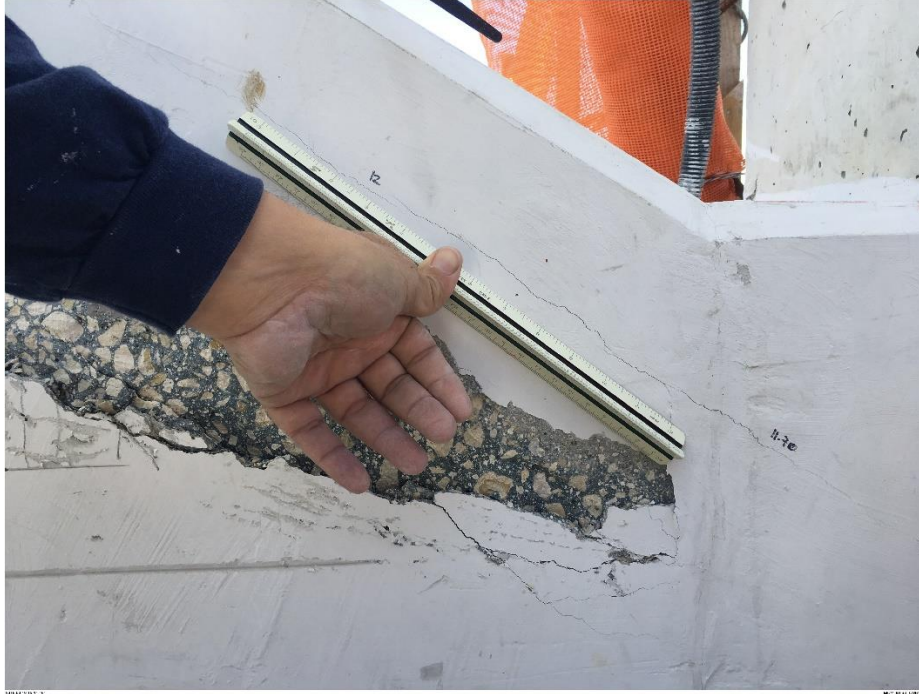
Bridge Factors Photo 82 – View of cracks and delamination at the bottom of diagonal support #11 on east side looking to the west on 3/13/18 at 1:11:16 p.m. (Source: Munilla Construction Management, MCM)
