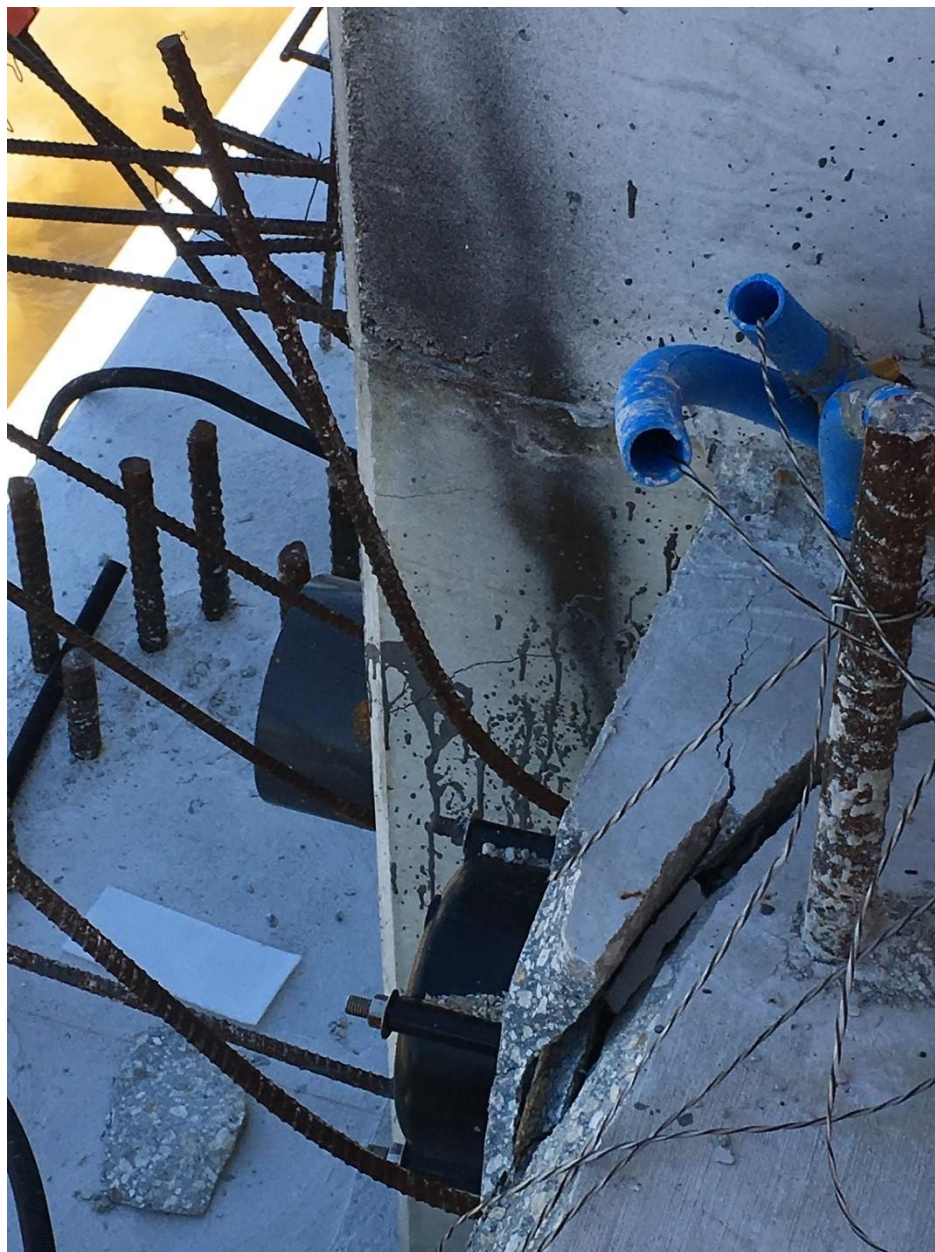
Bridge Factors Photo 99 – Top view of cracks along west side of Diaphragm II on 3/14/18 at 1:51 p.m. (Source: Bolton – Perez and Associates, BPA)
