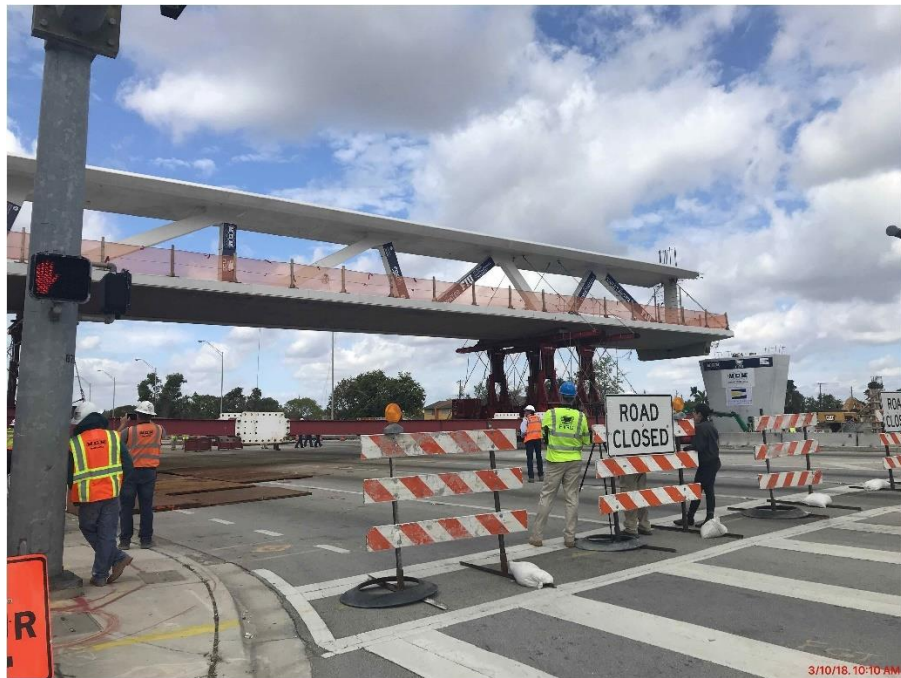
Bridge Factors Photo 55 – View of main span being transported on SPMT units immediately west of permanent piers looking to the northwest on 3/10/18 at 10:10 a.m. (Source: Munilla Construction Management, MCM)
