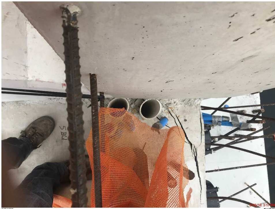
Bridge Factors Photo 65 – Top view of cracks along east side of Diaphragm II on 3/10/18 at 3:17 p.m. (Source: Munilla Construction Management, MCM)
