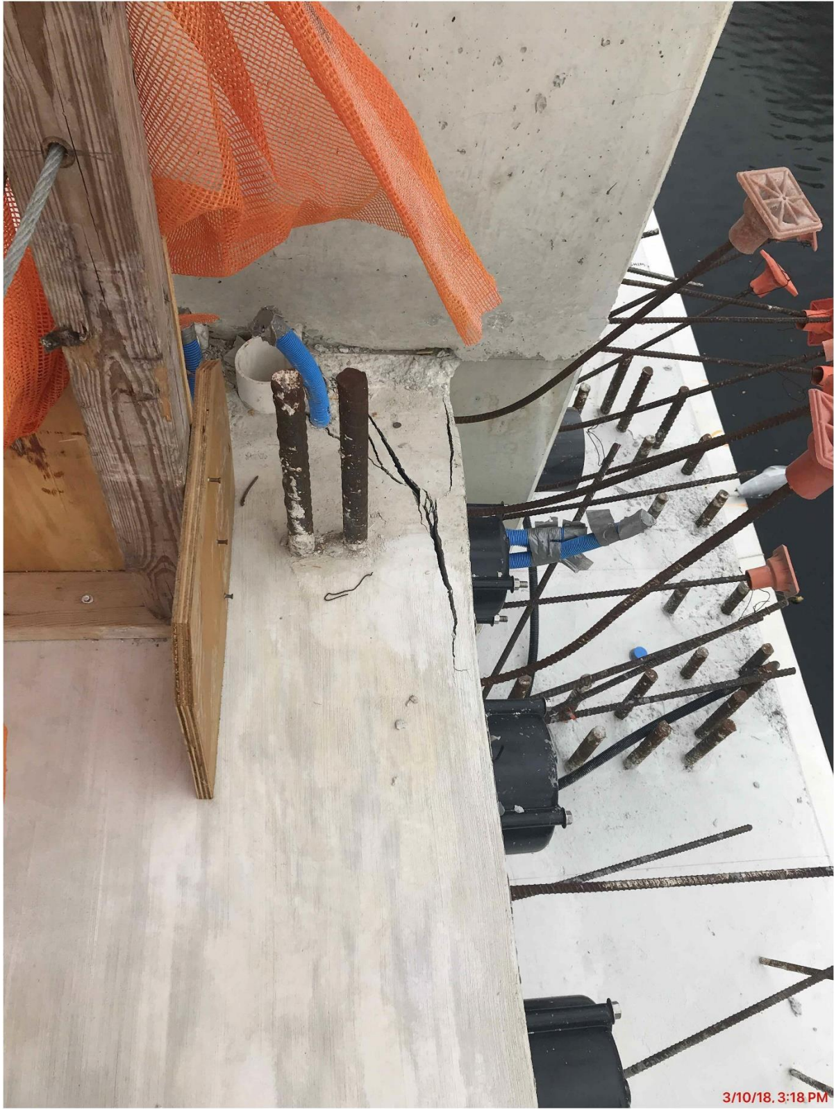
Bridge Factors Photo 66 – Top view of cracks along east side of Diaphragm II on 3/10/18 at 3:18 p.m. (Source: Munilla Construction Management, MCM)
