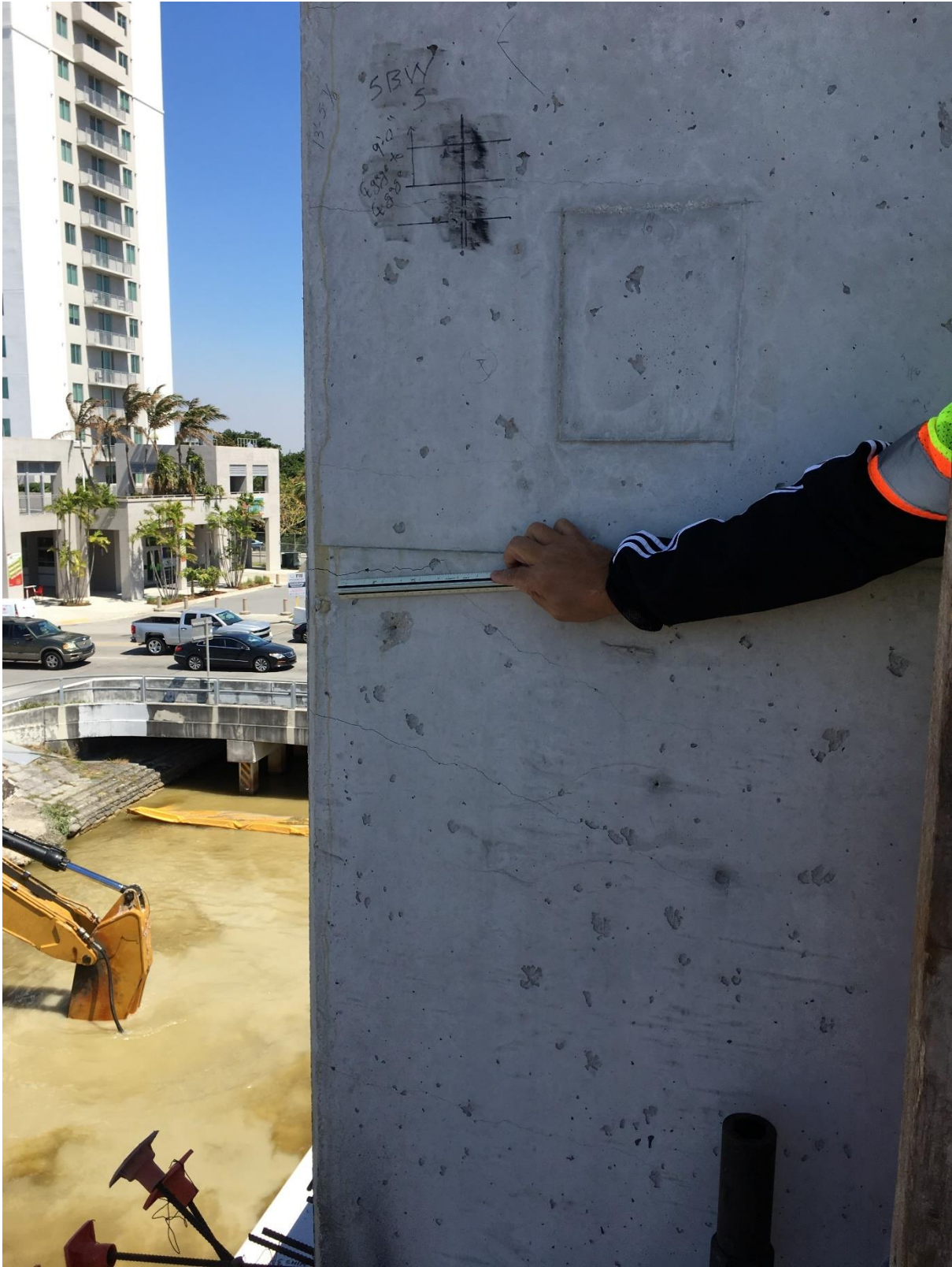
Bridge Factors Photo 100 – View of crack being monitored on the west side of vertical support #12 looking to the east on 3/14/18 at 1:51 p.m. (Source: Bolton – Perez and Associates, BPA)
