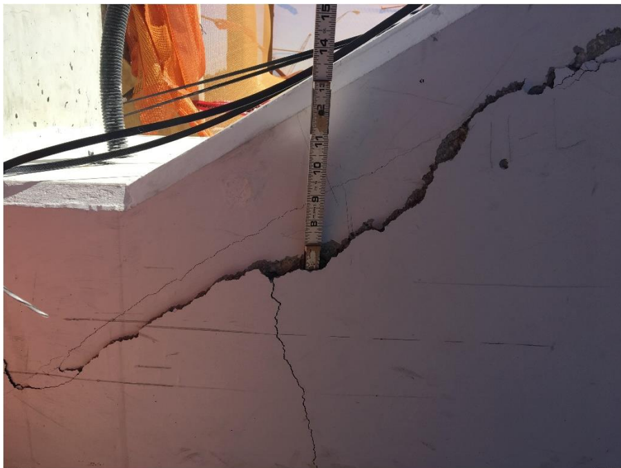
Bridge Factors Photo 77 – View of crack along bottom of diagonal support #11 on west side showing crack is approximately 6 inches deep on 3/13/18 at 11:18:50 a.m. (Source: Munilla Construction Management, MCM)
