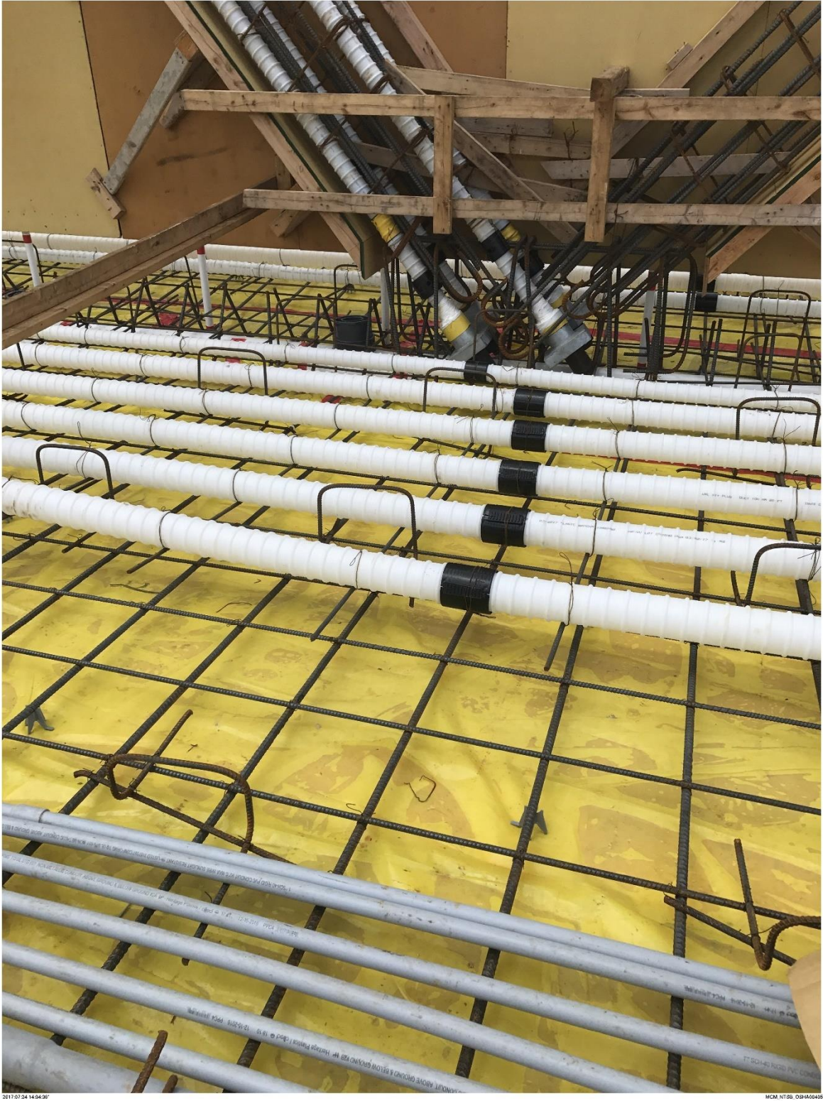
Bridge Factors Photo 7 – View of longitudinal tendons in deck encased in white plastic duct and post tensioning bars in diagonal supports encased in white plastic duct on 7/24/17 at 2:04:38 p.m. (Source: Munilla Construction Management, MCM)
