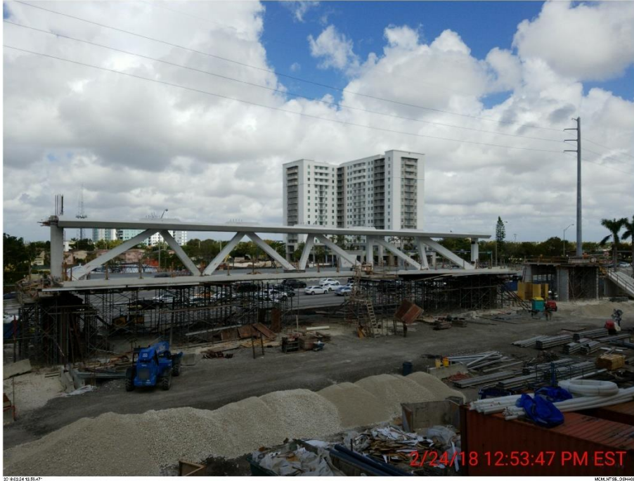
Bridge Factors Photo 40 – View of continued falsework removal under deck from middle to outward mega shores on 2/24/18 at 12:53:47 p.m. (Source: Munilla Construction Management, MCM)
