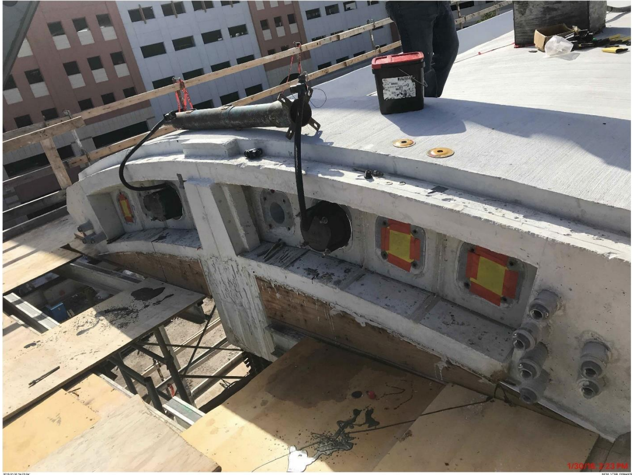
Bridge Factors Photo 29 – View of stressing canopy longitudinal tendons C2 completed on 1/30/18 at 2:23 p.m. (Source: Munilla Construction Management, MCM)
