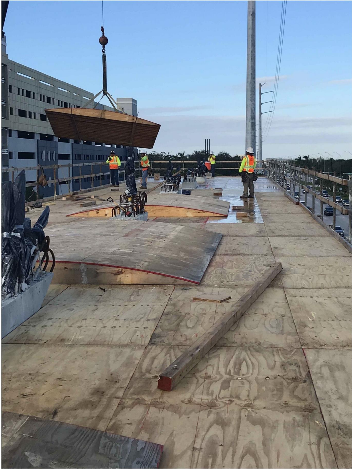
Bridge Factors Photo 20 – View of humped forms being set on top of canopy on 11/17/17 at 8:19:40 a.m. (Source: Munilla Construction Management, MCM)
