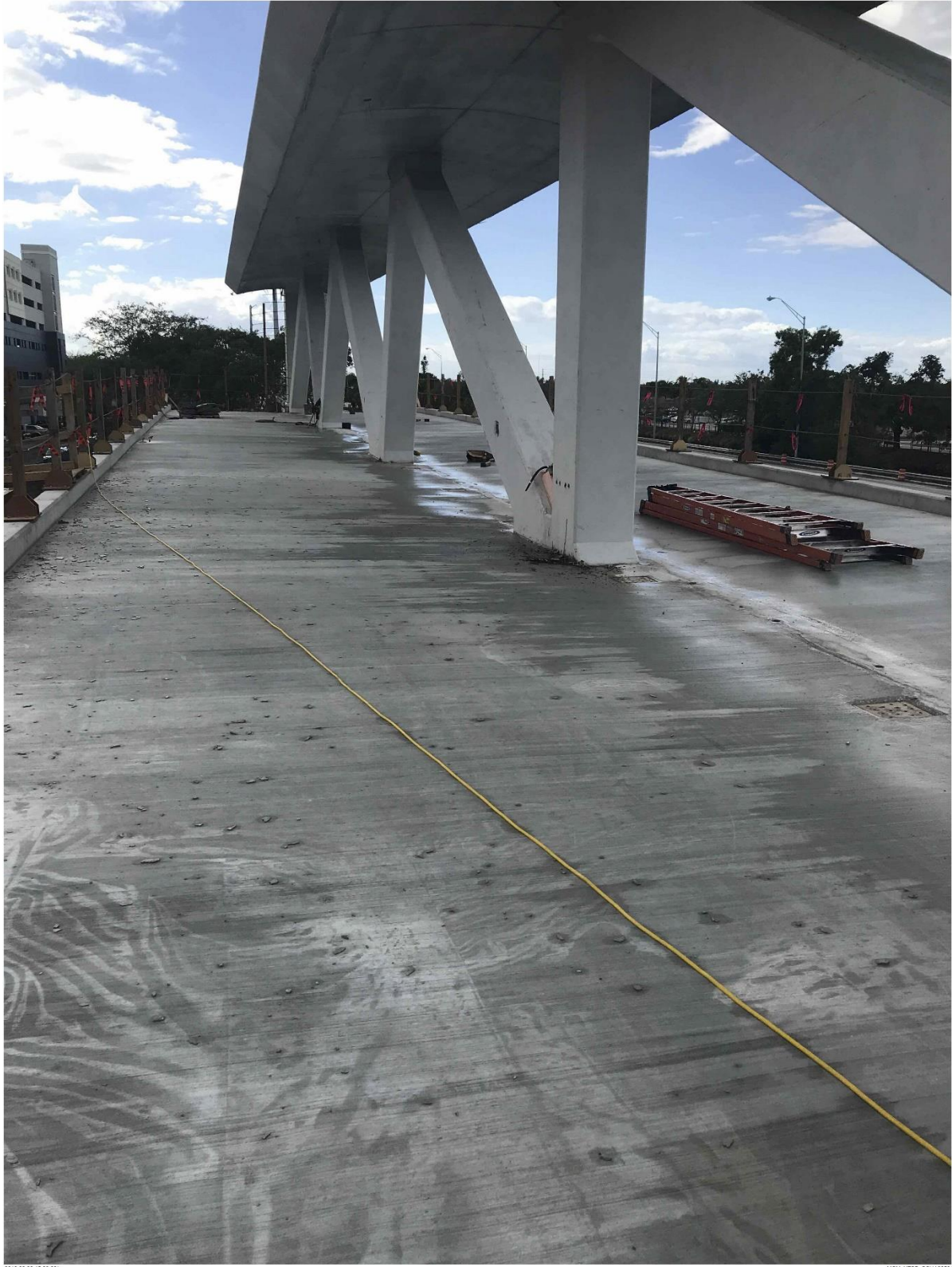
Bridge Factors Photo 46 – View of finished walkway of main span on 2/26/18 at 3:23:29 p.m. (Source: Munilla Construction Management, MCM)
