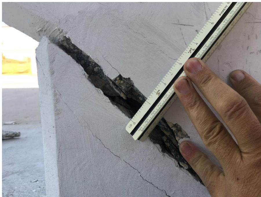
Bridge Factors Photo 81 – View of crack at the bottom of diagonal support #11 on east side looking to the west showing crack is 1 inch wide at one location on 3/13/18 at 1:02:14 p.m. (Source: Munilla Construction Management, MCM)
