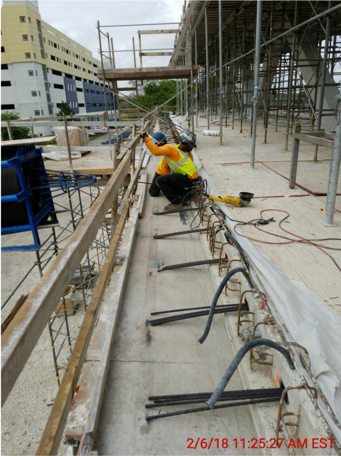
Bridge Factors Photo 31 – View of stressing deck transverse tendons on 2/6/18 at 11:25:27 a.m. (Source: Munilla Construction Management, MCM)
