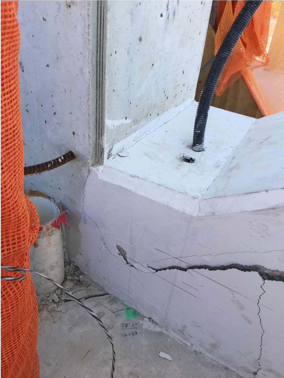
Bridge Factors Photo 93 – View of cracks at the bottom of diagonal support #11 and vertical support #12 on west side looking to the east on 3/14/18 at 1:46 p.m. (Source: Bolton – Perez and Associates, BPA)
