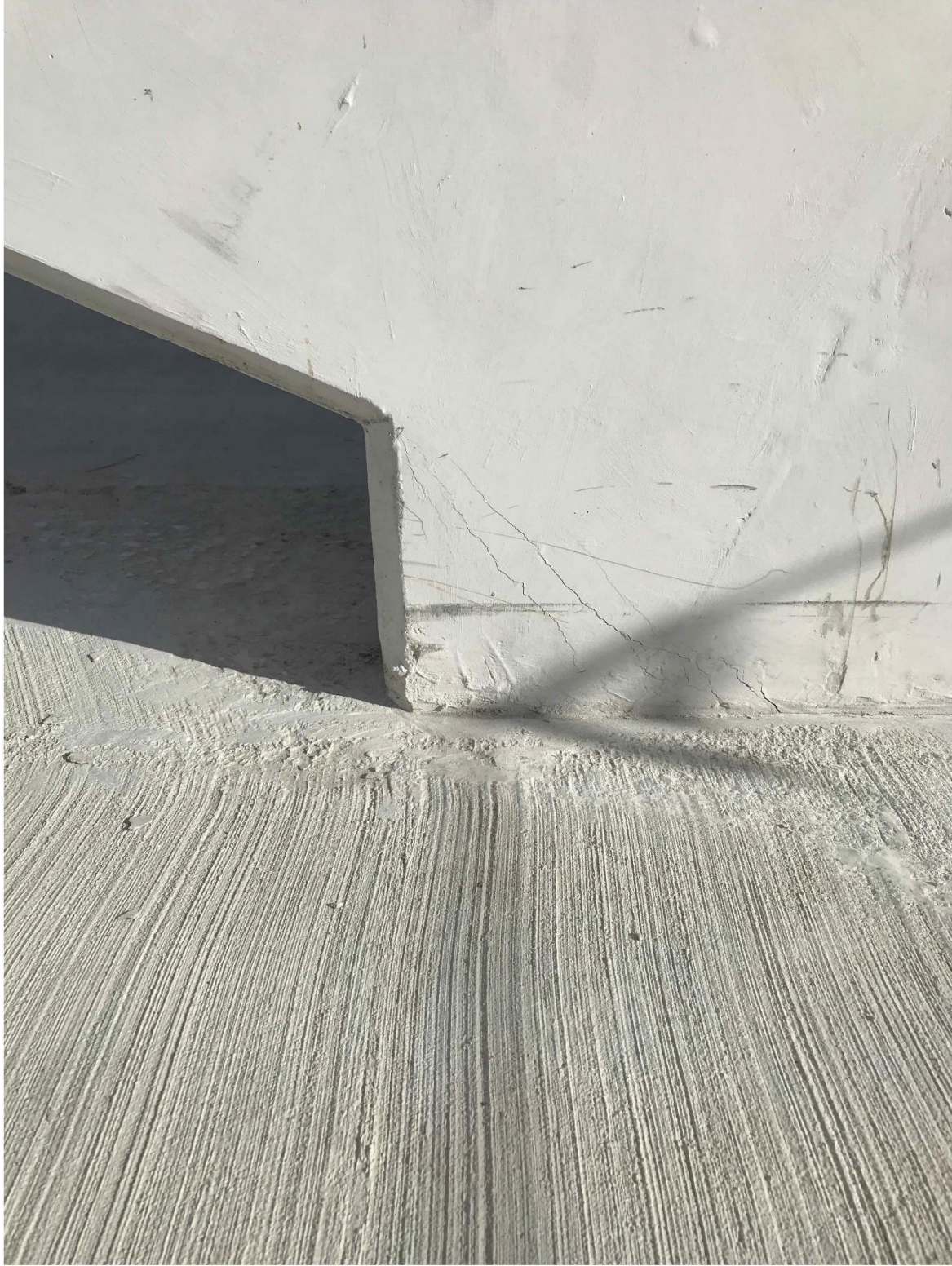
Bridge Factors Photo 44 – View of cracks at the bottom of diagonal support #2 on south side looking to the north in casting yard on 2/26/18 at 8:39:52 a.m. (Source: Munilla Construction Management, MCM)
