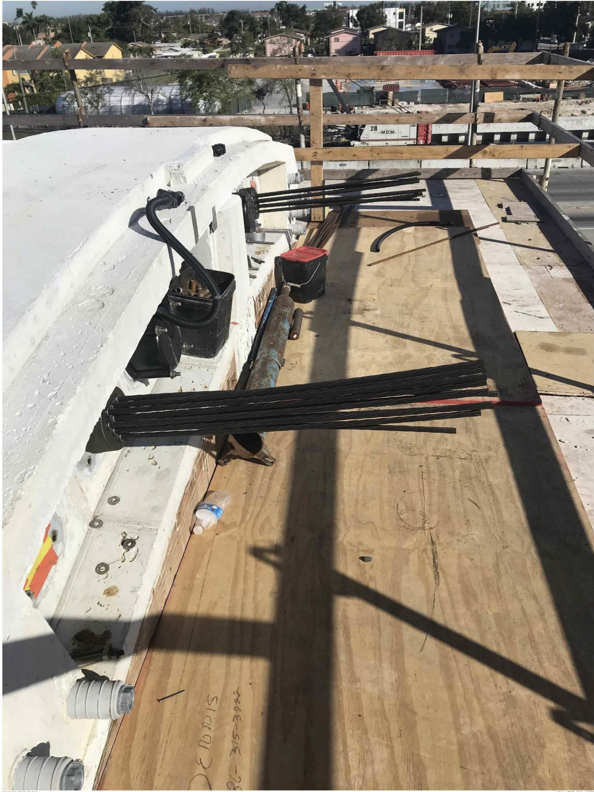
Bridge Factors Photo 33 – View of stressing canopy longitudinal tendon C3 on 2/17/18 at 9:09:21 a.m. (Source: Munilla Construction Management, MCM)
