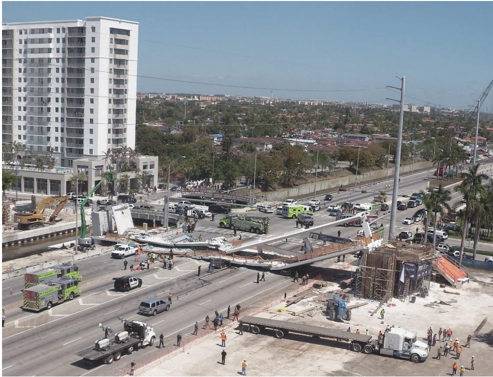
Bridge Factors Photo 107 – View of collapsed pedestrian bridge looking to the northeast (Source: FIU)
