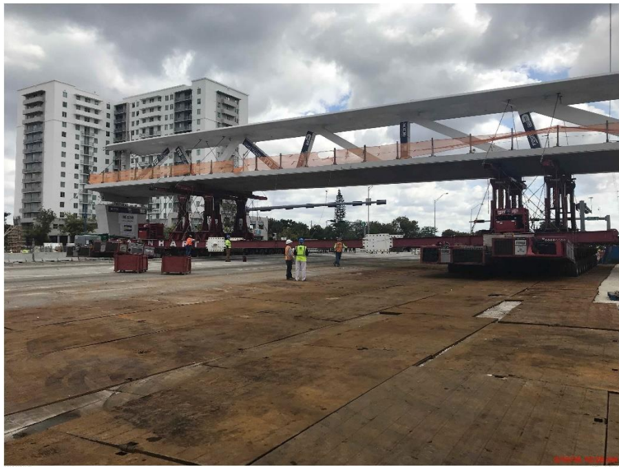
Bridge Factors Photo 59 – View of Diaphragm II, north end of main span, just prior to placement on pylon pier looking to the northeast on 3/10/18 at 10:26 a.m. (Source: Munilla Construction Management, MCM)
