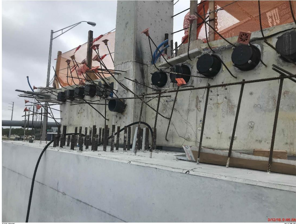
Bridge Factors Photo 67 – View of cracks on north face of Diaphragm II on west side on 3/12/18 at 9:46 a.m. (Source: Munilla Construction Management, MCM)
