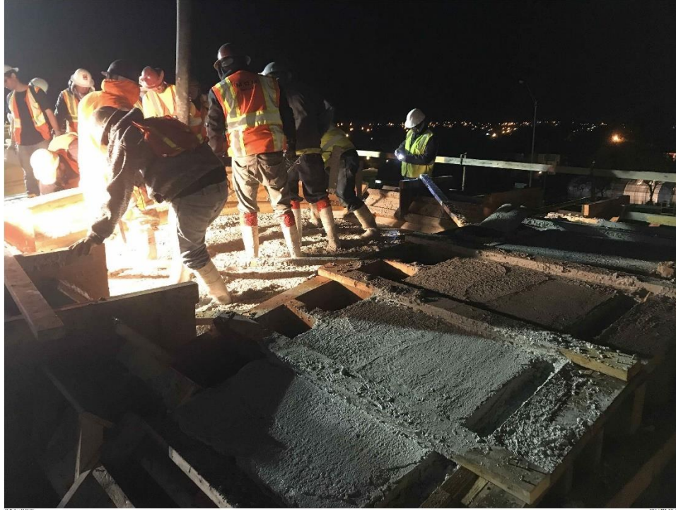
Bridge Factors Photo 25 – View of concrete being poured on top of canopy on 12/14/17 at 2:04:13 a.m. (Source: Munilla Construction Management, MCM)
