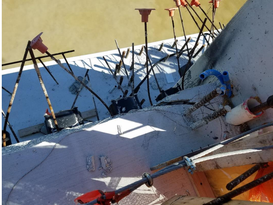
Bridge Factors Photo 104 – Top view of cracks along west side of Diaphragm II on 3/15/18 at 10:55 a.m. (Source: FIU Associate Vice-President of Facilities Management)
