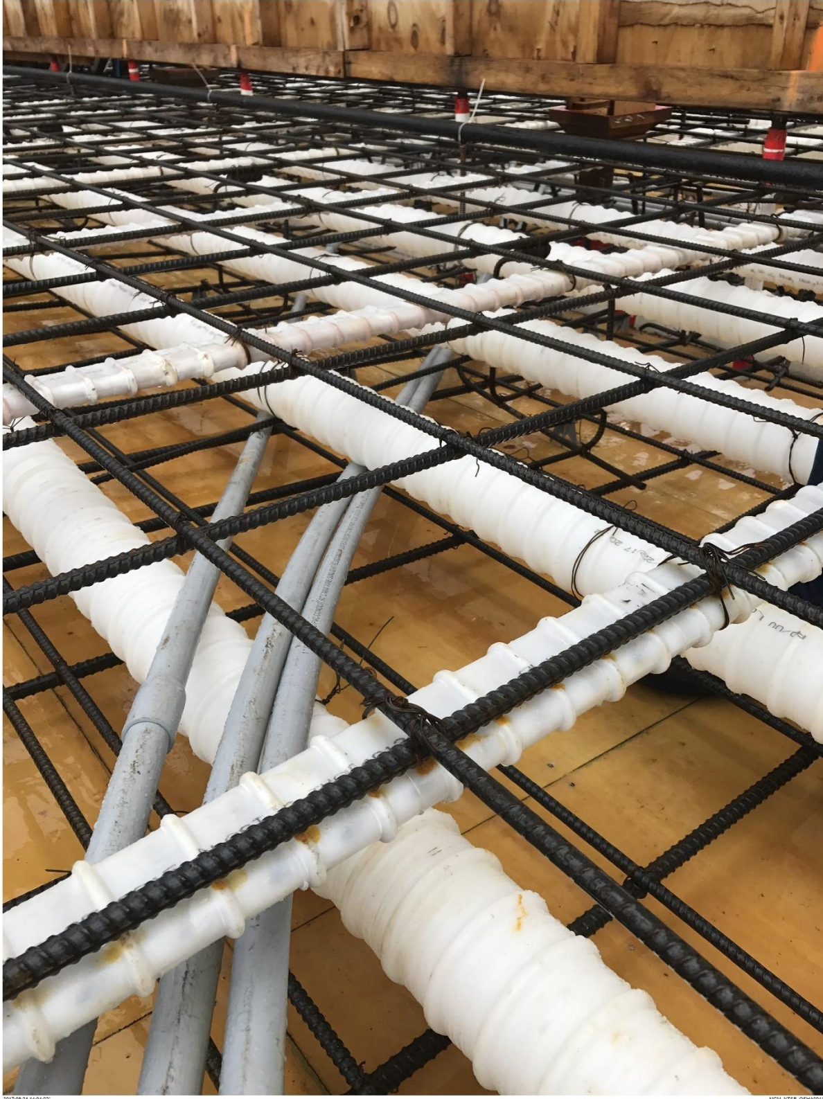
Bridge Factors Photo 10 – View of longitudinal and transverse tendons encased in white plastic duct in deck on 8/24/17 at 2:04:02 p.m. (Source: Munilla Construction Management, MCM)
