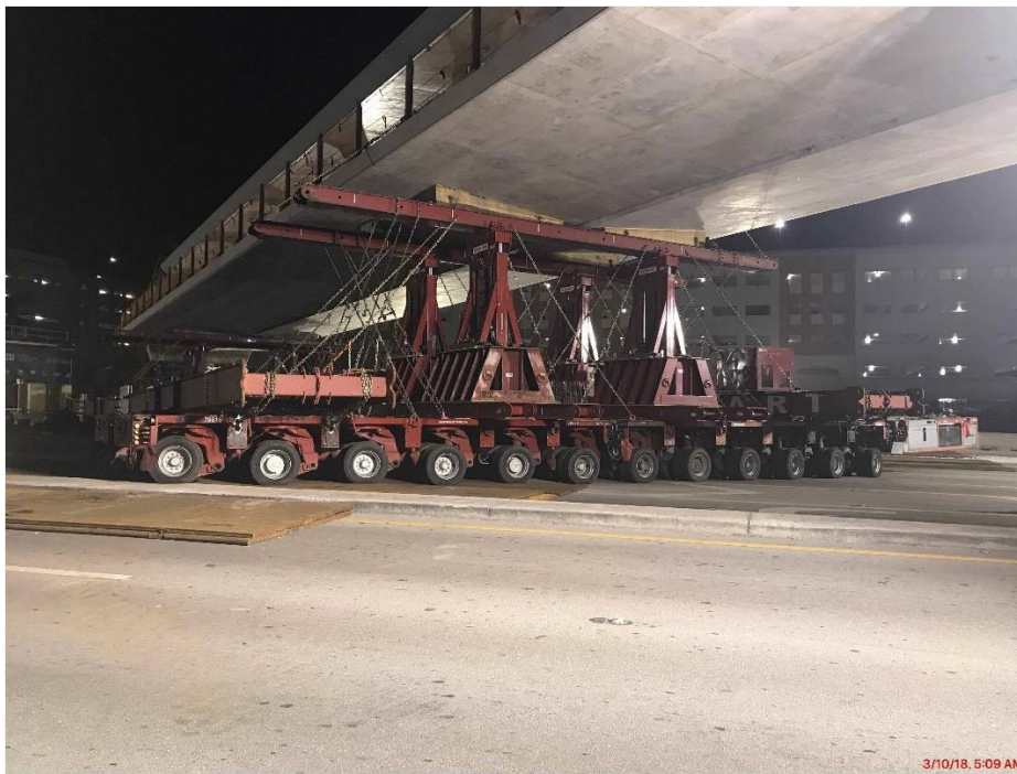
Bridge Factors Photo 53 – View of main span being transported on SPMT units across travel lanes of SW 8 th Street on 3/10/18 at 5:09 a.m. (Source: Munilla Construction Management, MCM)
