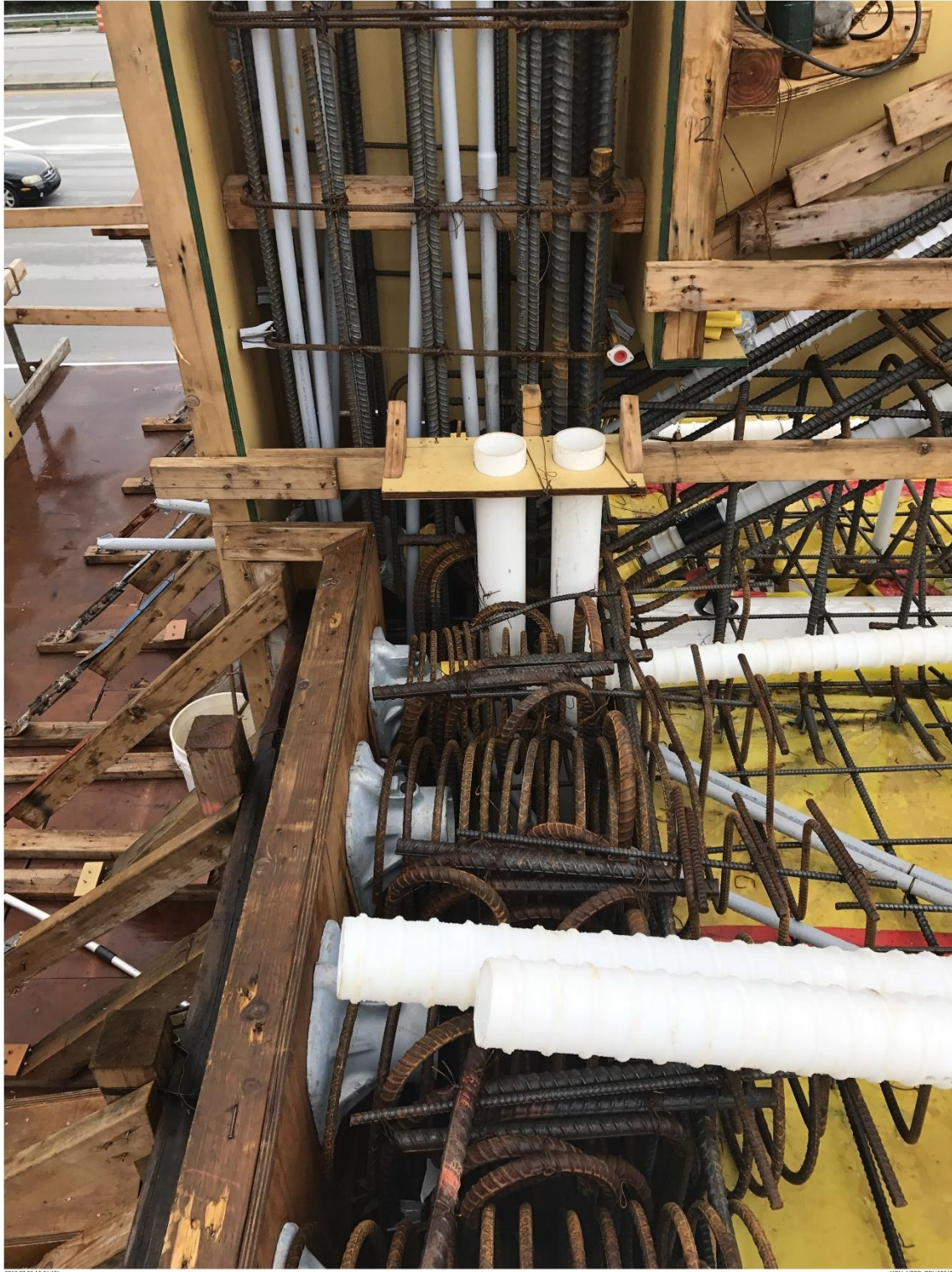
Bridge Factors Photo 8 – View of nodal region including vertical #12 support and diagonal #11 support (background) and deck end region including bridge deck and diaphragm II (foreground) including reinforcing and conduits before concrete placement on 7/25/17 at 5:24:15 p.m. (Source: Munilla Construction Management, MCM)
