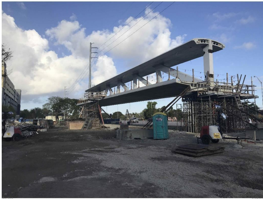
Bridge Factors Photo 41 – View of all falsework removed under deck, only mega shores at each end holding main span on 2/25/18 at 8:01:38 a.m. (Source: Munilla Construction Management, MCM)
