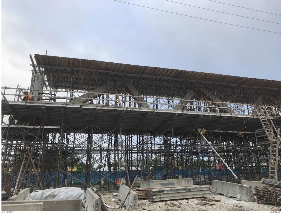
Bridge Factors Photo 18 – View of forms being set for canopy looking from ground level on 11/15/17 at 7:27:11 a.m. (Source: Munilla Construction Management, MCM)
