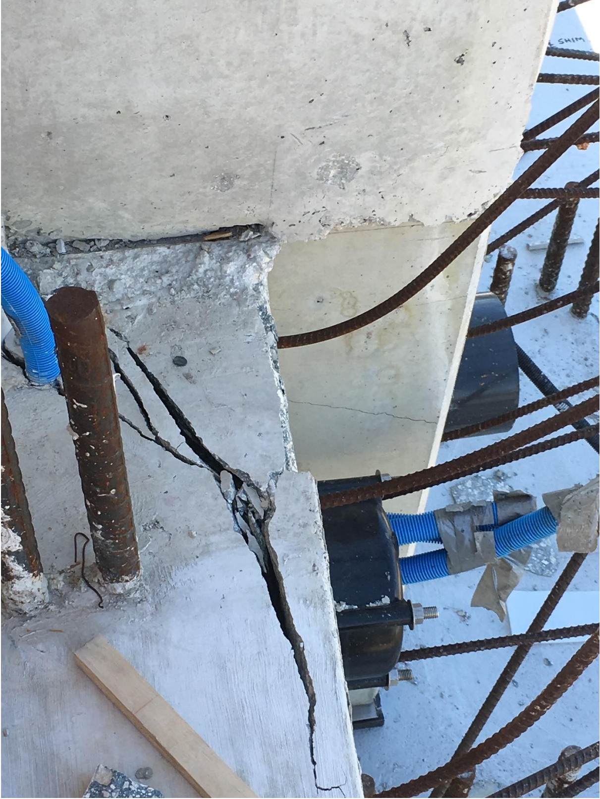
Bridge Factors Photo 97 – Top view of cracks along east side of Diaphragm II on 3/14/18 at 1:50 p.m. (Source: Bolton – Perez and Associates, BPA)
