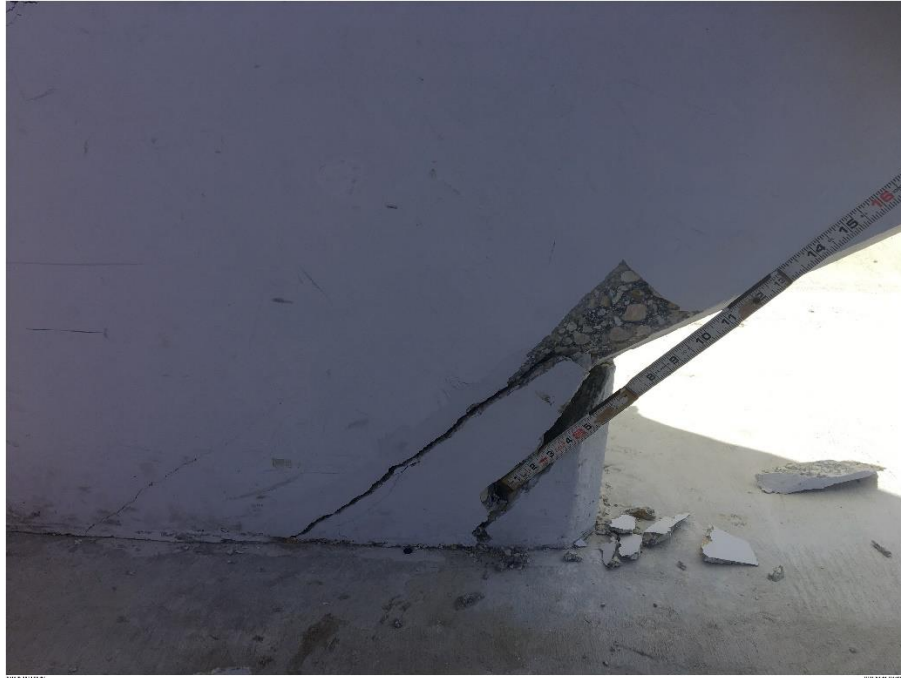
Bridge Factors Photo 80 – View of cracks at the bottom of diagonal support #11 on west side looking to the east showing folding rule inside crack on 3/13/18 at 11:26:36 a.m. (Source: Munilla Construction Management, MCM)
