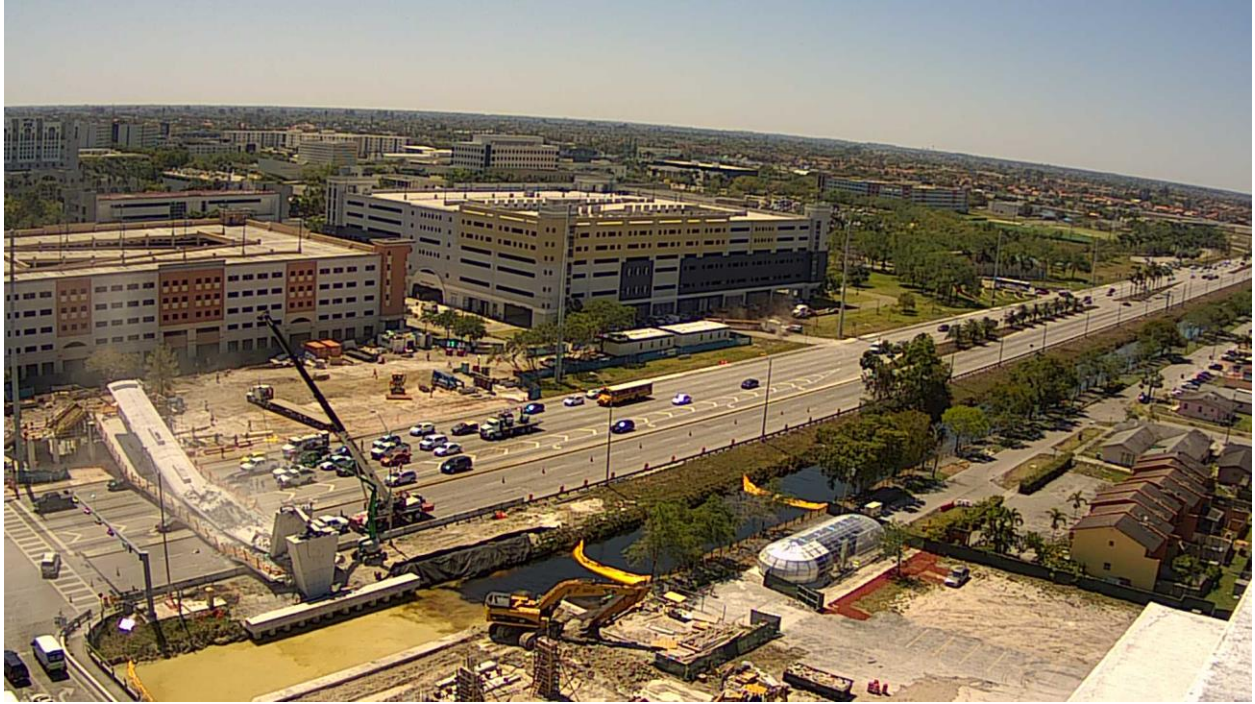
Bridge Factors Photo 106 – View of collapsed pedestrian bridge looking to the southwest on 3/15/18 at approximately 1:47 p.m. (Source: FIU)
