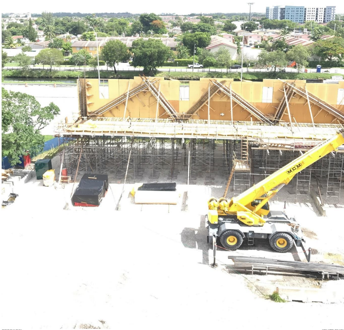
Bridge Factors Photo 9 – View of post tensioning bars and rebar shown in diagonal supports on 8/5/17 at 11:06:51 a.m. (Source: Munilla Construction Management, MCM)
