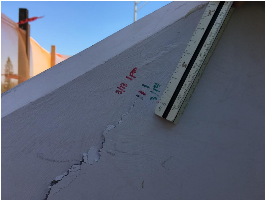
Bridge Factors Photo 95 – View of crack being monitored at the bottom of diagonal support #11 on west side looking to the east on 3/14/18 at 1:47 p.m. (Source: Bolton – Perez and Associates, BPA)
