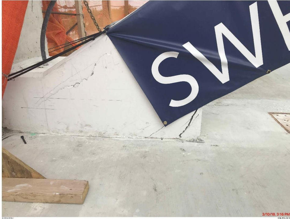
Bridge Factors Photo 62 – View of cracks at the bottom of diagonal support #11 on west side looking to the east on 3/10/18 at 3:16 p.m. (Source: Munilla Construction Management, MCM)
