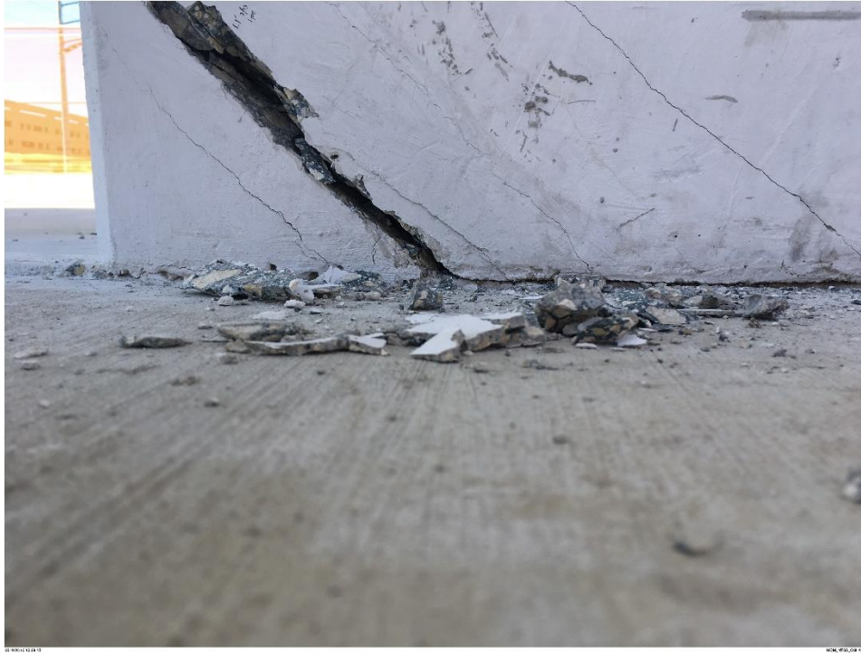
Bridge Factors Photo 84 – View of cracks at the bottom of diagonal support #11 on east side looking to the west on 3/13/18 at 1:29:15 p.m. (Source: Munilla Construction Management, MCM)
