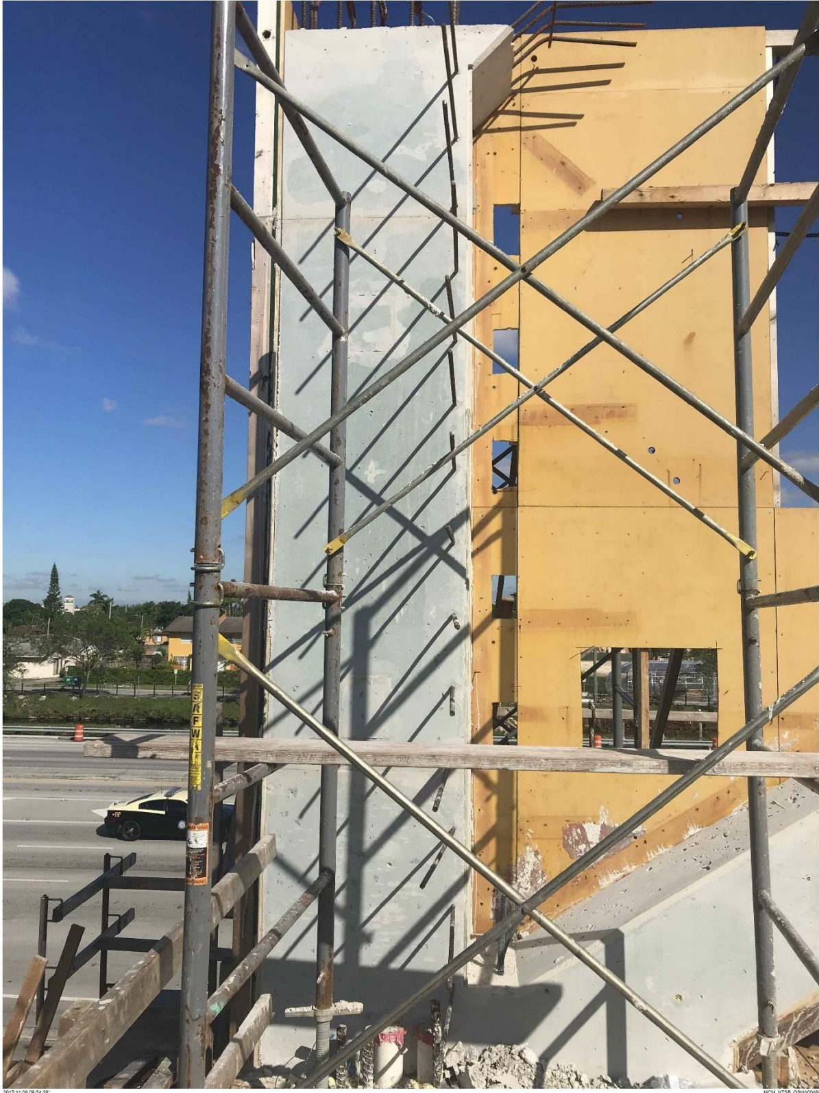
Bridge Factors Photo 15 – View of forms removed from vertical #12 support on 11/8/17 at 9:54:28 a.m. (Source: Munilla Construction Management, MCM)
