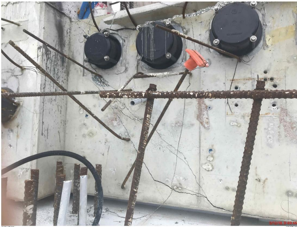
Bridge Factors Photo 68 – View of cracks on north face of Diaphragm II on west side on 3/12/18 at 9:49 a.m. (Source: Munilla Construction Management, MCM)
