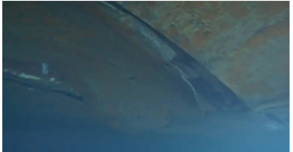
Long crack from aft to fwd (ref 7.), where damage opened the plating.
