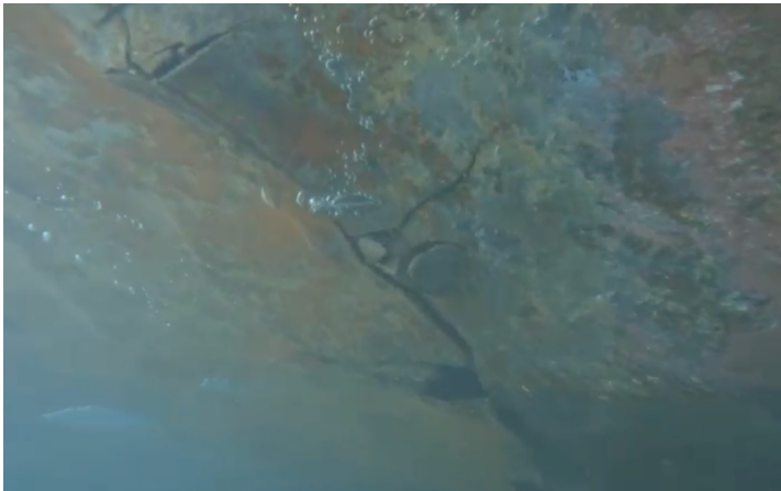
Crack further on SB side (ref 12)
