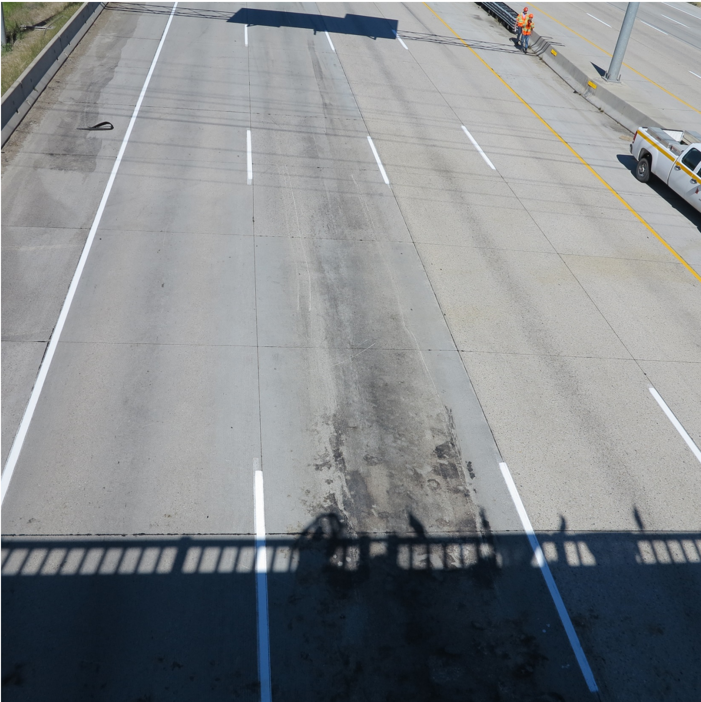
Highway Photo 11 – View of tire marks and pavement scrapes leading to a burned area on the concrete impact lane.
