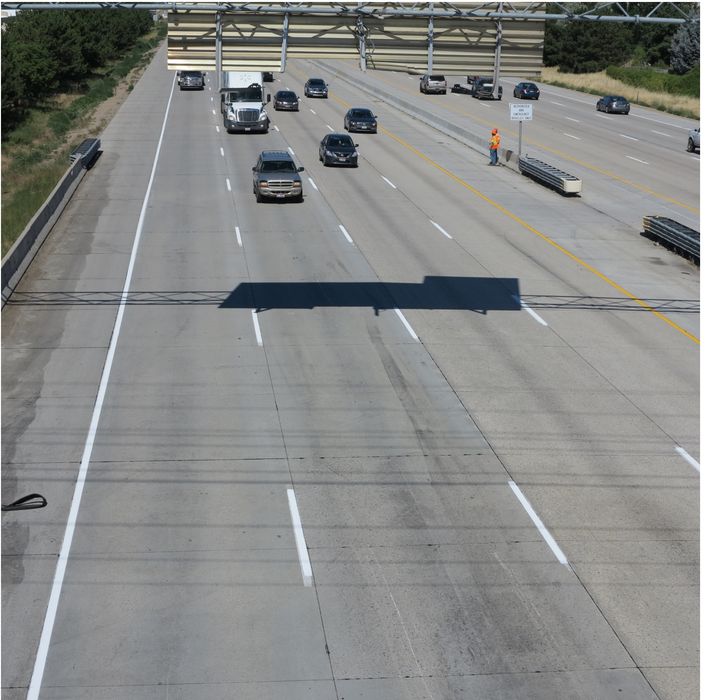
Highway Photo 9 – View of tire friction marks and scrape marks in the number 2 lane. Also note the damage to the bottom of the overhead sign. Photos were taken from the Cloverdale Road overpass.
