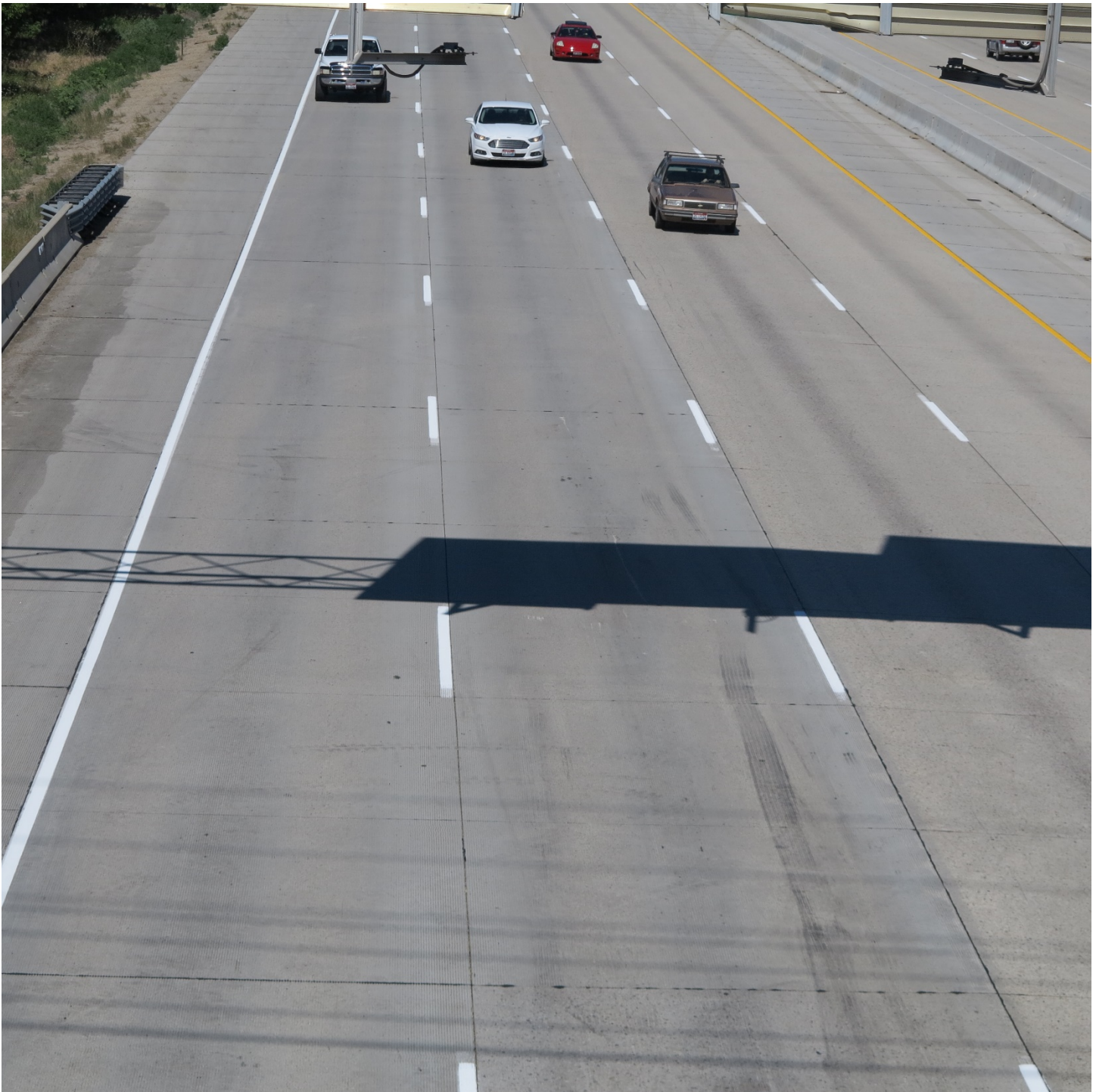
Highway Photo 12 – Additional view looking west in the I-84 eastbound lanes from the Cloverdale overpass. Tire marks and scrapes begin west of the shadow on the pavement formed by the sunlight on the overhead highway sign.
