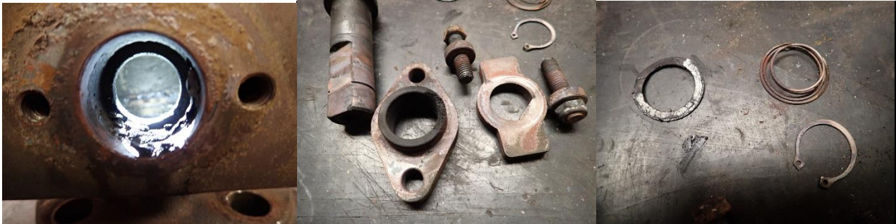
Stem packing has disintegrated.
