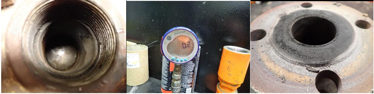
Valve would not hold pressure to test.
