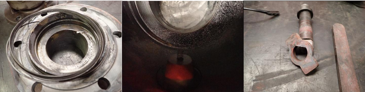
Top and bottom extreme seats only reside remaining. Stem packing disintegrated.
