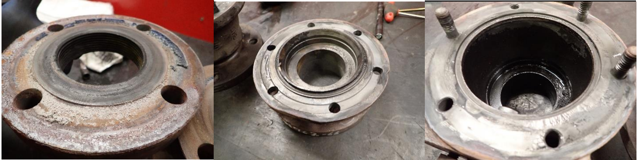
1570E flange gasket disintegrated. Spiral wound body gasket disintegrated.
