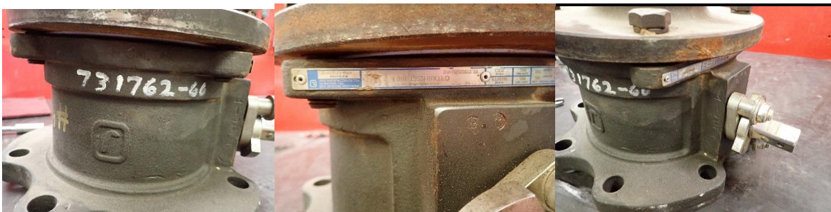
Valve doesn't appear to have direct heat damage
