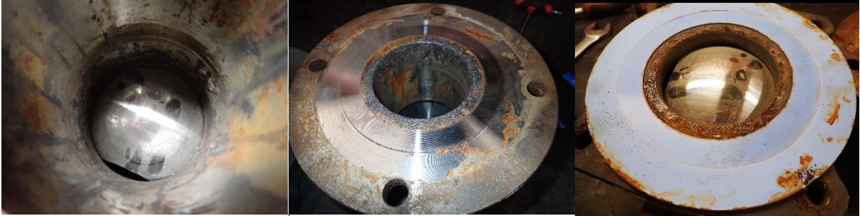
Ball and gasket were in good condition considering.
