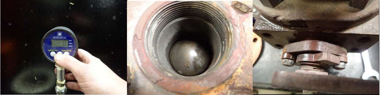
Valve would not hold any pressure or make bubbles due to size of leakage.
