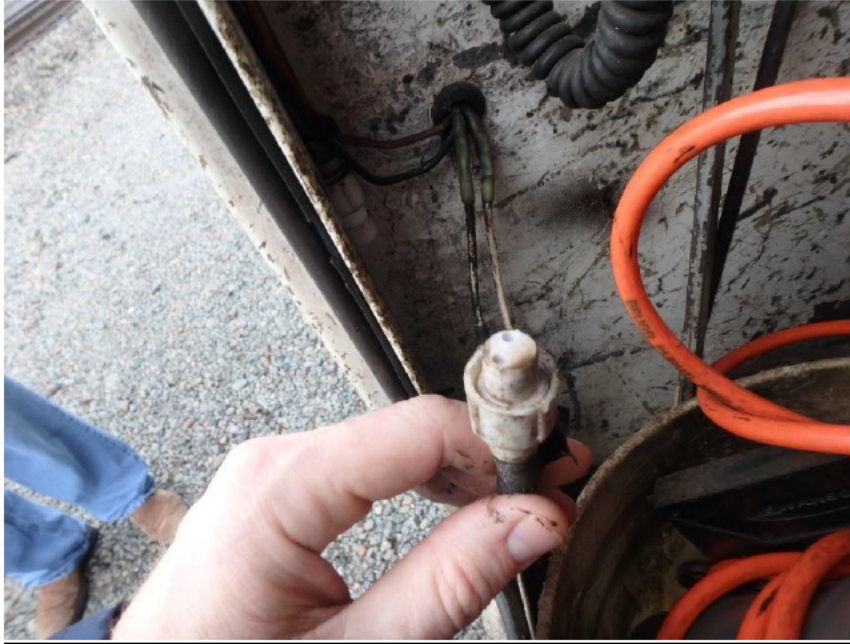
Figure 3. Photo showing disconnected white wire connector that was intended to connect the external mounted speaker to the external radio. The wire was disconnected from the radio and hanging inside the cabinet.
