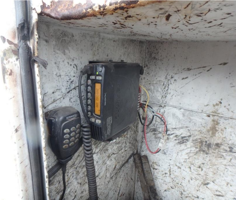
Figure 2. Photo showing the external radio mounted inside of a cabinet on the body of CSXT welding truck No. 240150.
