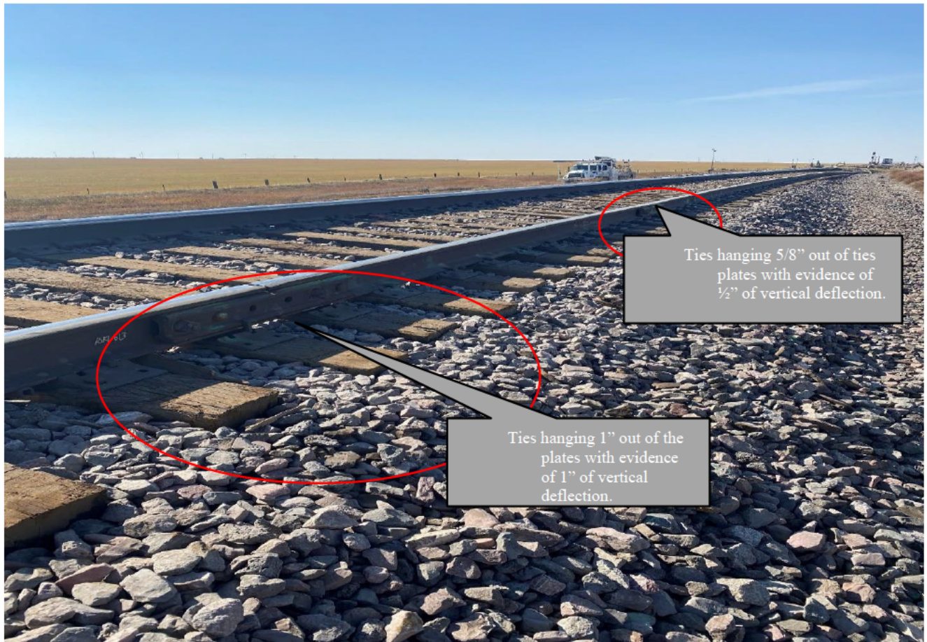
Figure 3 – “As found” by investigators - non-supporting ties under suspended plug rail joint
