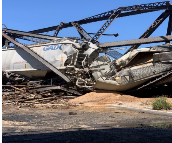
Figure 2- Photo of Rio Salado Park way after bridge collapse (Photo courtesy of SMART-TD)
