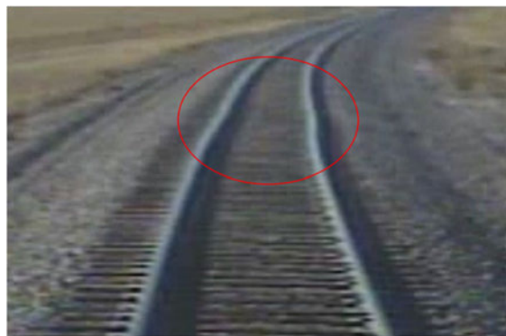
Figure 4 – Still image taken from the outward facing camera footage from the lead locomotive of Amtrak Train No. 7. This image was taken seconds before the train derailed. (Photo courtesy of Amtrak)
