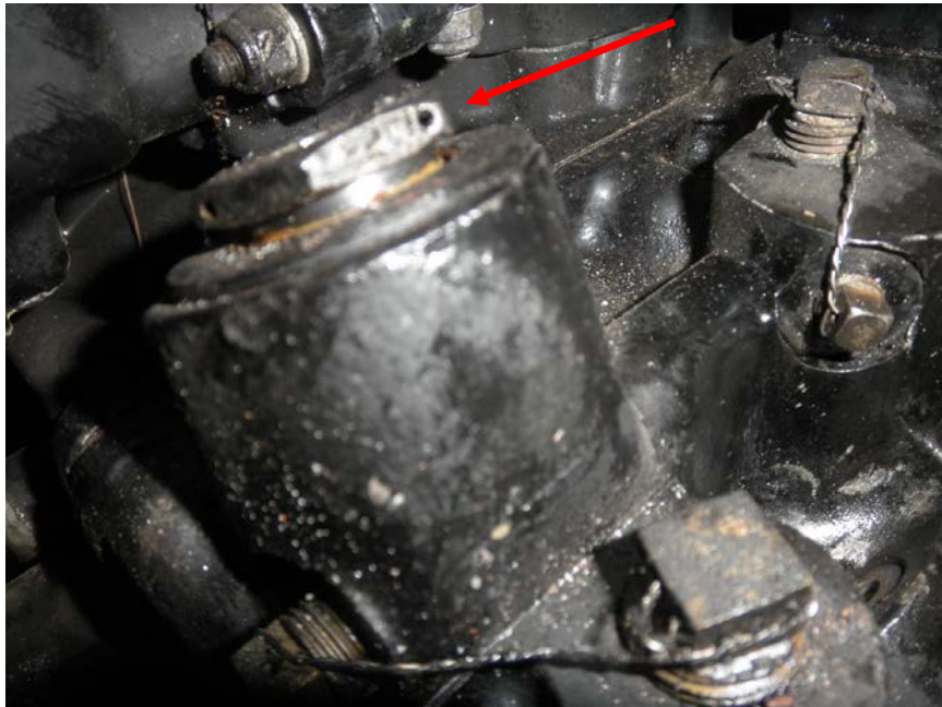
Photo No. 141: Close up of the No. 3 engine's carburetor vent adapter nut showing that it was not safety wired.
