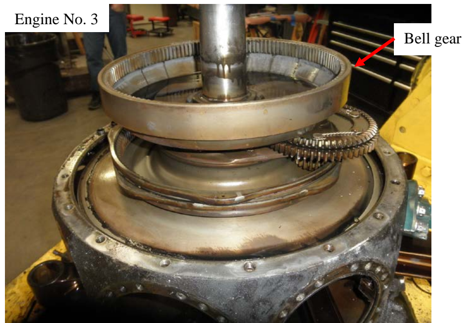
Photo No. 40: View of the bell gear showing that it was intact and had no rotational damage to the gear teeth.
