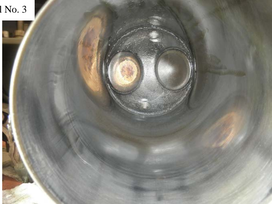
Photo No. 168: View of the inside of the No. 3 cylinder showing no damage to the barrel and the two valves were centered in place in the closed position.
