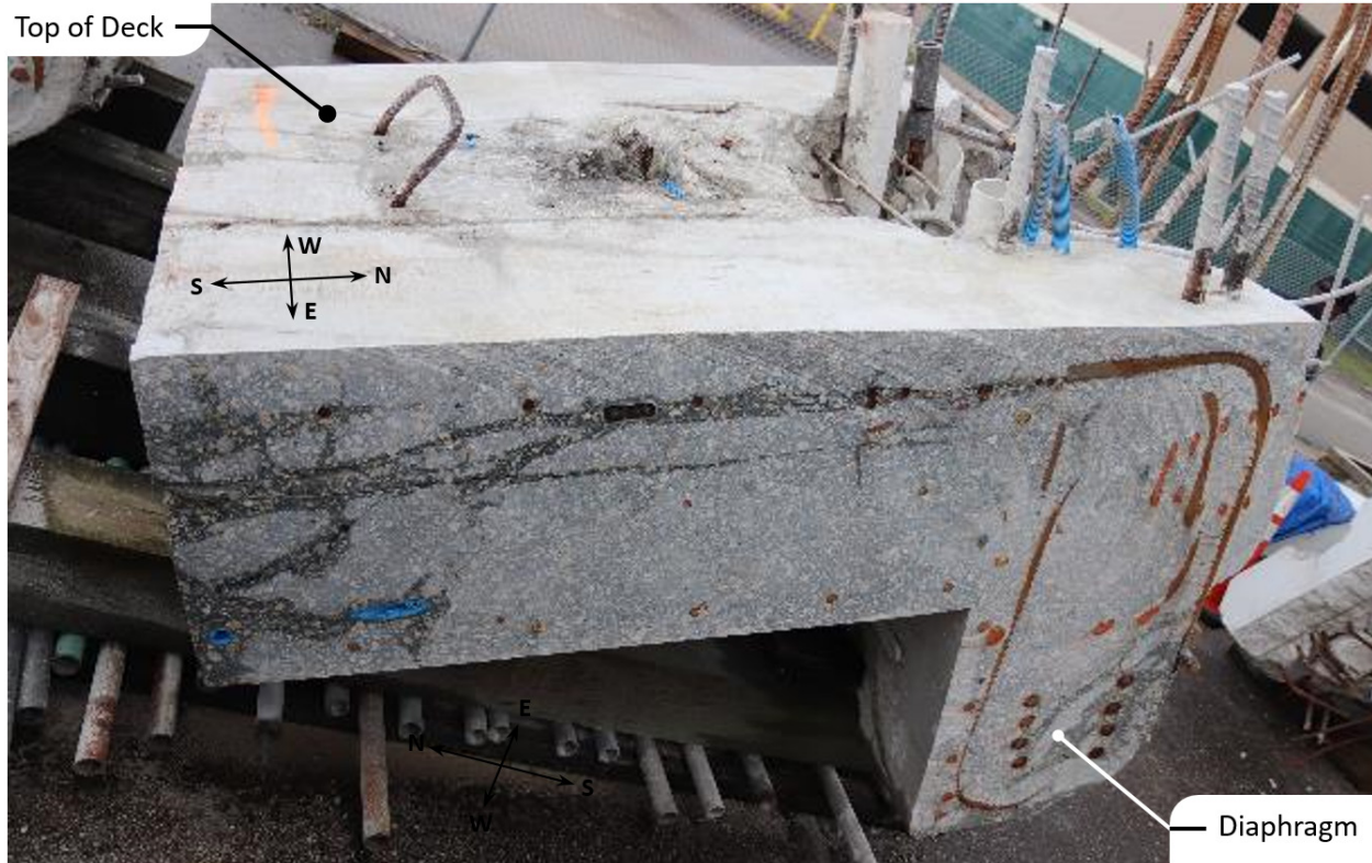
Figure 53. Photograph of longitudinal cross section of bridge deck after being cut from retained nodal region deck element. The vertical cut is approximately 20-inches east of the east face of member 12.
