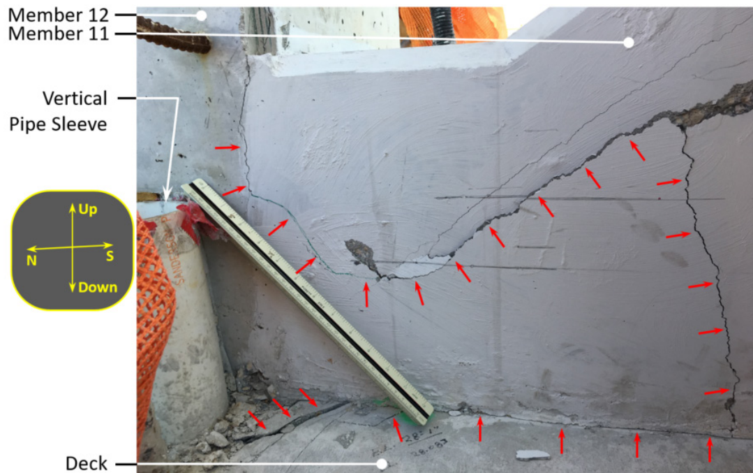
Figure 38. Photograph showing the west face of truss member 11 where it meets the deck on March 14, 2018 at 1:45 p.m. Corresponds to Bridge Factors Factual Report Photo 92.
