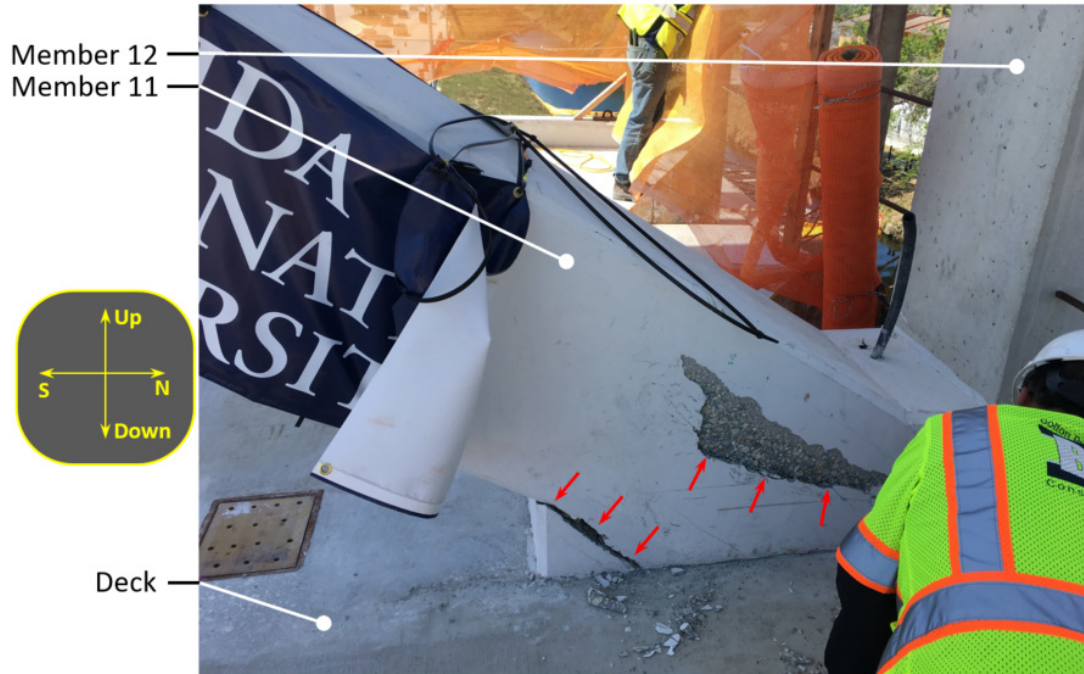
Figure 37. Photograph showing the east face of truss member 11 where it meets the deck on March 14, 2018 at 1:42 p.m. Corresponds to Bridge Factors Factual Report Photo 90.
