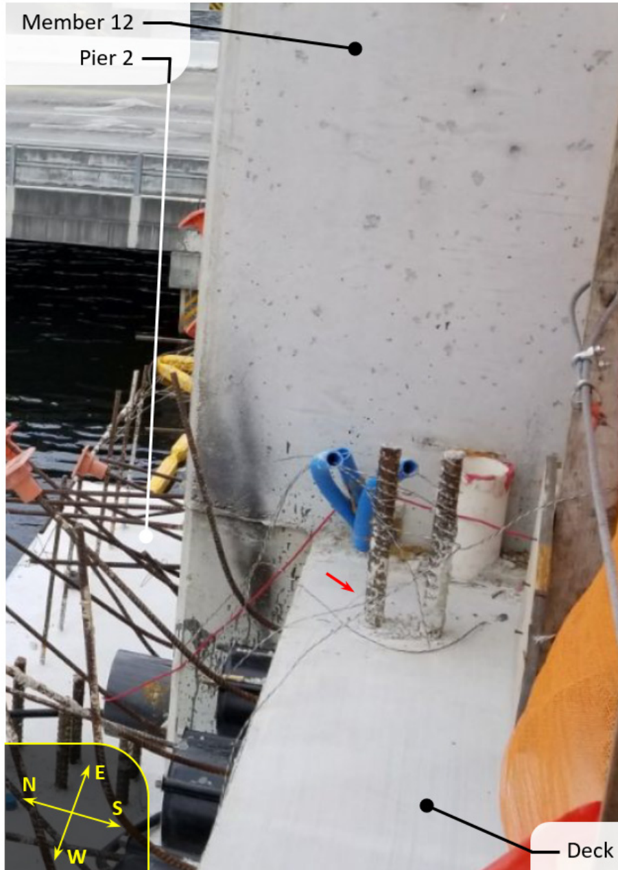
Figure 19. Photograph showing west side of member 12 at the deck after SPMT transport. Captured on March 10, 2018. Corresponds to Bridge Factors Factual Report Photo “MCM’s Photo Submission MCM-3”.
