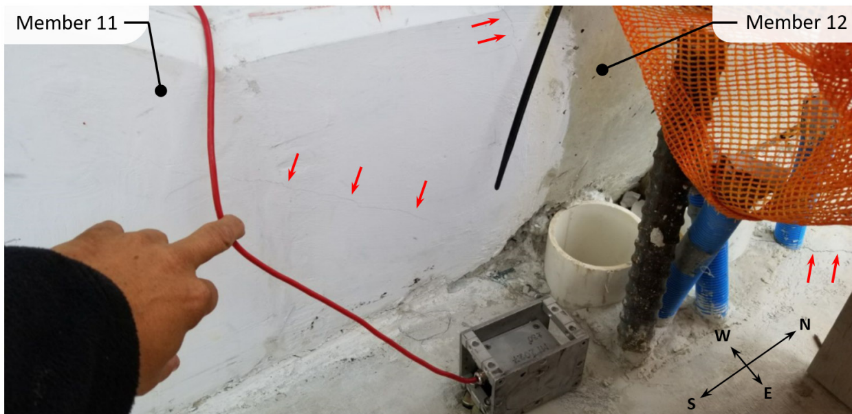
Figure 18. Photograph showing east side of members 11 and 12 at the deck after SPMT transport. Captured on March 10, 2018. Corresponds to Bridge Factors Factual Report Photo "MCM's Photo Submission MCM-4".
