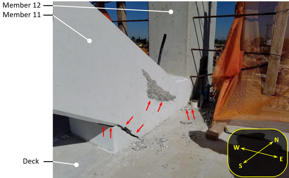
Figure 45. Photograph showing the east face of truss member 11 where it met the deck on March 15, 2018 at 10:53 a.m. Corresponds to Bridge Factors Factual Report Photo 102.
