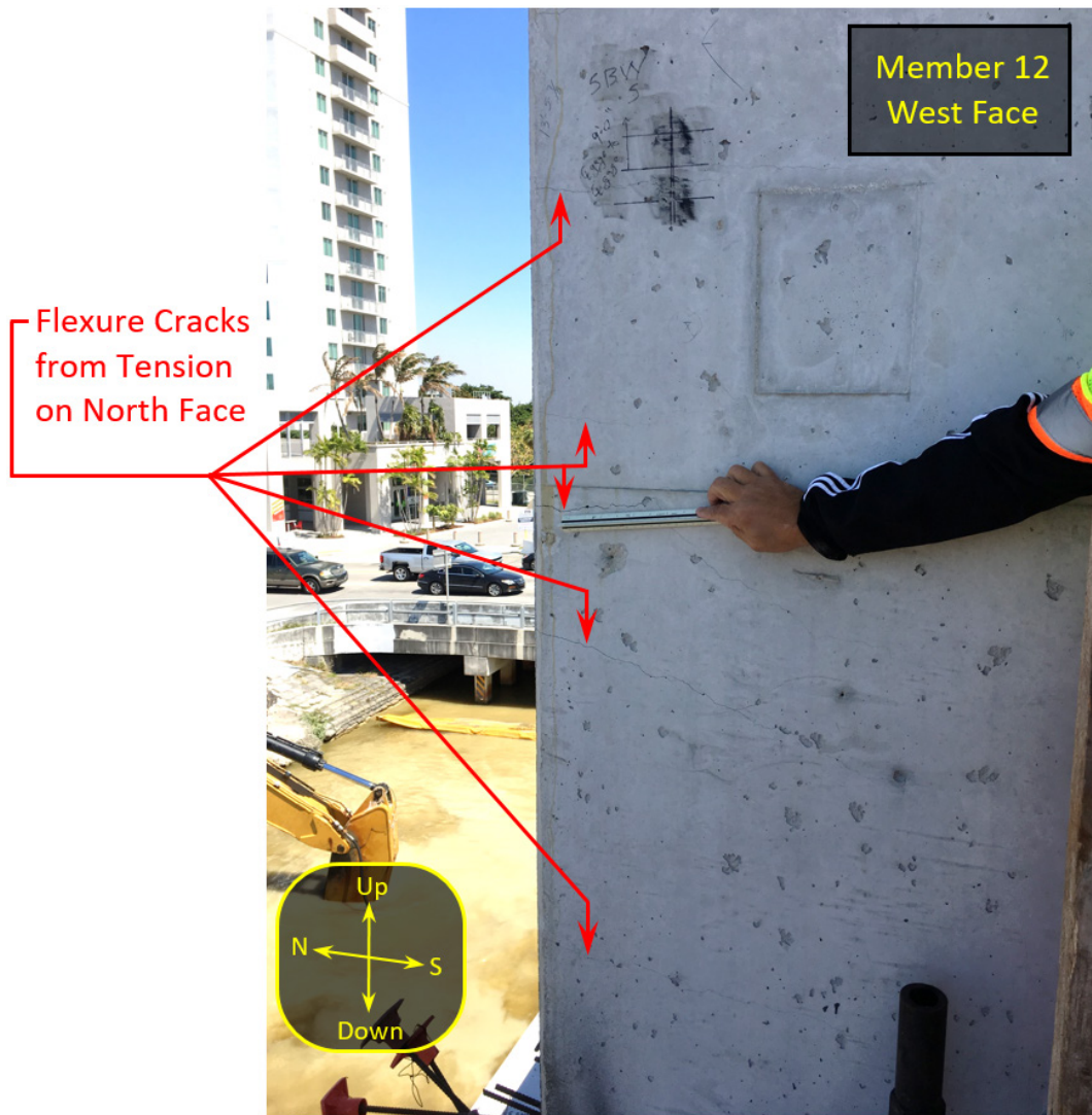
Figure 41. Photograph showing the west face of truss member 12 on March 14, 2018 at 1:51 p.m. Corresponds to Bridge Factors Factual Report Photo 100.
