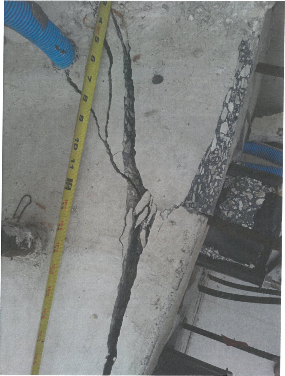
PHOTO 15: Diaphragm 2, Eastside Top view cracks
