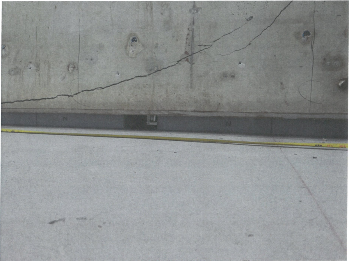
PHOTO 13: Diaphragm 2, Eastside North view cracks
