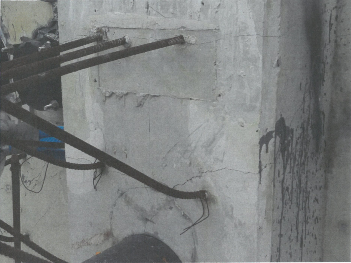
PHOTO 8: Truss 12, North view cracks
