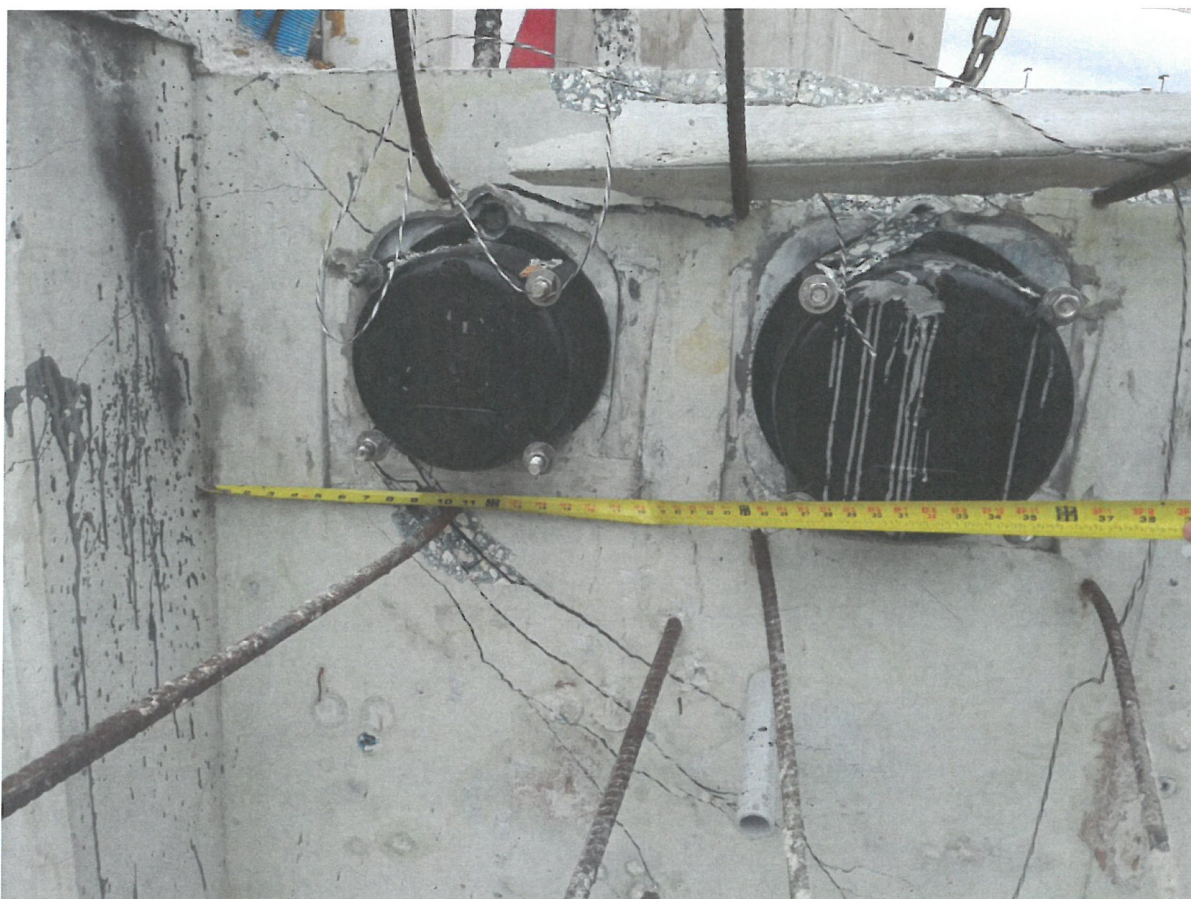
PHOTO 6: Diaphragm 2, Westside North view cracks
