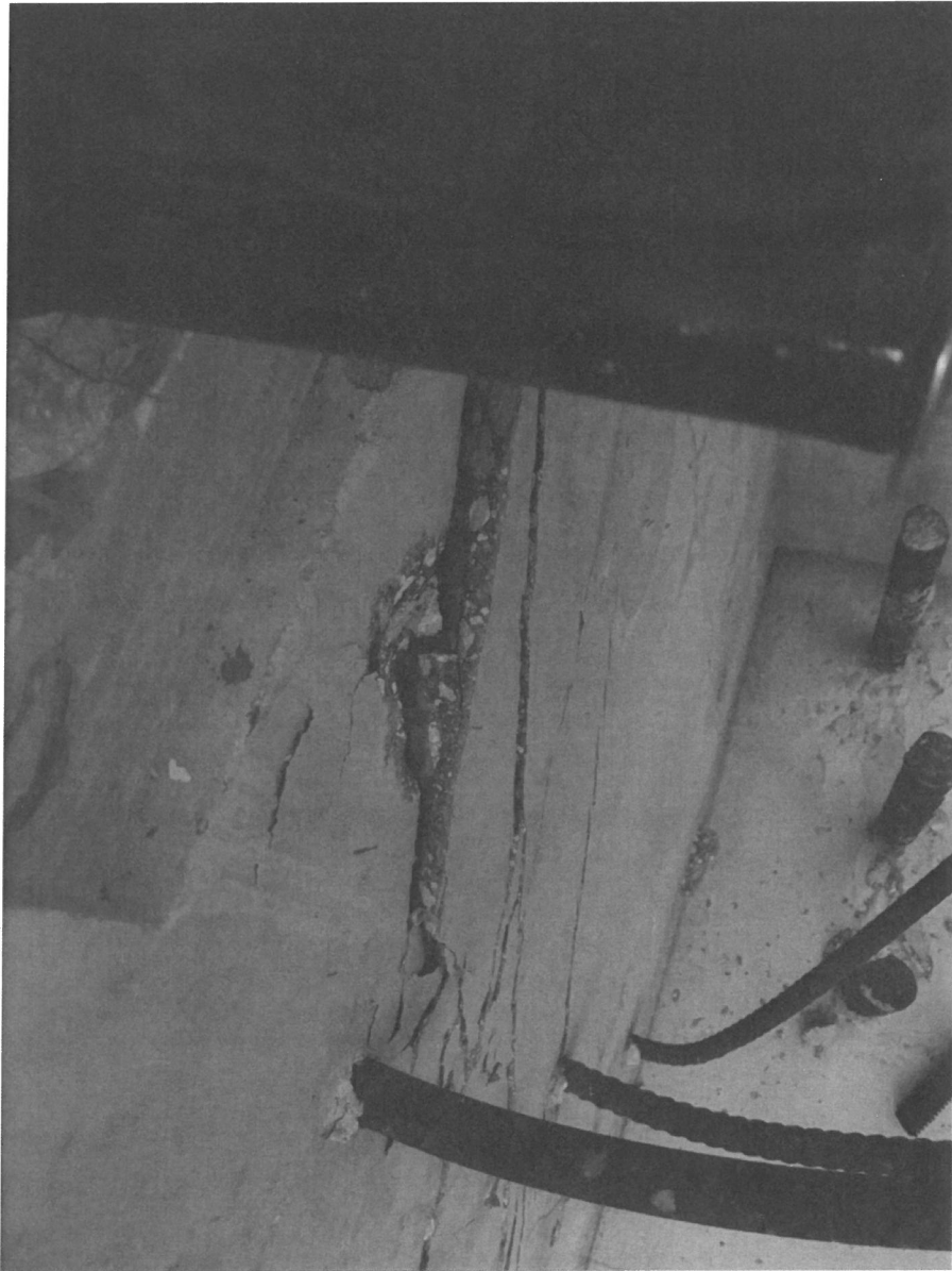
PHOTO 16: Diaphragm 2, Eastside Top/side view cracks
