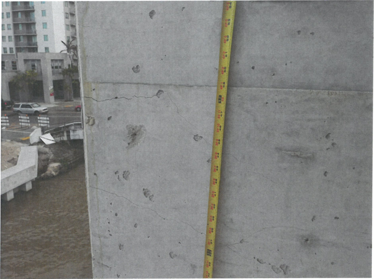
PHOTO 2: Truss 12, Westside hair cracks
