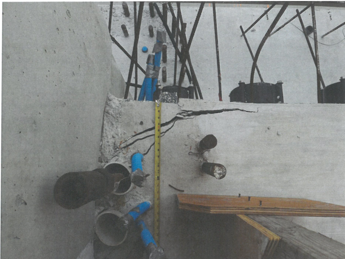
PHOTO 5: Diaphragm 2, Eastside top view crack
