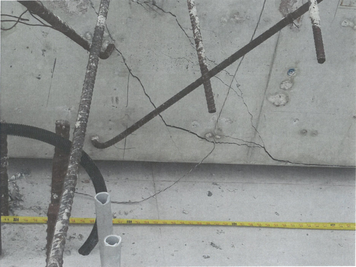
PHOTO 9: Diaphragm 2, Westside North view cracks
