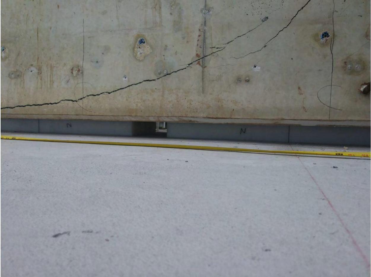
PHOTO 13: Diaphragm 2, Eastside North view cracks
