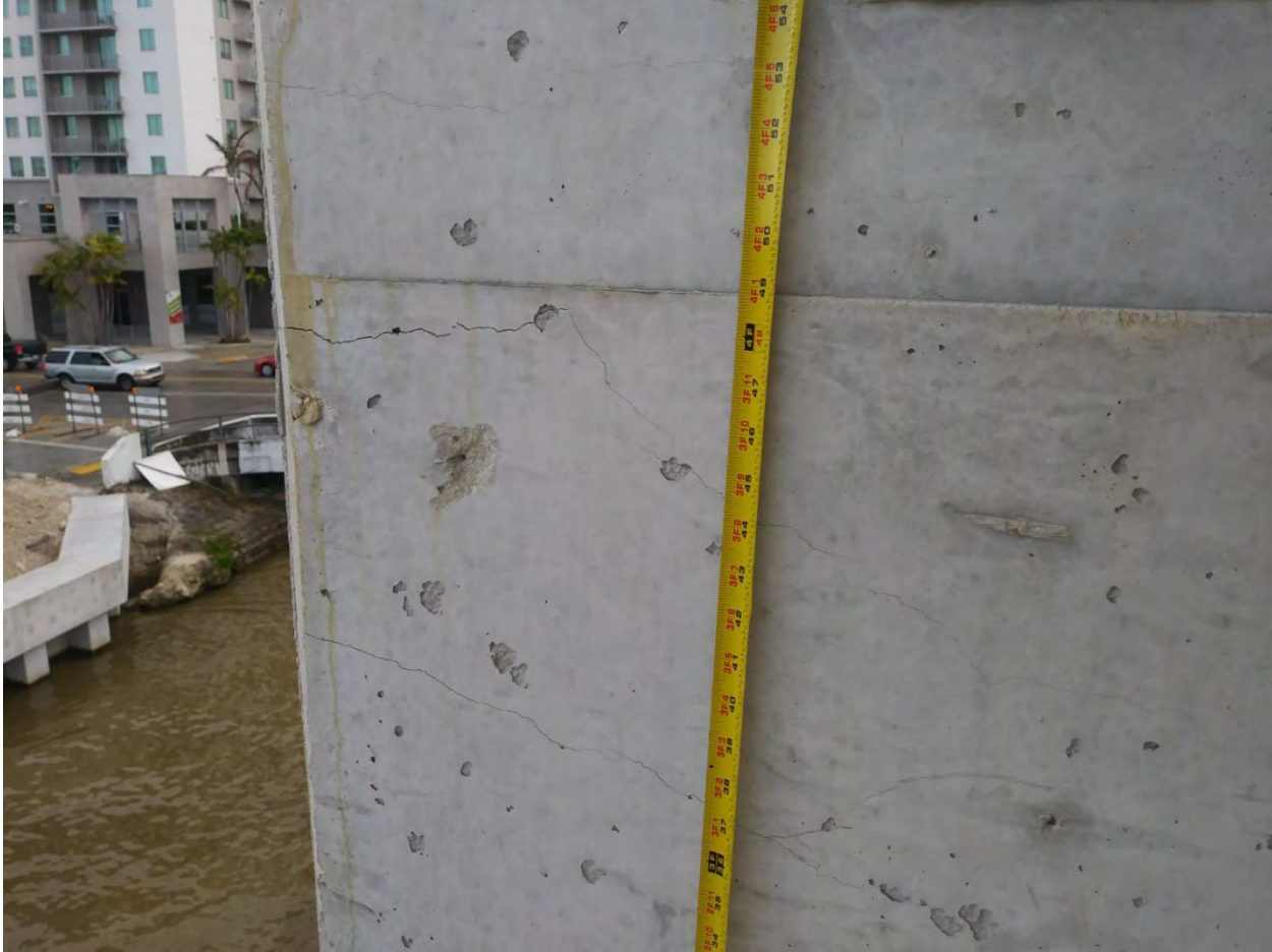
PHOTO 2: Truss 12, Westside hair cracks
