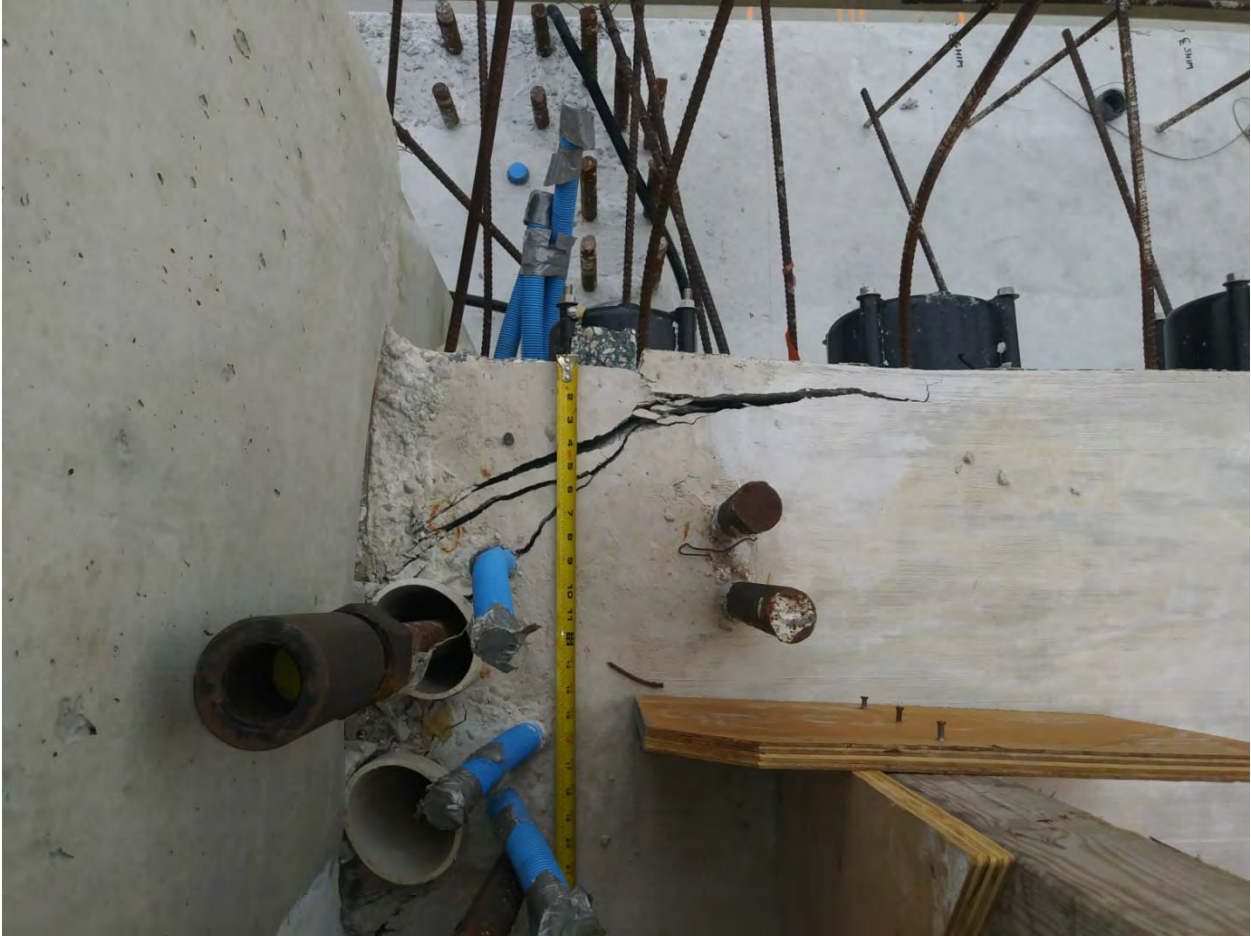
PHOTO 5: Diaphragm 2, Eastside top view crack
