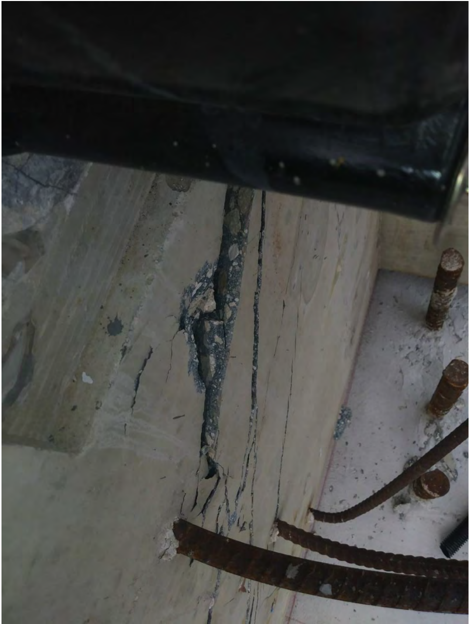
PHOTO 16: Diaphragm 2, Eastside Top/side view cracks
