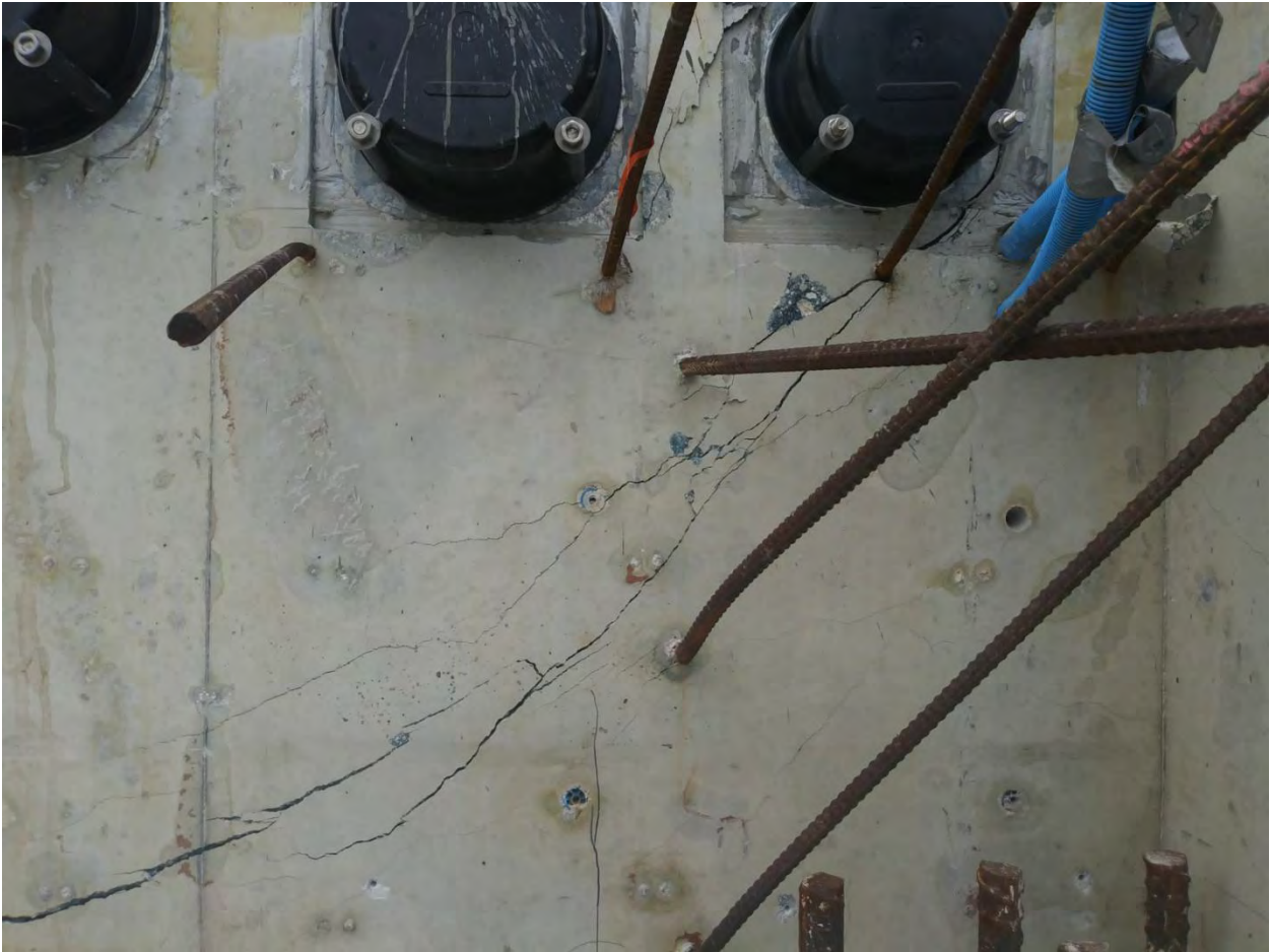
PHOTO 14: Diaphragm 2, Eastside North view cracks
