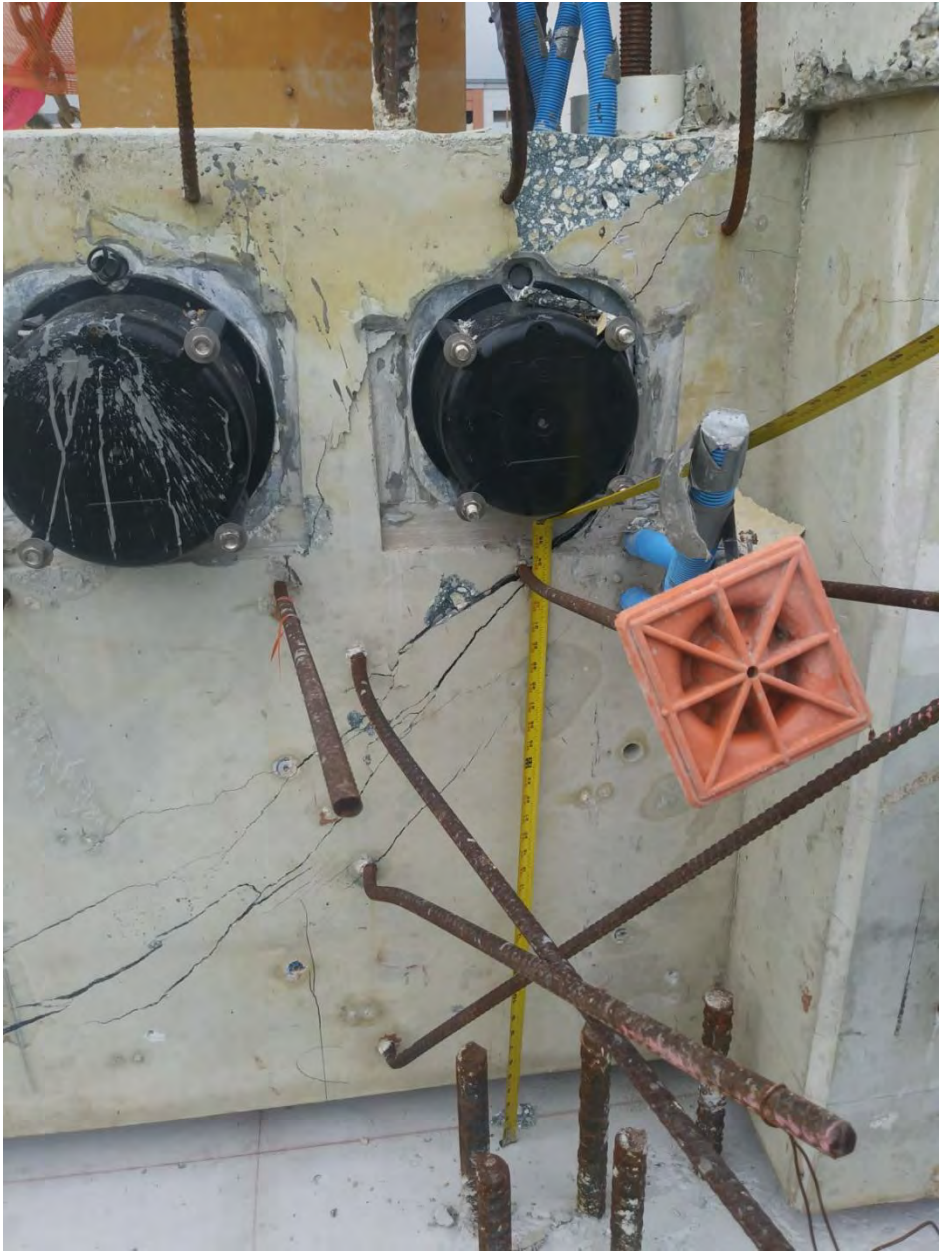
PHOTO 11: Diaphragm 2, Eastside North view cracks
