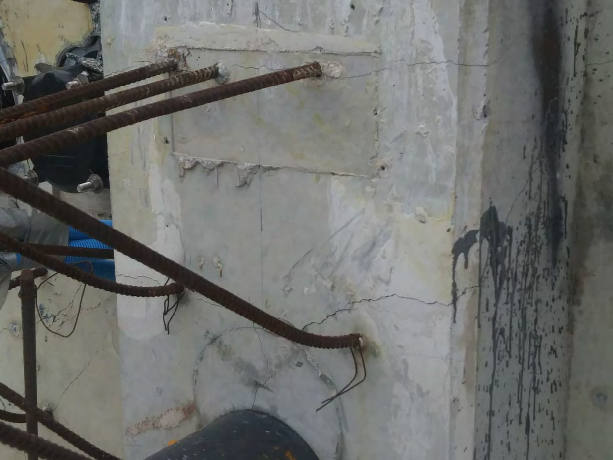
PHOTO 8: Truss 12, North view cracks
