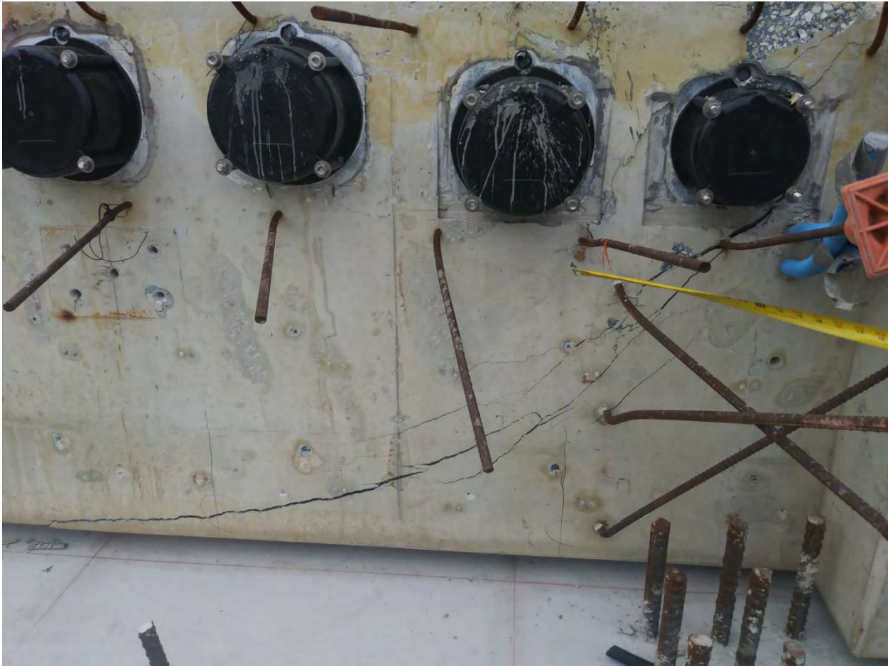
PHOTO 12: Diaphragm 2, Eastside North view cracks
