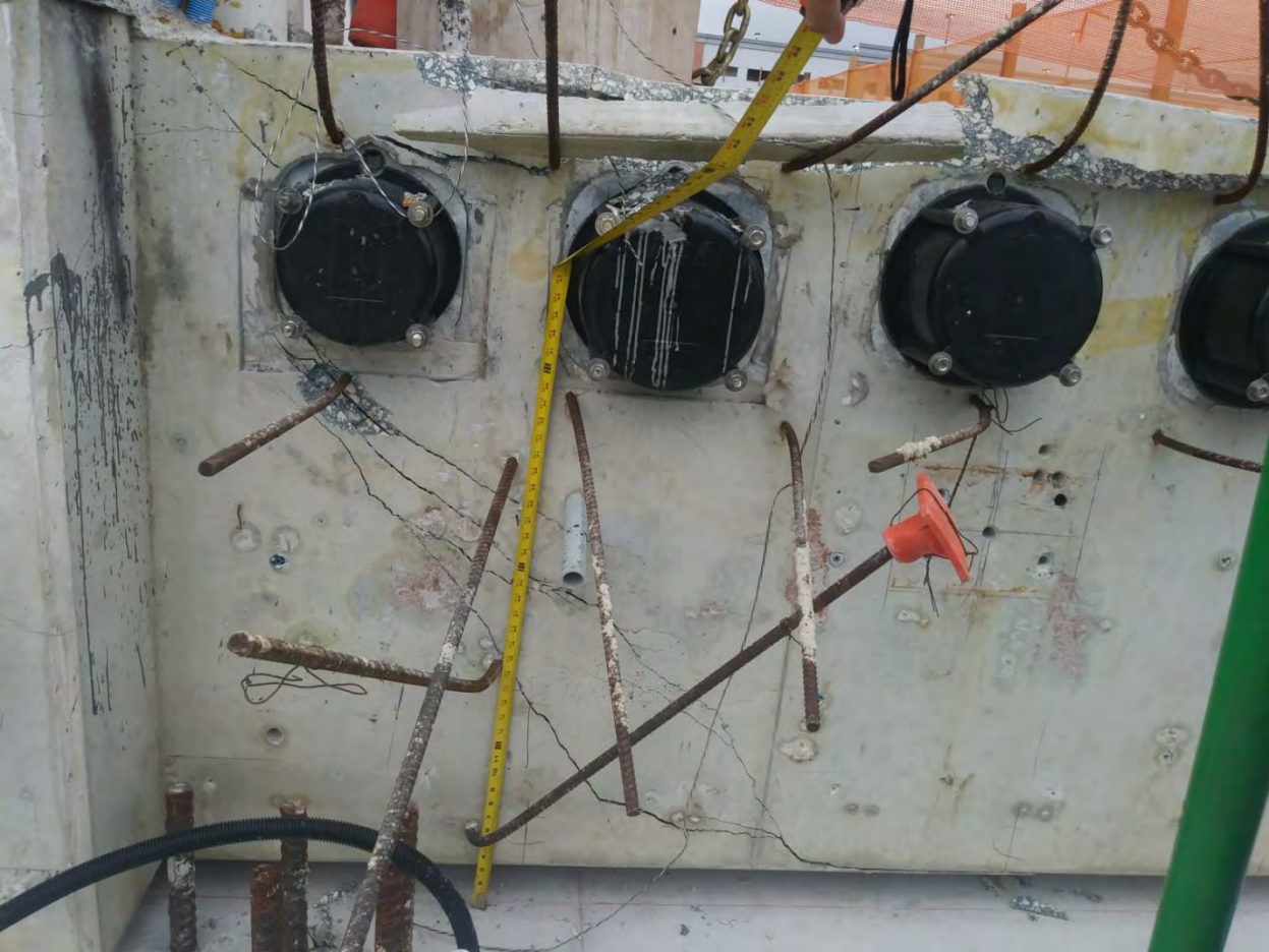
PHOTO 7: Diaphragm 2, Westside North view cracks
