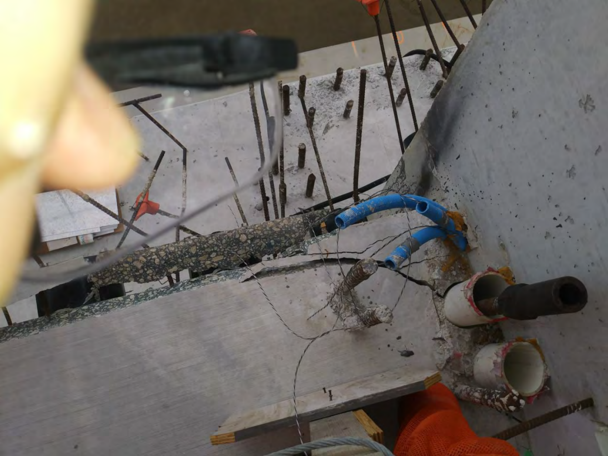
PHOTO 1: Diaphragm 2, Westside top view, crack
