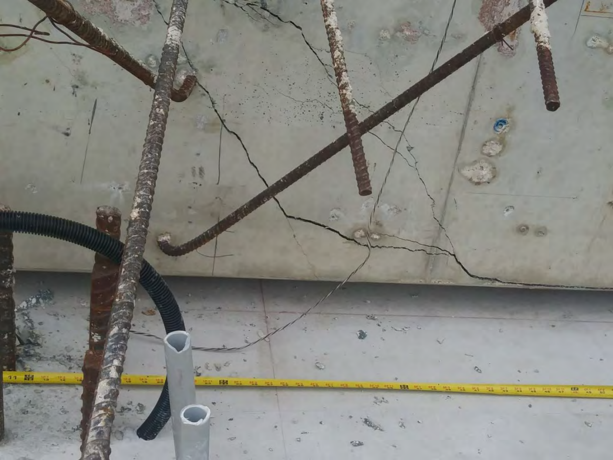
PHOTO 9: Diaphragm 2, Westside North view cracks
