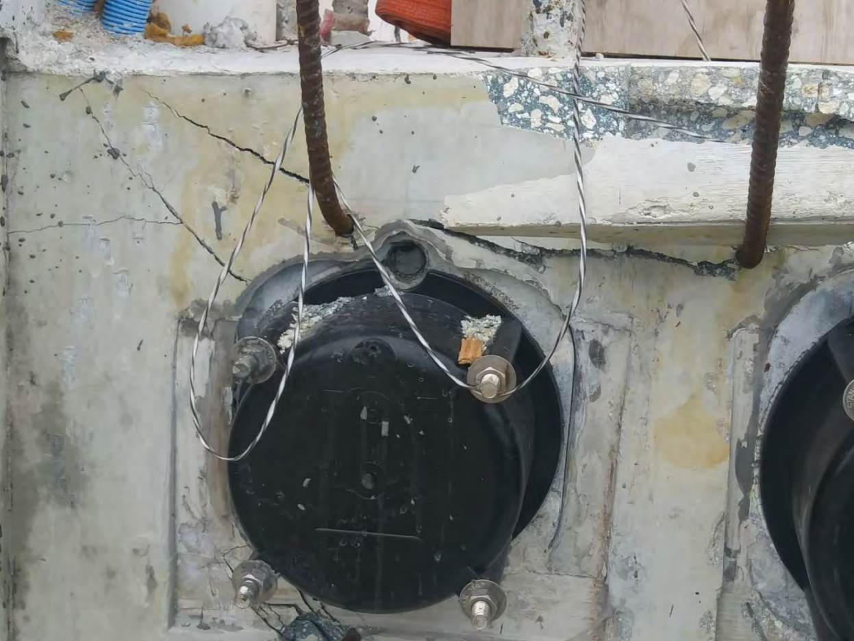
PHOTO 10: Diaphragm 2, Westside North view cracks
