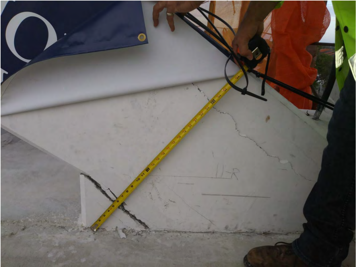
PHOTO 3: Truss 11, Eastside cracks
