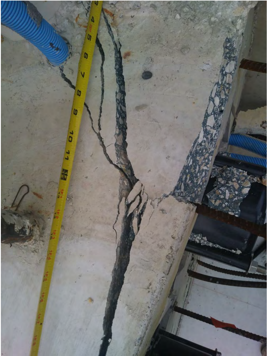
PHOTO 15: Diaphragm 2, Eastside Top view cracks
