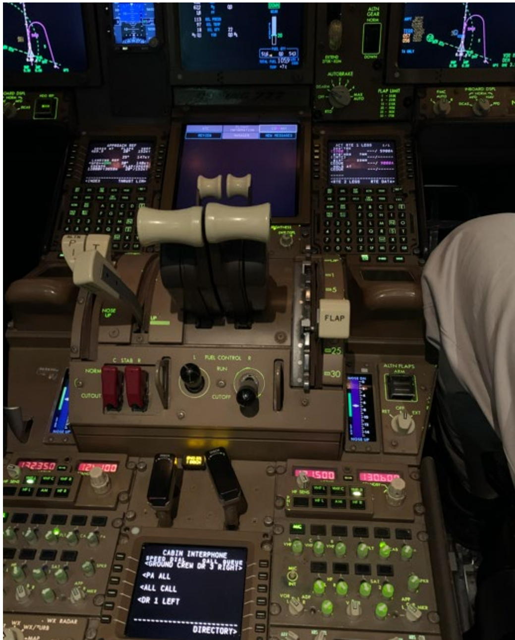
Photo 9: Engine still on fire with no indication to the crew that the detection loops burned through.
