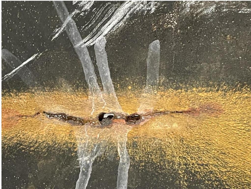
Unprepared ID Surface
