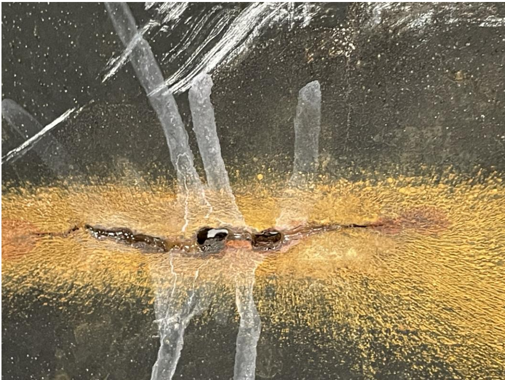
Unprepared ID Surface
