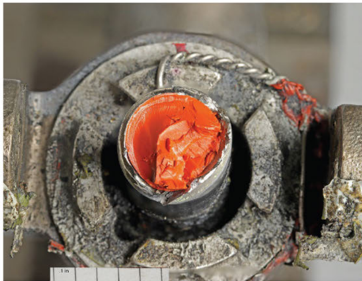
Figure 95. Close-up of fracture surface at cylinder end
