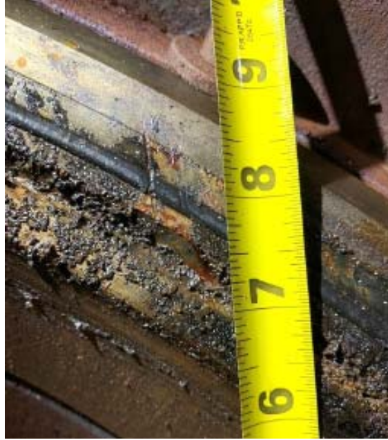
Figure 6. Photo of scratches in the outer seat ring and O-ring of the 24" mainline valve (from NTSB Materials Laboratory Factual Report No. 21-094).
