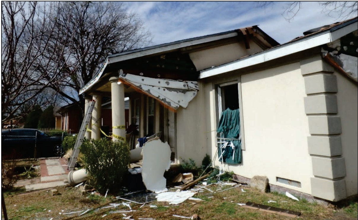
Figure 14. Photo of 3527 Durango Drive Post-Incident by NTSB.
