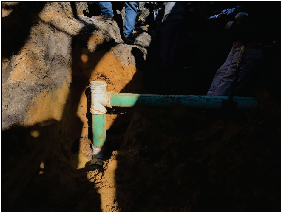
Figure 31. Sewer lateral from 3539 Durango Drive Connection to Sanitary Sewer Main, Facing East (Photograph by Atmos Energy, 3/7/18)
