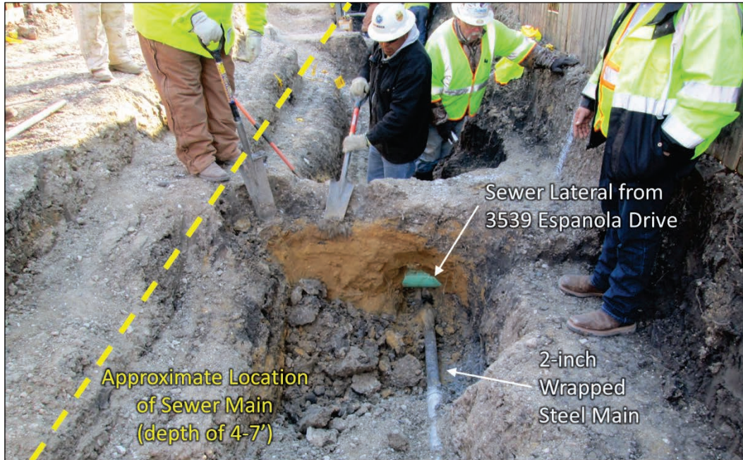
Figure 27. Sewer Lateral from 3539 Espanola Drive at Excavation #8 Facing East (Photograph by TX-RRC, 3/6/18)
