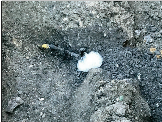
Figure 25. Photograph of Leak on Threads of 3524 Espanola Drive Service Tee and Service Tee Cap (Photograph by Atmos Energy, 2/28/19)
