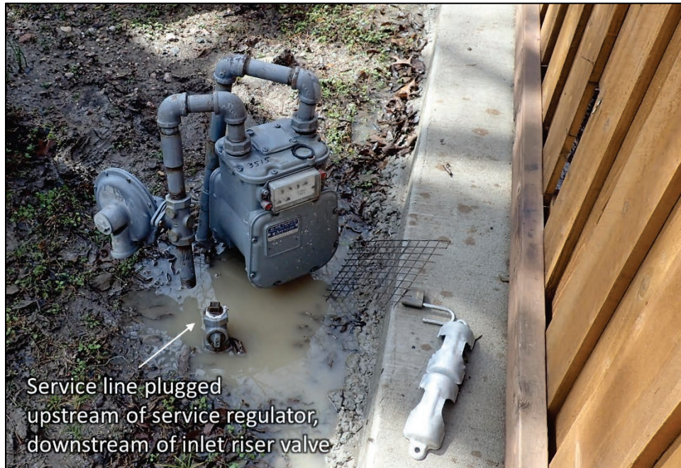
Figure 24. Example Service Line Preparation for Pressure Test. Meter-Regulator Set Shown is from 3515 Durango Drive. Photo by Baker-Risk on Behalf of Atmos Energy: 2/24/18 at 2:49PM.
