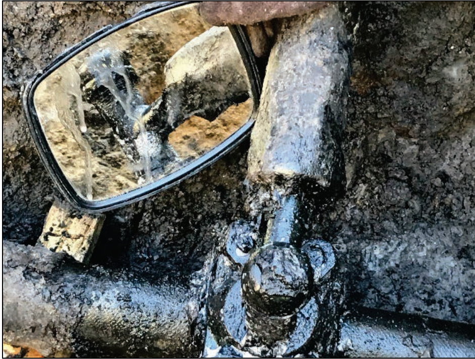
Figure 30. Photograph of Leak on 3539 Durango Drive Service Tap (Photograph by Atmos Energy, 3/7/18)
