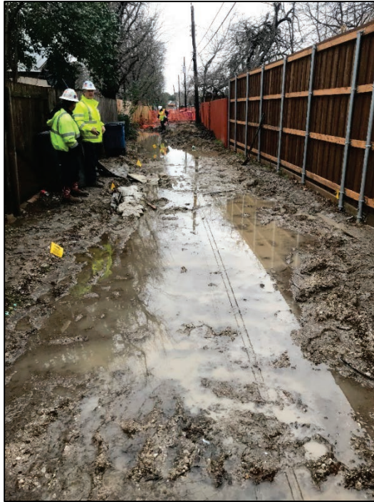
Figure 20. Alley Behind 3534 Espanola Drive Prior to Excavation. Wet muddy soil and puddles of standing water are shown. Photograph by Atmos Energy, 3/01/18.
