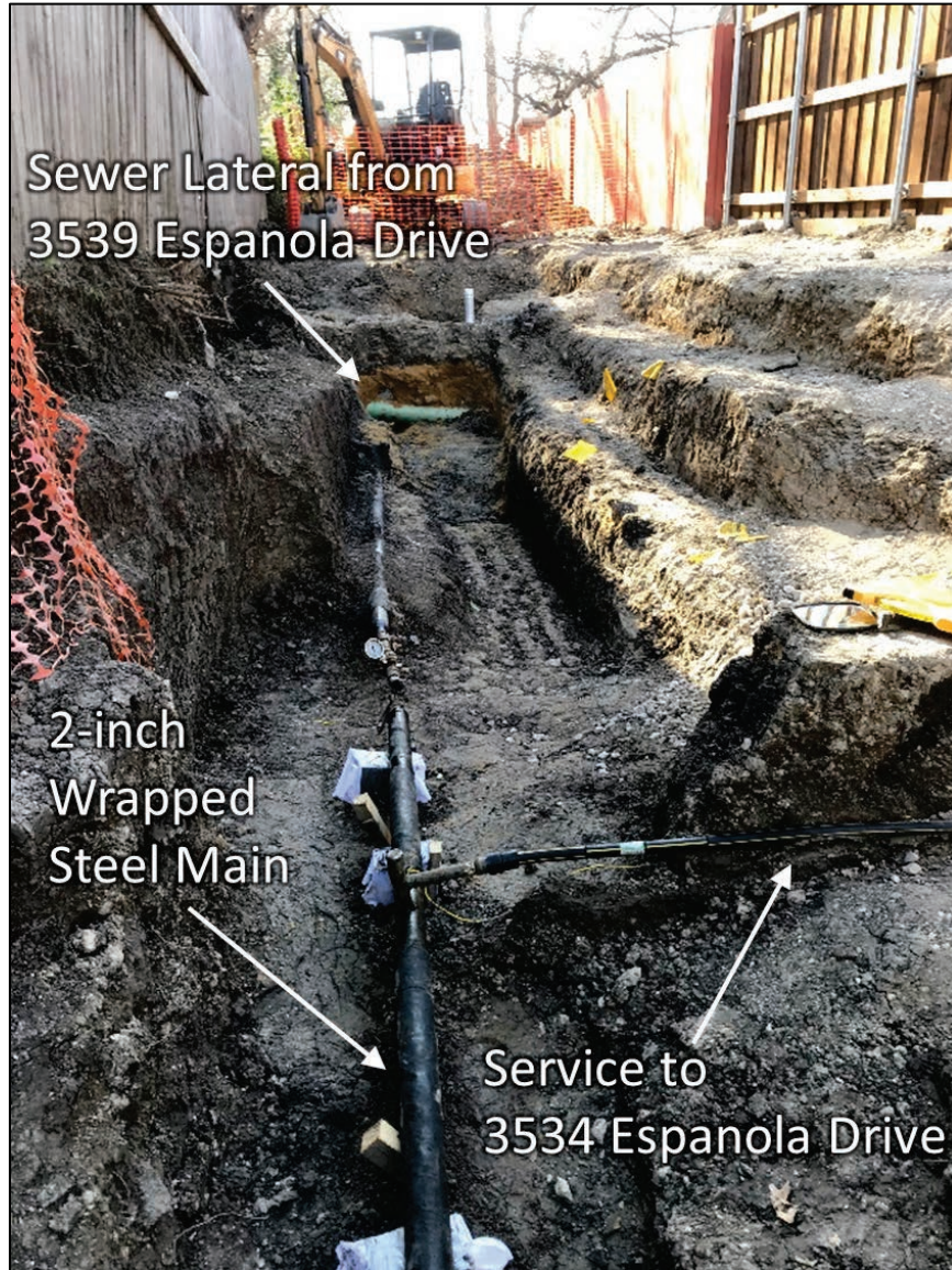
Figure 28. View from Excavation #7 Facing West Towards 3539 Espanola Drive Sewer Lateral (Photograph by Atmos Energy, 3/6/18)
