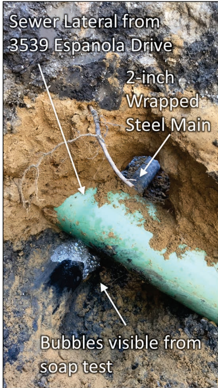
Figure 29. Soap Bubbles from 2-inch gas main at 3539 Durango Drive sewer lateral crossing (Photograph by Atmos Energy, 3/6/18)
