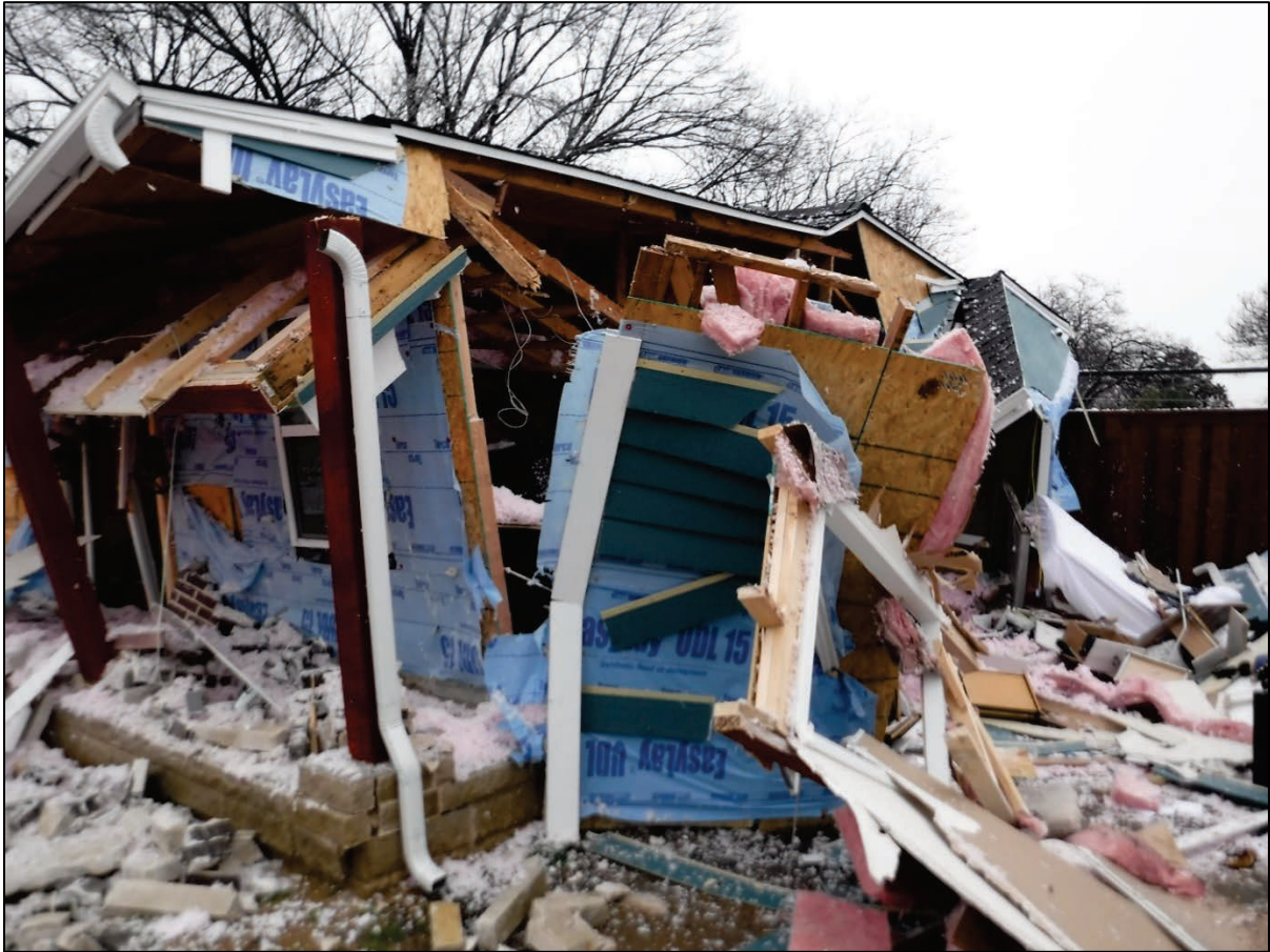
Figure 21. Northwest corner of 3534 Espanola Drive, Photo Taken Post-Accident on 2/23/18 by DFR
