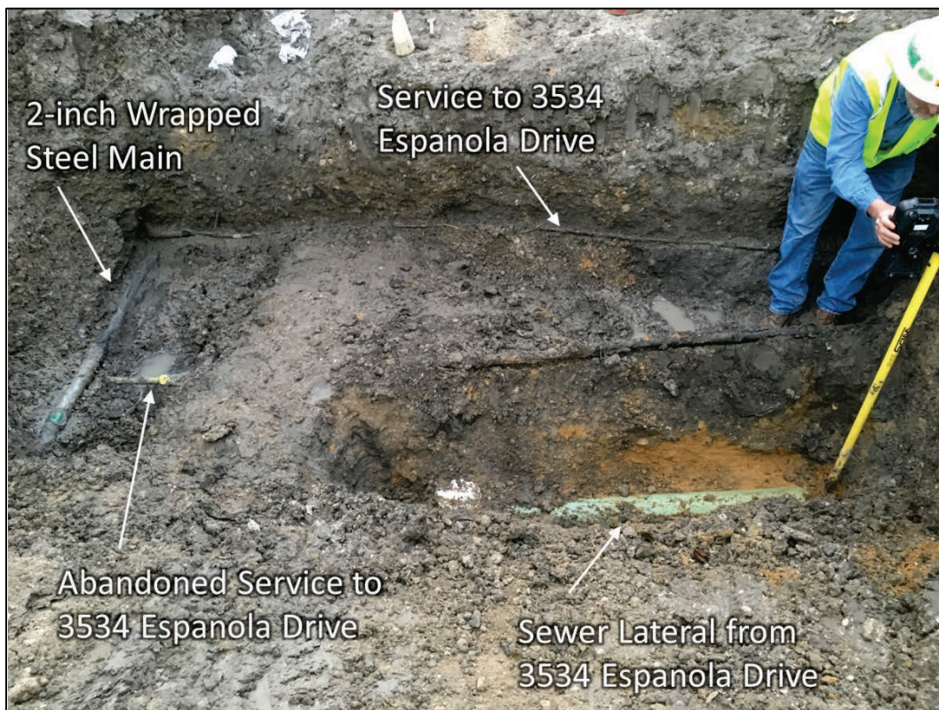
Figure 26. Sewer Lateral from 3534 Espanola Drive at Excavation #7 facing west (Photograph by PHMSA, 3/1/18)
