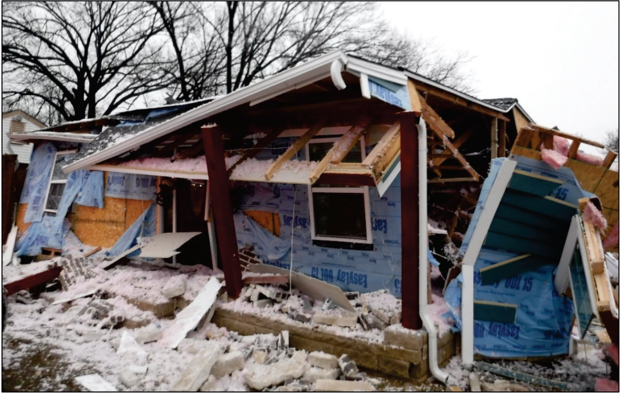
Figure 1. Front of 3534 Espanola Drive after the Explosion. Photo by DFR on February 23, 2018.
