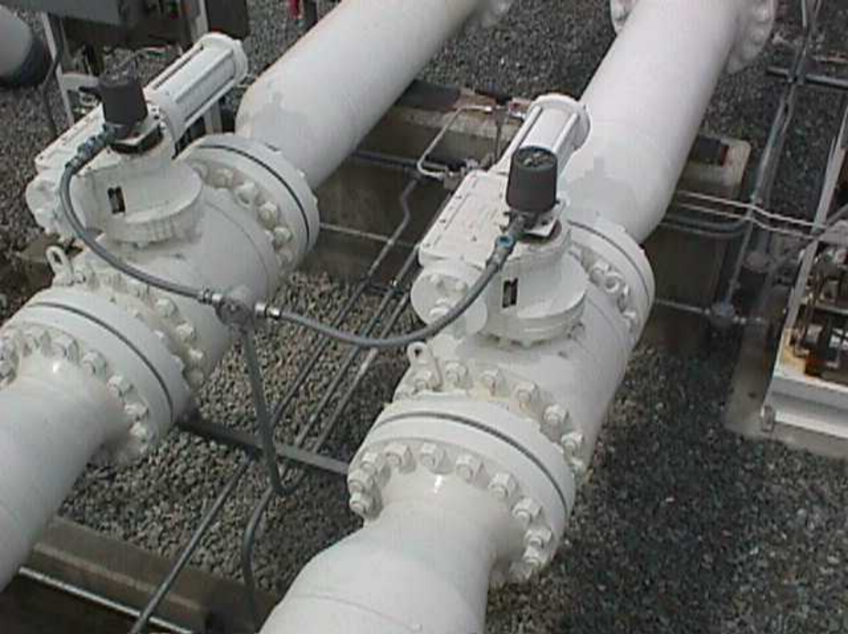
Appendix T to the Pipeline Operations Factual Report, Photo 4, Inlet control valves.
