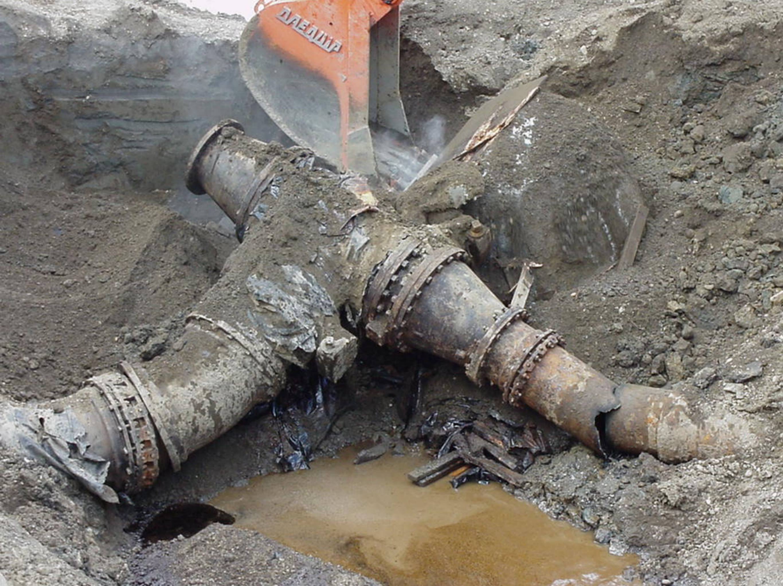
Appendix S to the Water Treatment Plant Factual Report, Photo 8, Removing waterline tee and thrust block.
