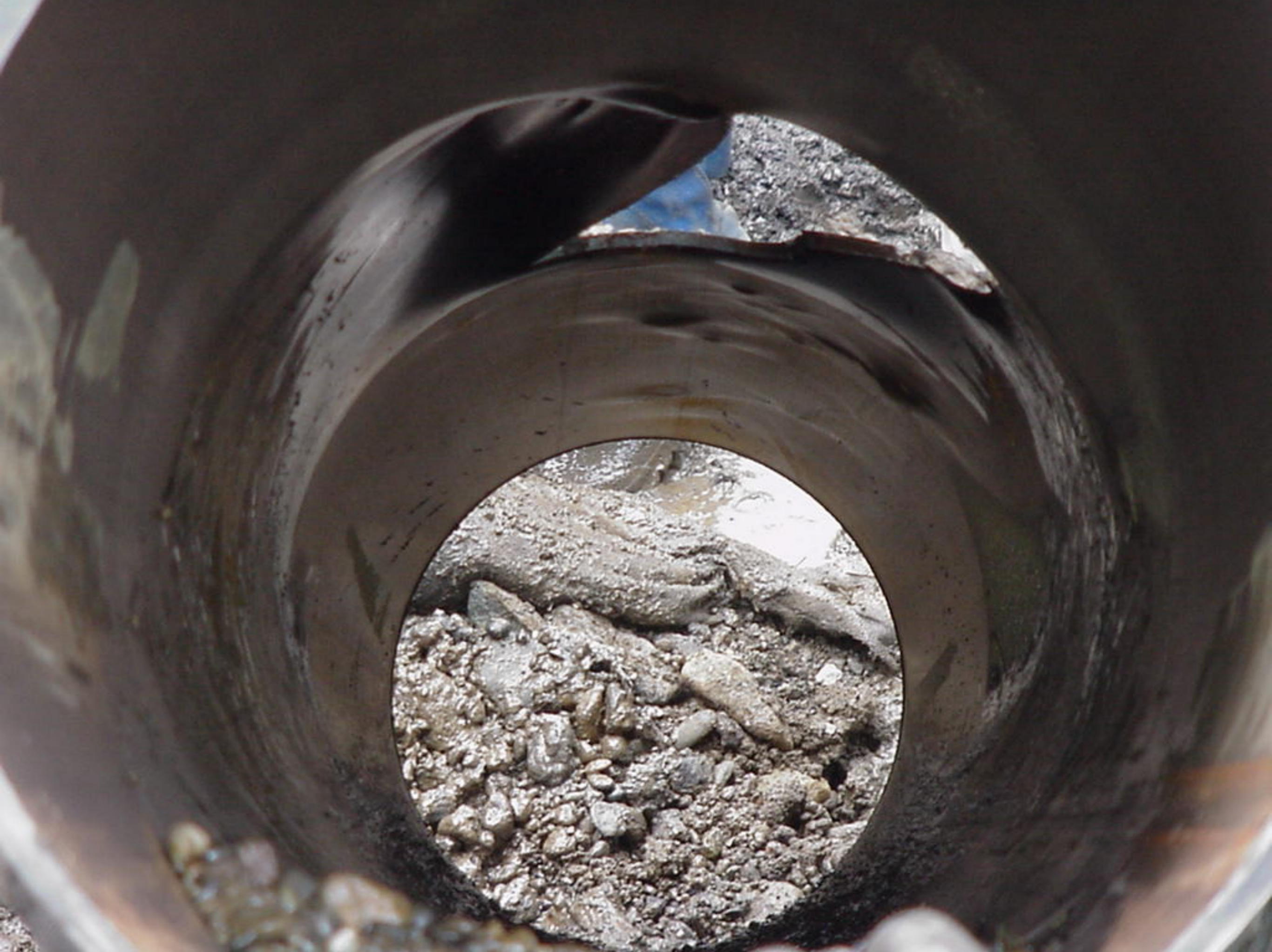
Appendix S to the Water Treatment Plant Factual Report, Photo 7, Internal view of damage to ruptured pipe segment.
