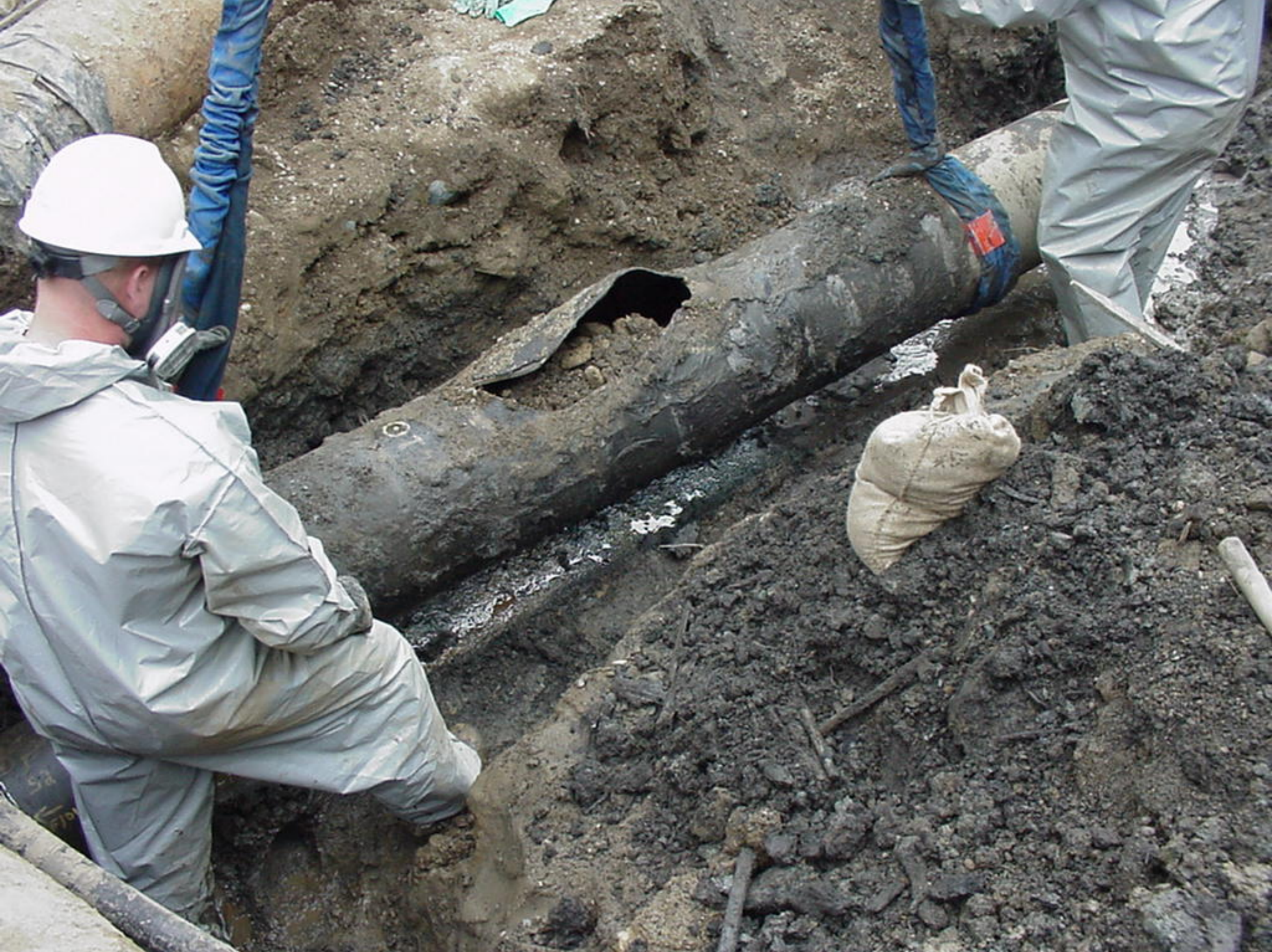
Appendix S to the Water Treatment Plant Factual Report, Photo 6, Removing ruptured pipe segment.
