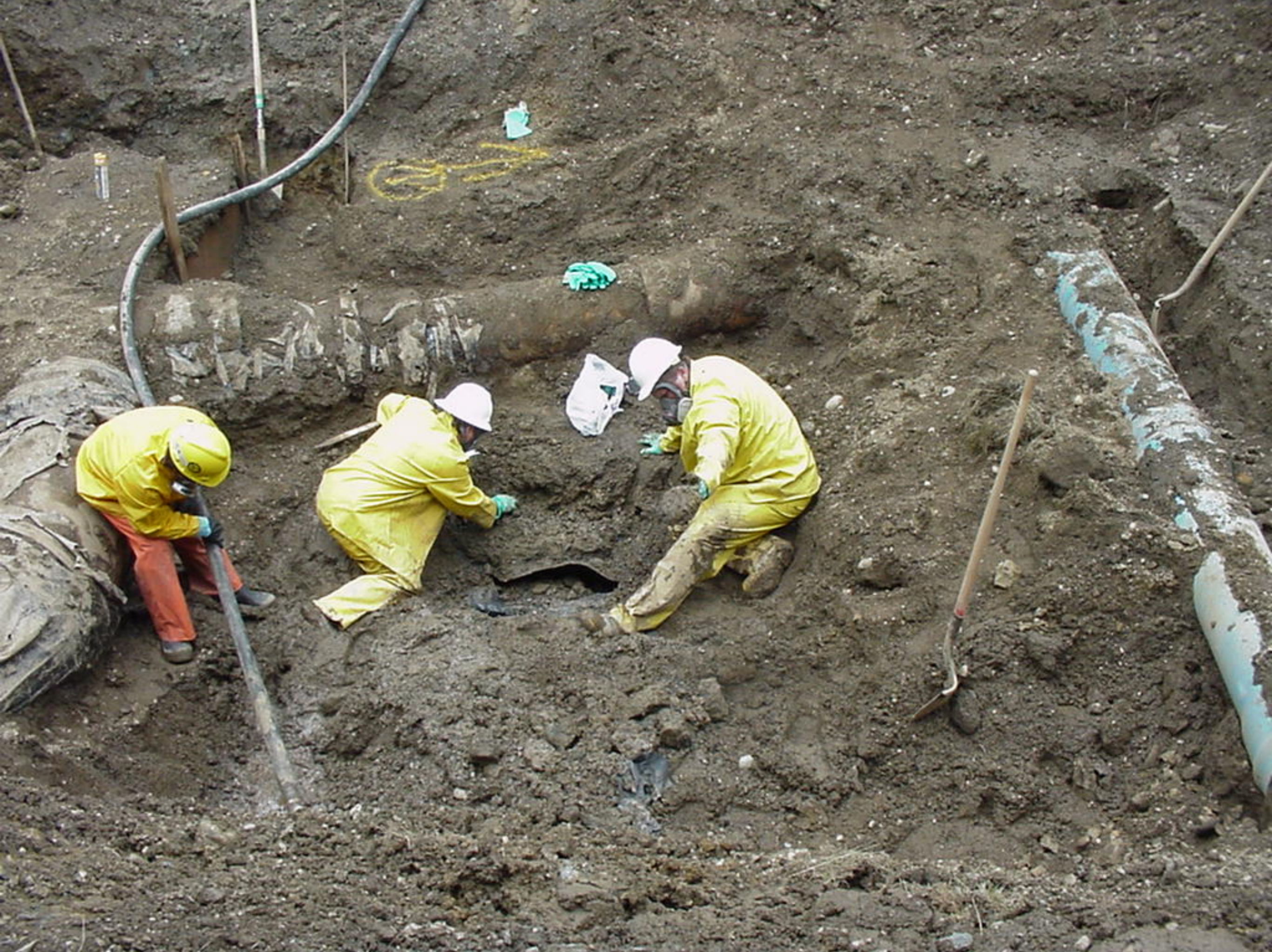
Appendix S to the Water Treatment Plant Factual Report, Photo 4, Exposing rupture in relation to waterline tee and PVC utility duct crossing.
