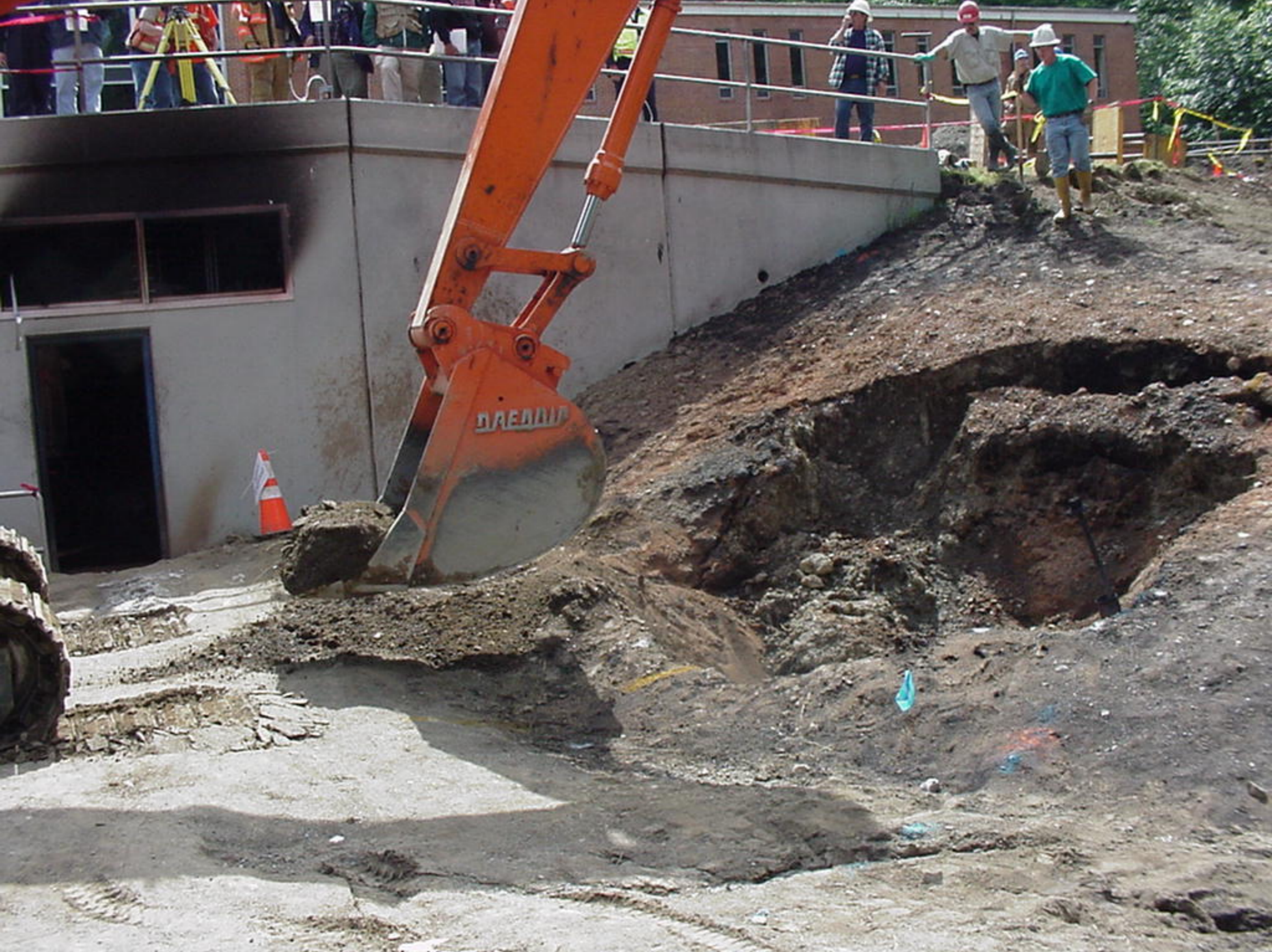
Appendix S to the Water Treatment Plant Factual Report, Photo 2, Beginning excavation to recover ruptured pipe.
