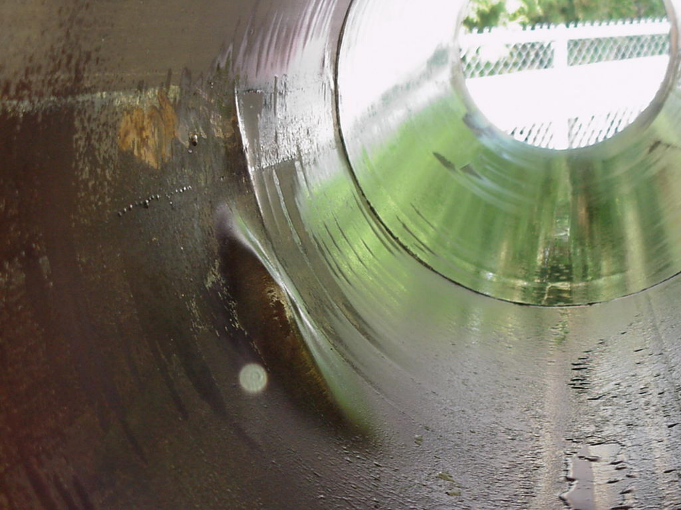
Appendix S to the Water Treatment Plant Factual Report, Photo 14, Internal view of damage to second pipe segment.
