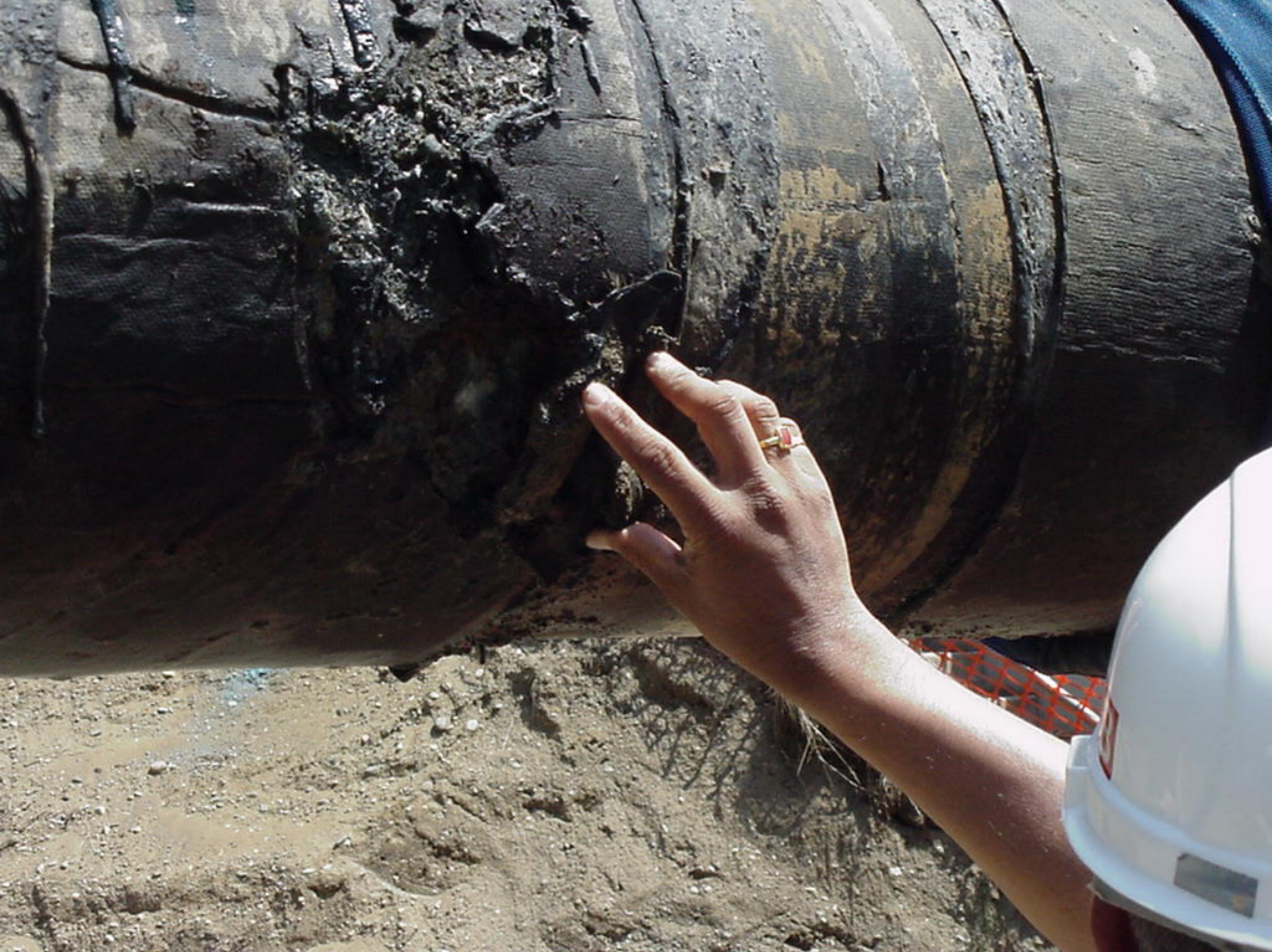
Appendix S to the Water Treatment Plant Factual Report, Photo 13, View of external damage to second pipe segment.
