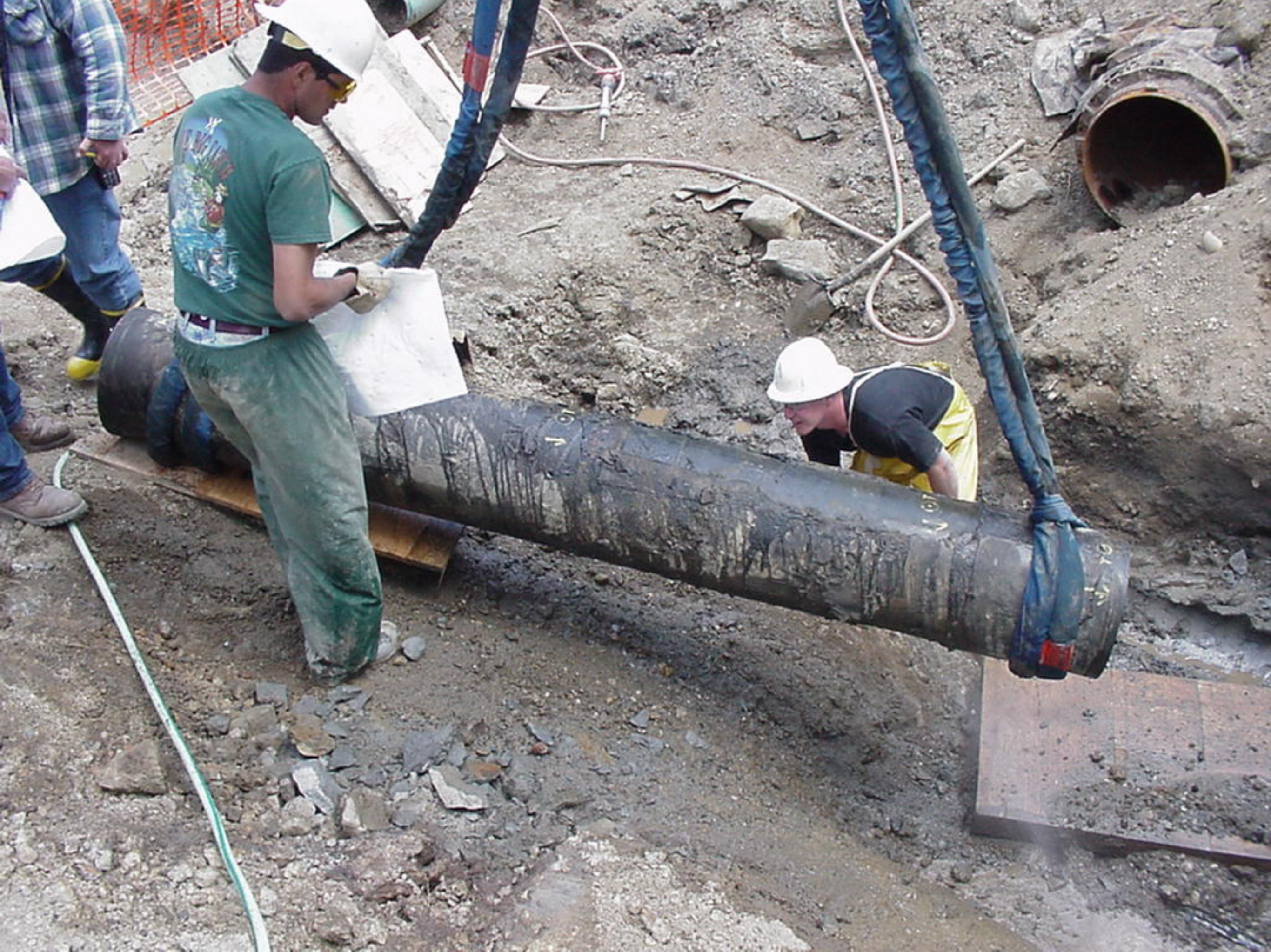
Appendix S to the Water Treatment Plant Factual Report, Photo 12, Removing second pipe segment.
