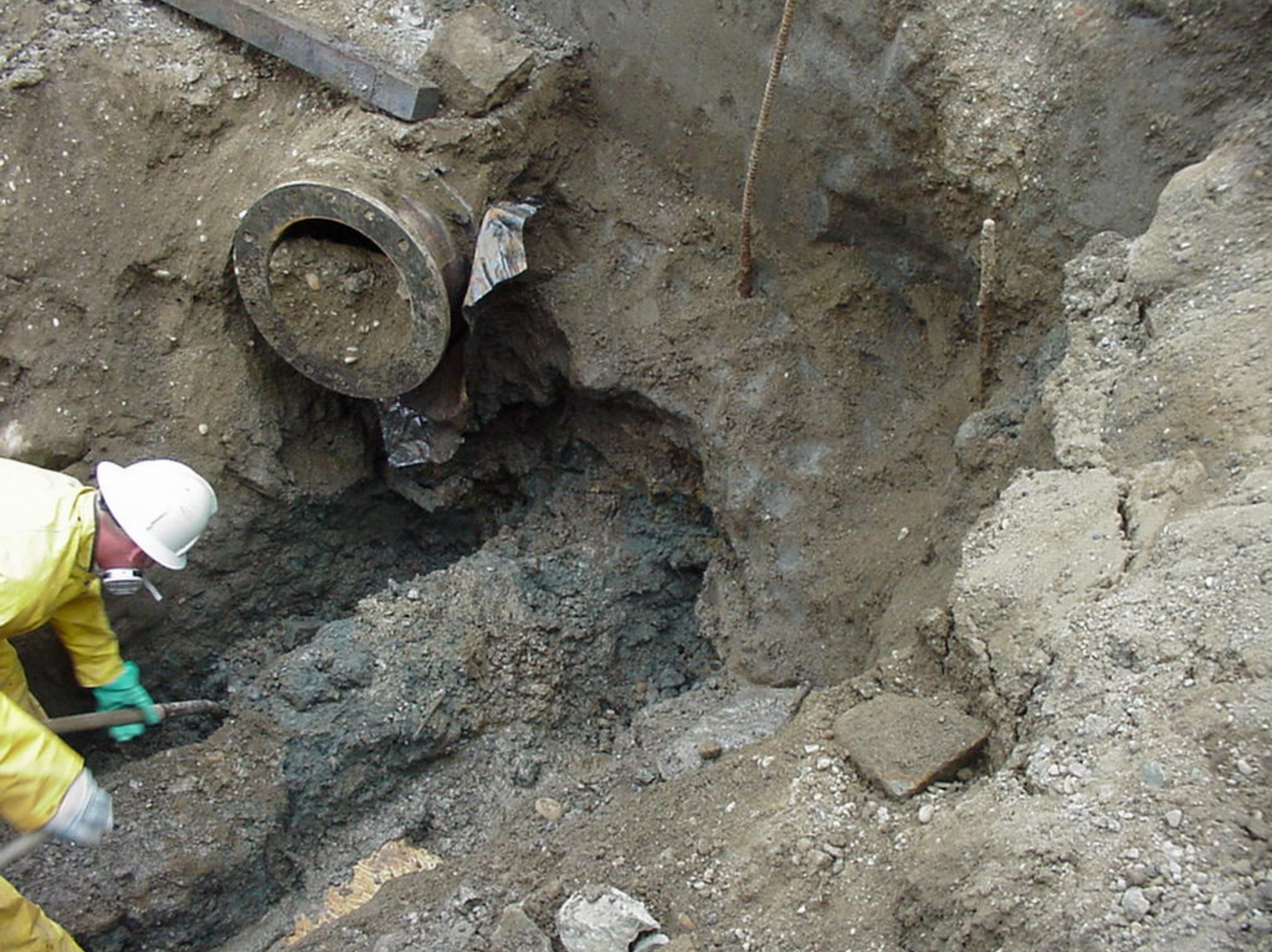
Appendix S to the Water Treatment Plant Factual Report, Photo 10, Excavating to remove second pipe segment containing anomaly.
