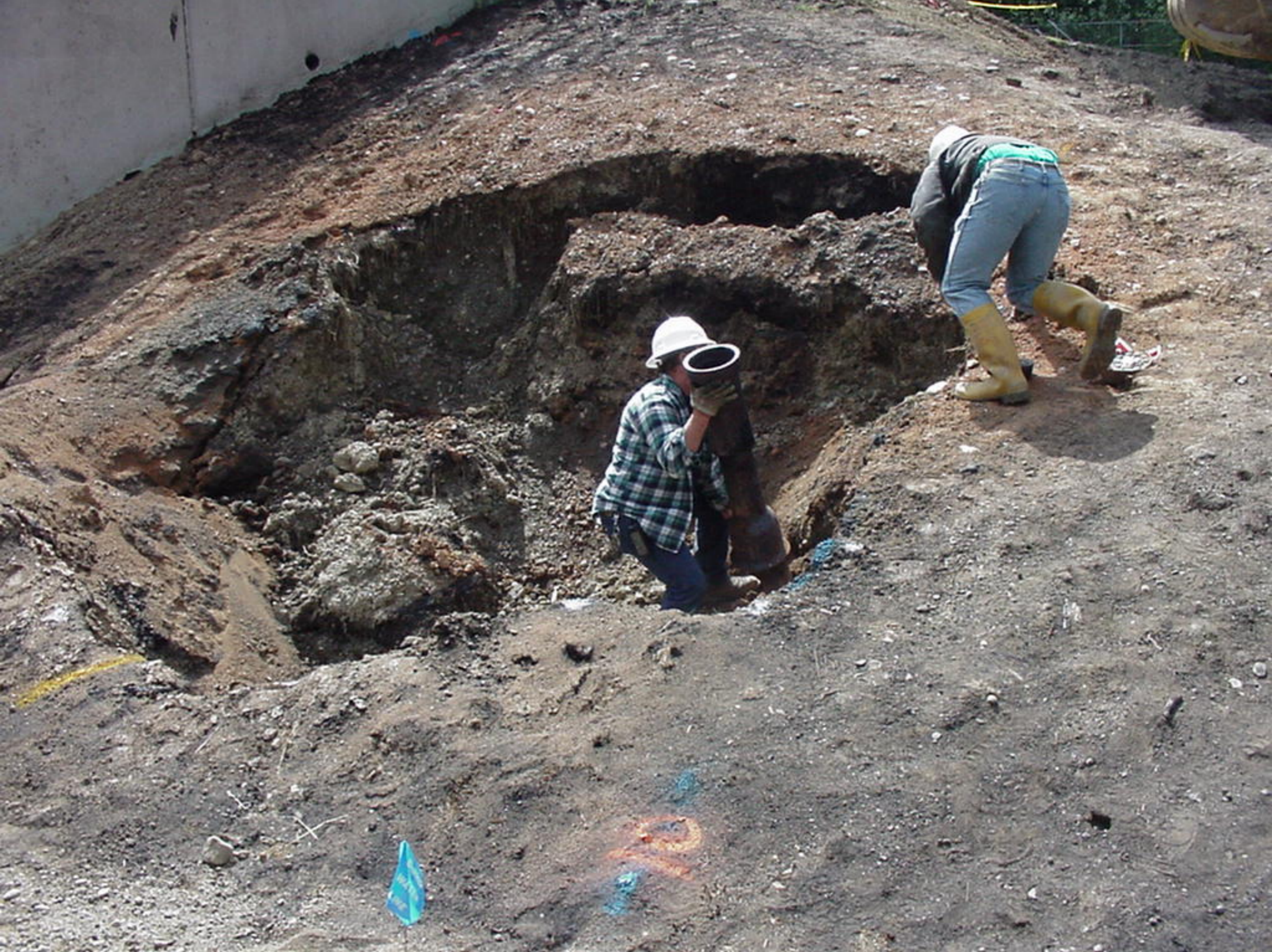
Appendix S to the Water Treatment Plant Factual Report, Photo 1, Post-accident crater with waterline valve risers.
