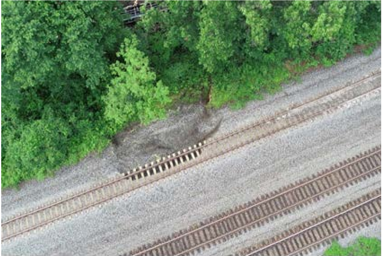
Figure 2. Aerial view of subgrade fill failure location on May 20th. Note additional degradation.
