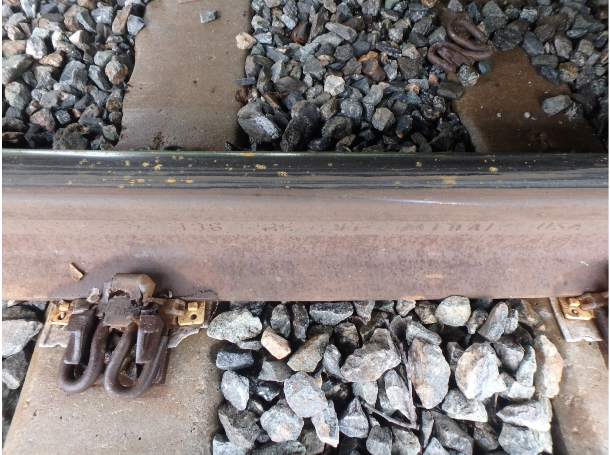
Figure 3. Photo showing the flange mark from a railcar wheel traversing over the top of the rail head in the curve at the location of the subsided subgrade.
