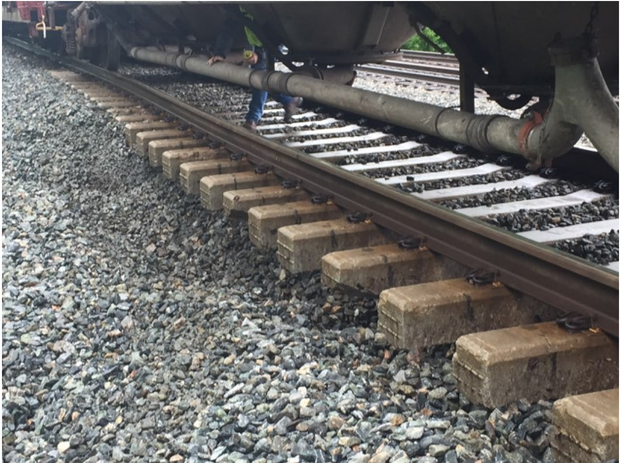
Figure 1. This photo shows the subgrade, fill-failure as it was about 4 hours after the derailment.
