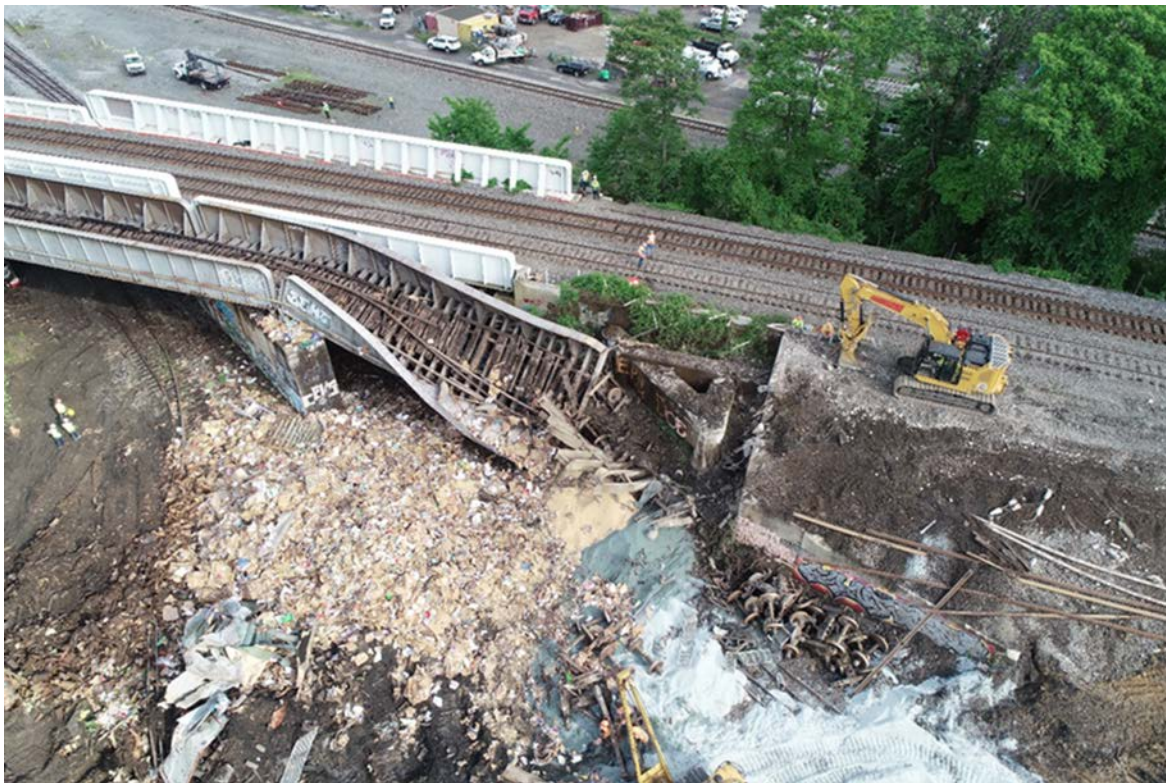
Figure 5. Aerial photo of displaced bridge structure. No. 1 track, MP CFP 102.8
