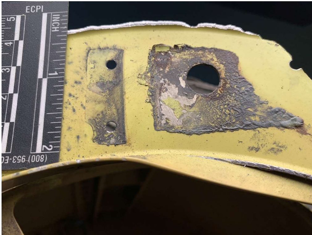
Figure 3. The aft fuselage bulkhead faying surface to which the upper-left longeron fitting's aft face contacted.
