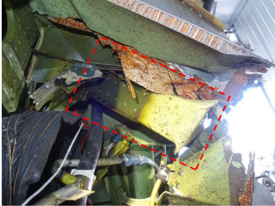
Figure 2. The upper-left longeron's connection to the engine pan longeron.
