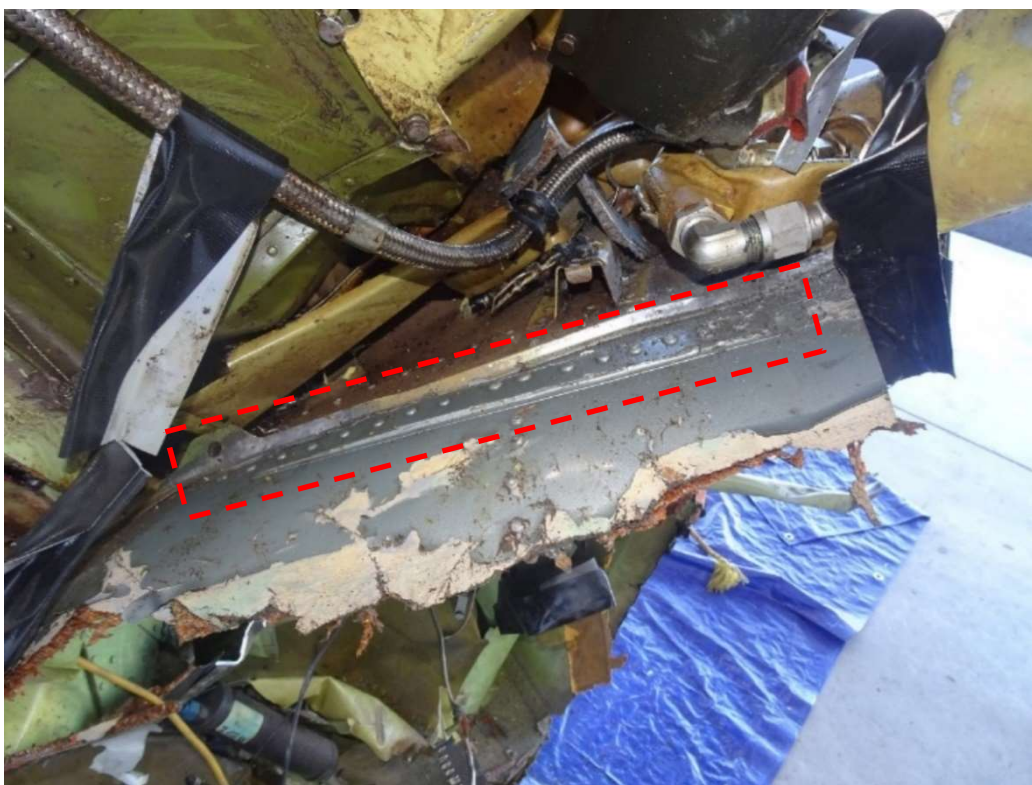
Figure 1. The strap doubler installation visible on the exterior of the aft fuselage.
