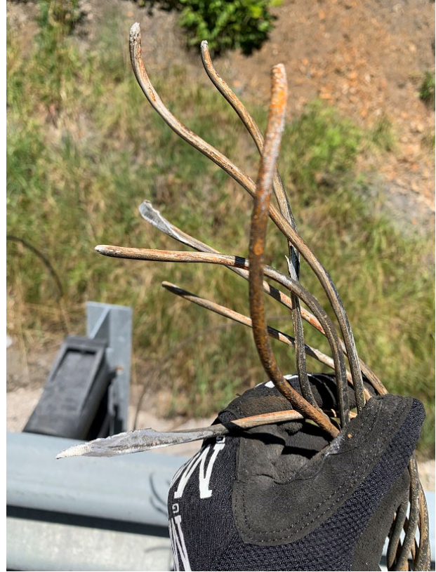
Figure 5. The severed end of the powerline about 397 feet away from the single suspended powerline.
