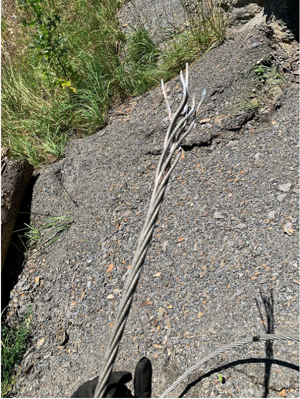
Figure 4. The severed end of powerline about 220 feet away from the single suspended powerline.
