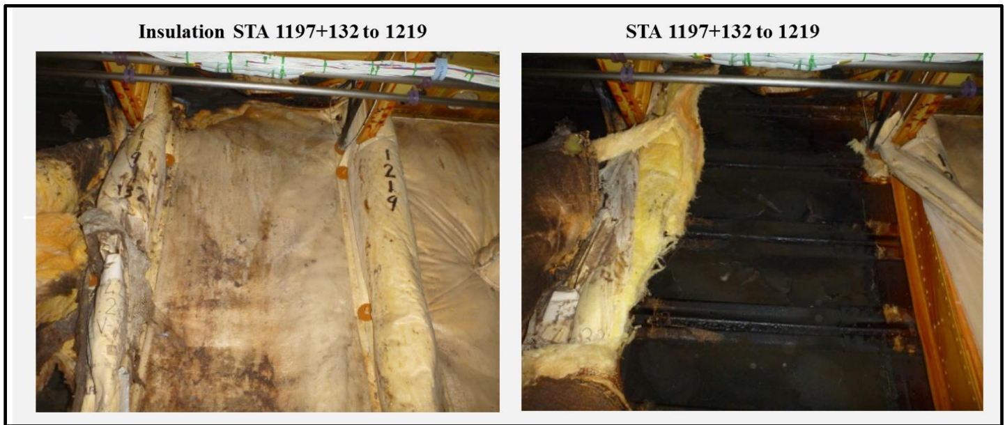
Figure 66 Insulation blanket damage
