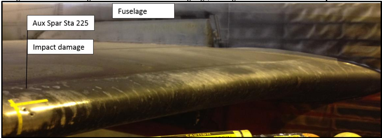
Figure 51 View of the right horizontal stabilizer leading edge, looking aft and inboard from aux spar station 230
