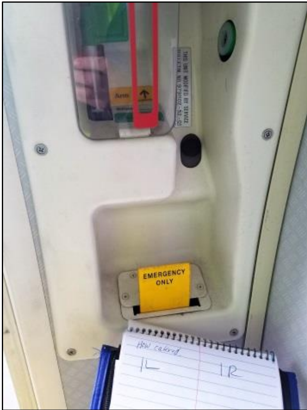
Figure 67 Door 1L was armed and open with ramp stand in place
