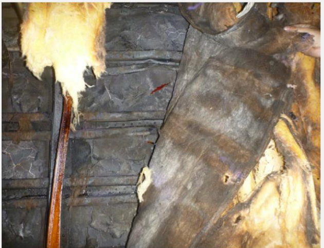
STA 1197+44 to 1197+66 (note the cracks)
