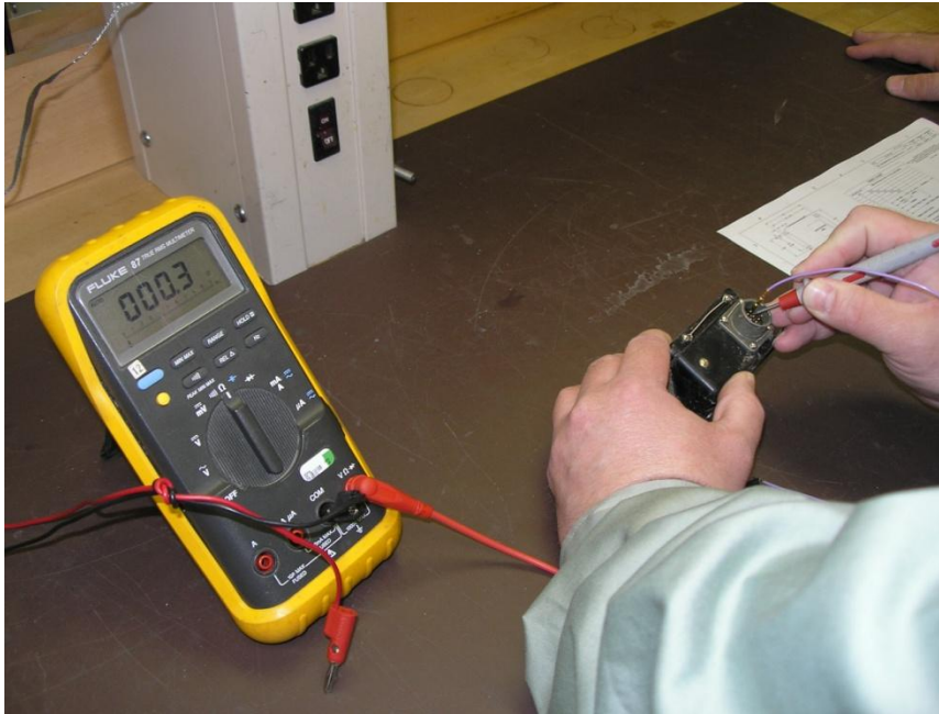
Figure 24 – Photo of Electrical Continuity Check of the Boots Deicing Timer Pin B to Pin J
