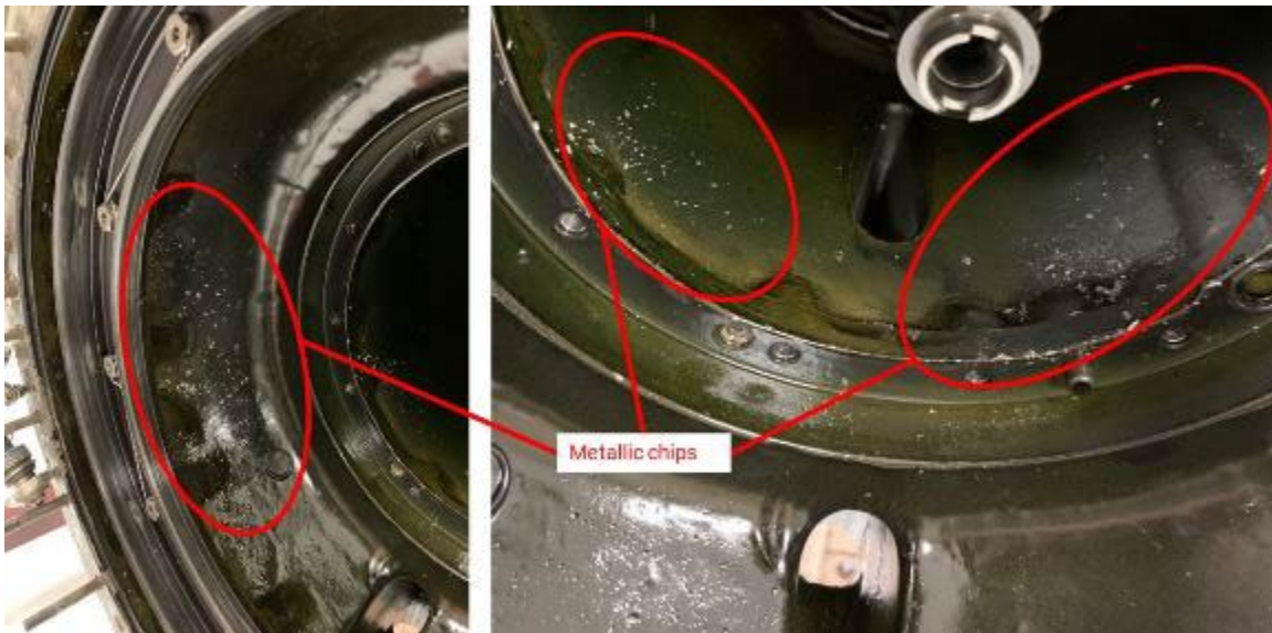
PHOTO 23: METALLIC FLAKES INSIDE THE REDUCTION CARRIER
