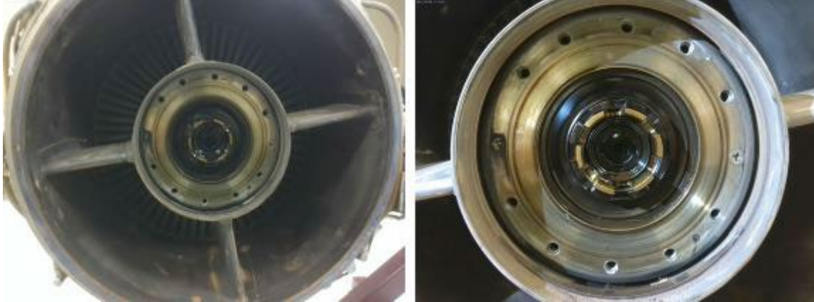
PHOTO 31: EXHAUST DIFFUSER HOUSING, SUPPORTS, AND RETAINING CUP
