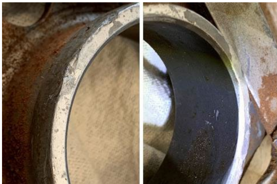
PHOTO 12: KAFLEX DRIVESHAFT COUPLING ENGINE END FITTING SHAFT
