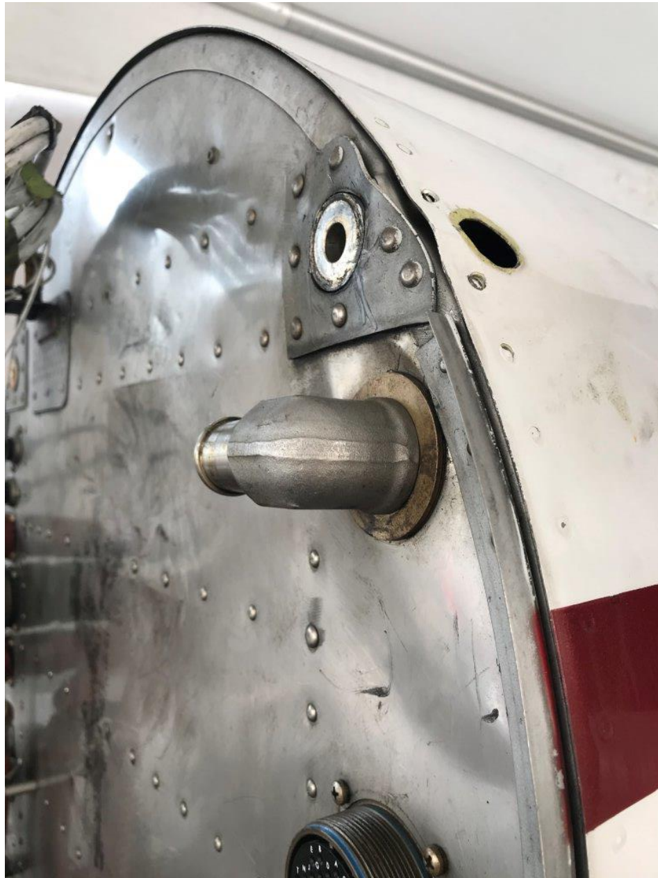
Photo 1 – View of engine mount damage (photo courtesy of the FAA).
