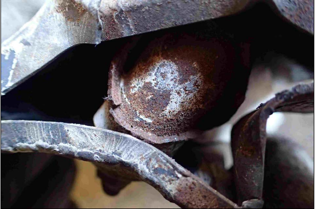
Photo 14 – Aft Control Stick Weldment at Bellcrank
