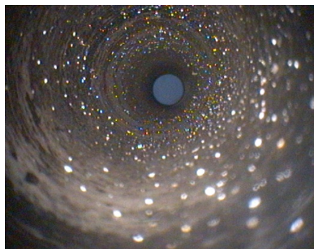
PHOTO 28: OIL SCAVENGE LINE
