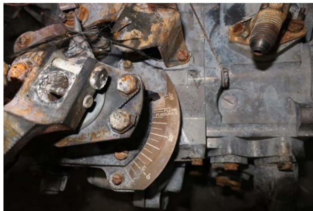
PHOTO 9: NO. 2 ENGINE FCU POSITION POINTER NEAR 62° POSITION
