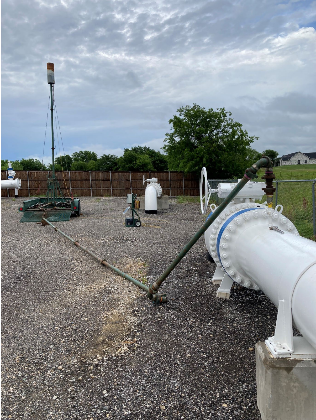
Figure 2. Flare System (6/28/2021 at 7:05PM, Courtesy of RRC)
