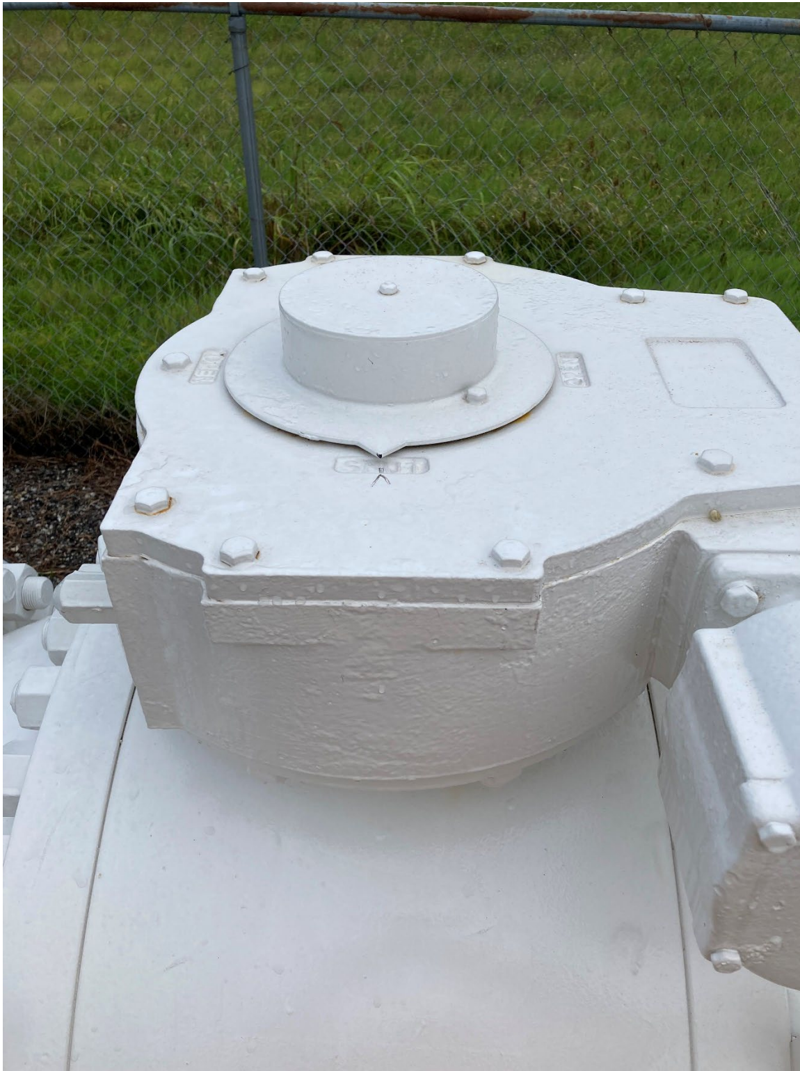
Figure 1. Indicator on Mainline Valve (6/28/2021 at 7:04PM, Courtesy of RRC)
