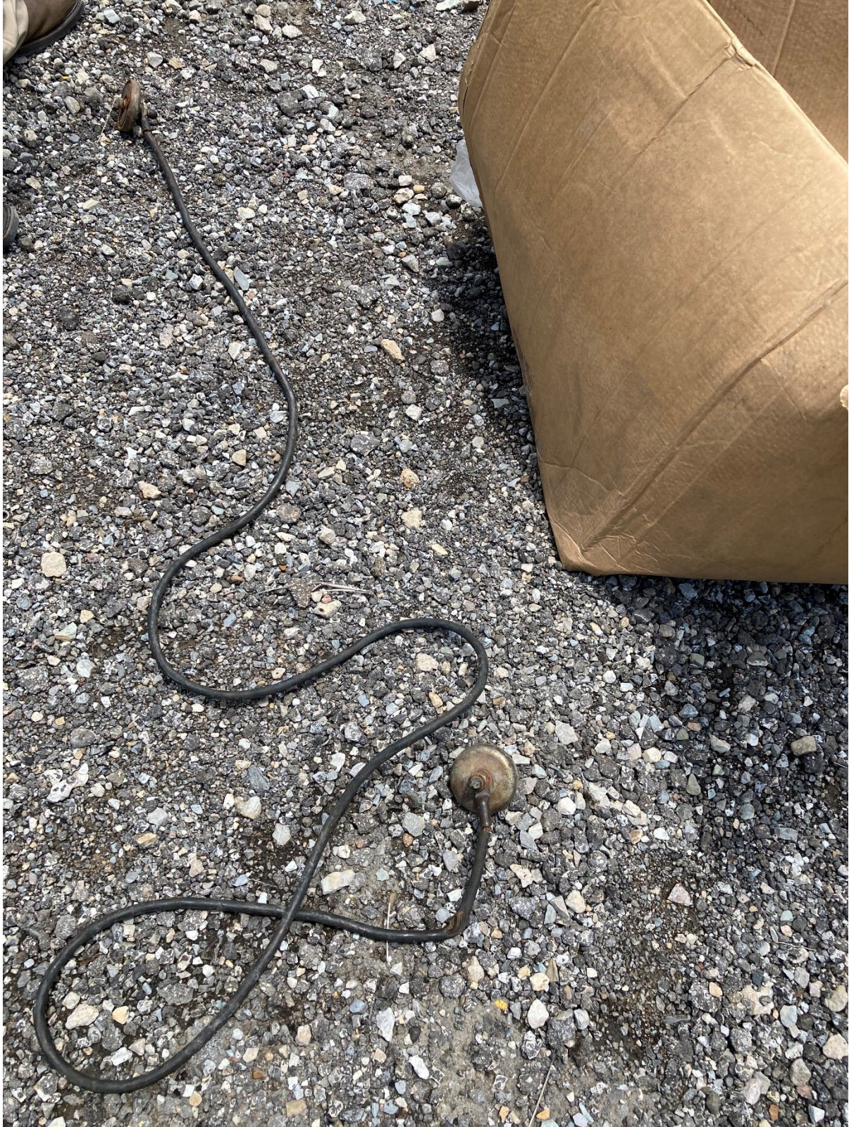
Figure 3. Grounding Cable (6/29/2021 at 1:10PM, Courtesy of RRC)
