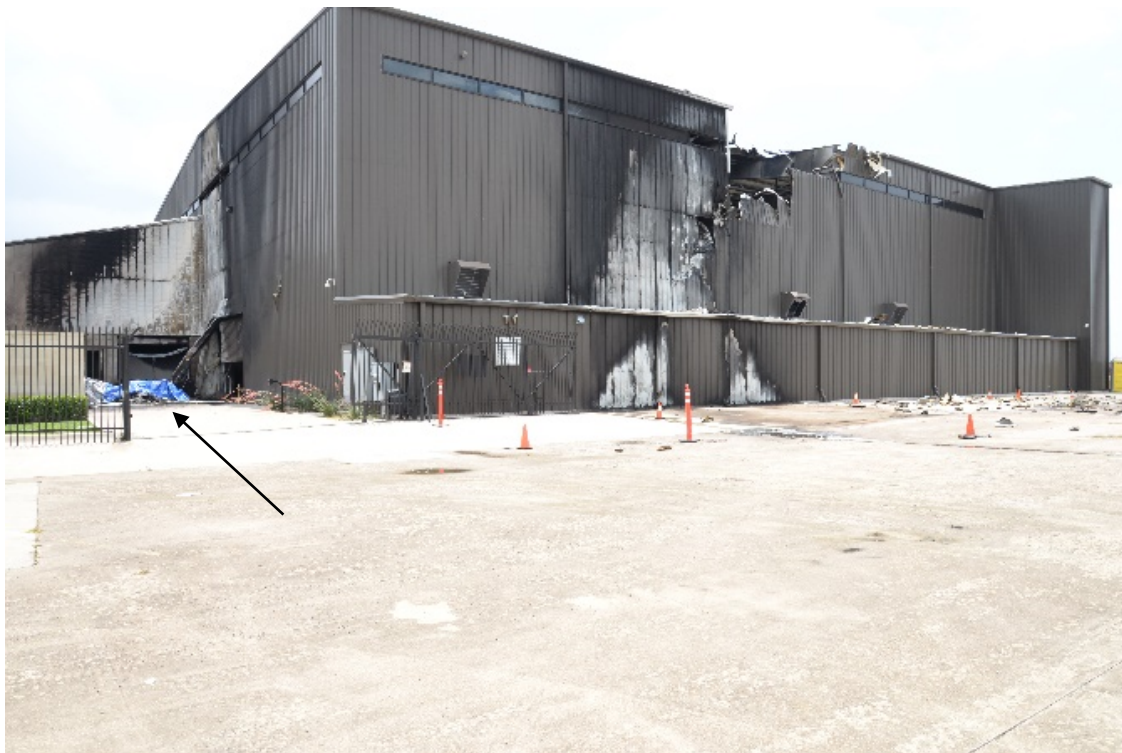
Photo 12. Ground view of the hangar impacted by accident airplane and airplane's final resting location.
