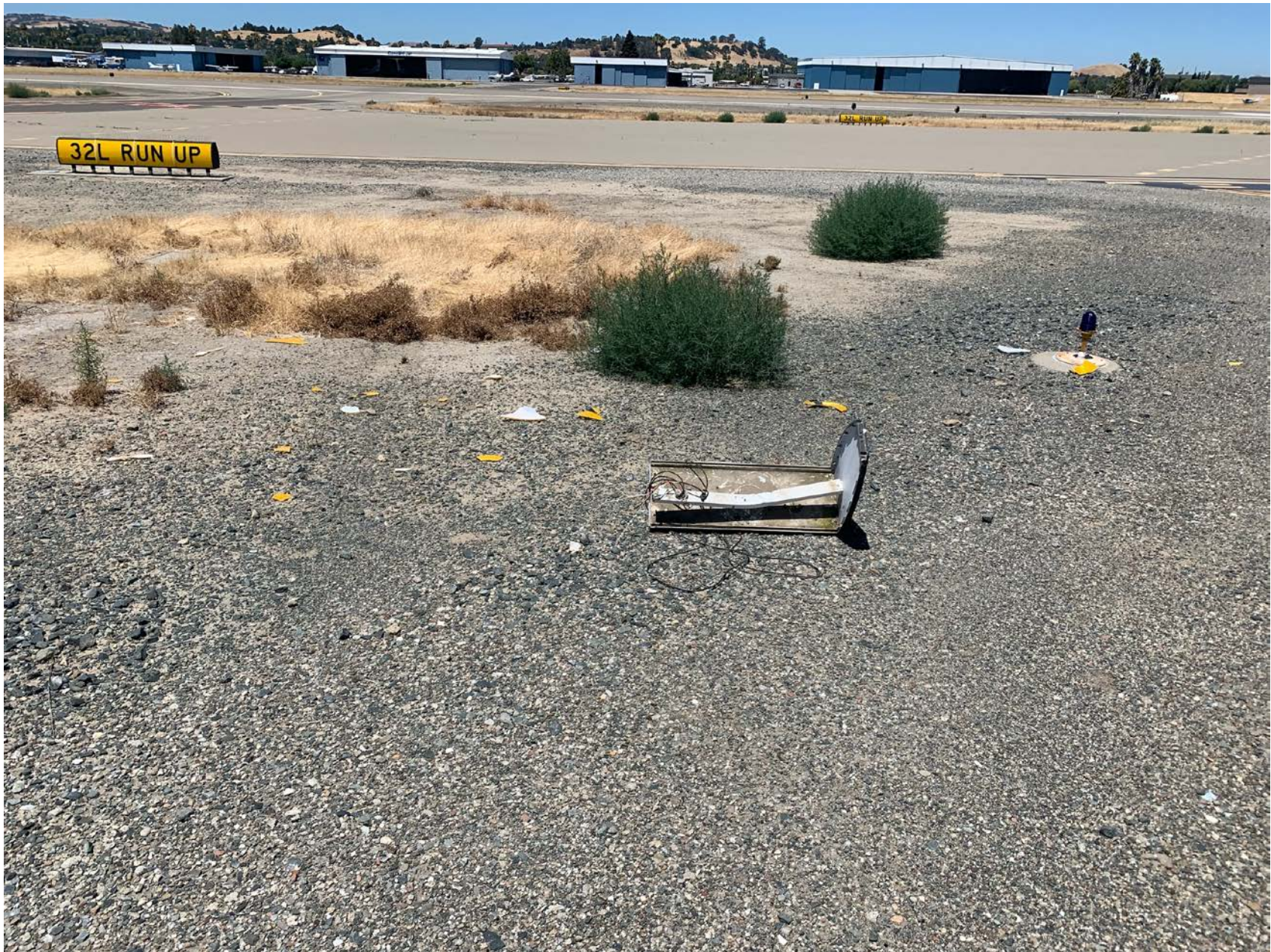
Photo 2 – View of damaged runway sign (courtesy of the FAA)
