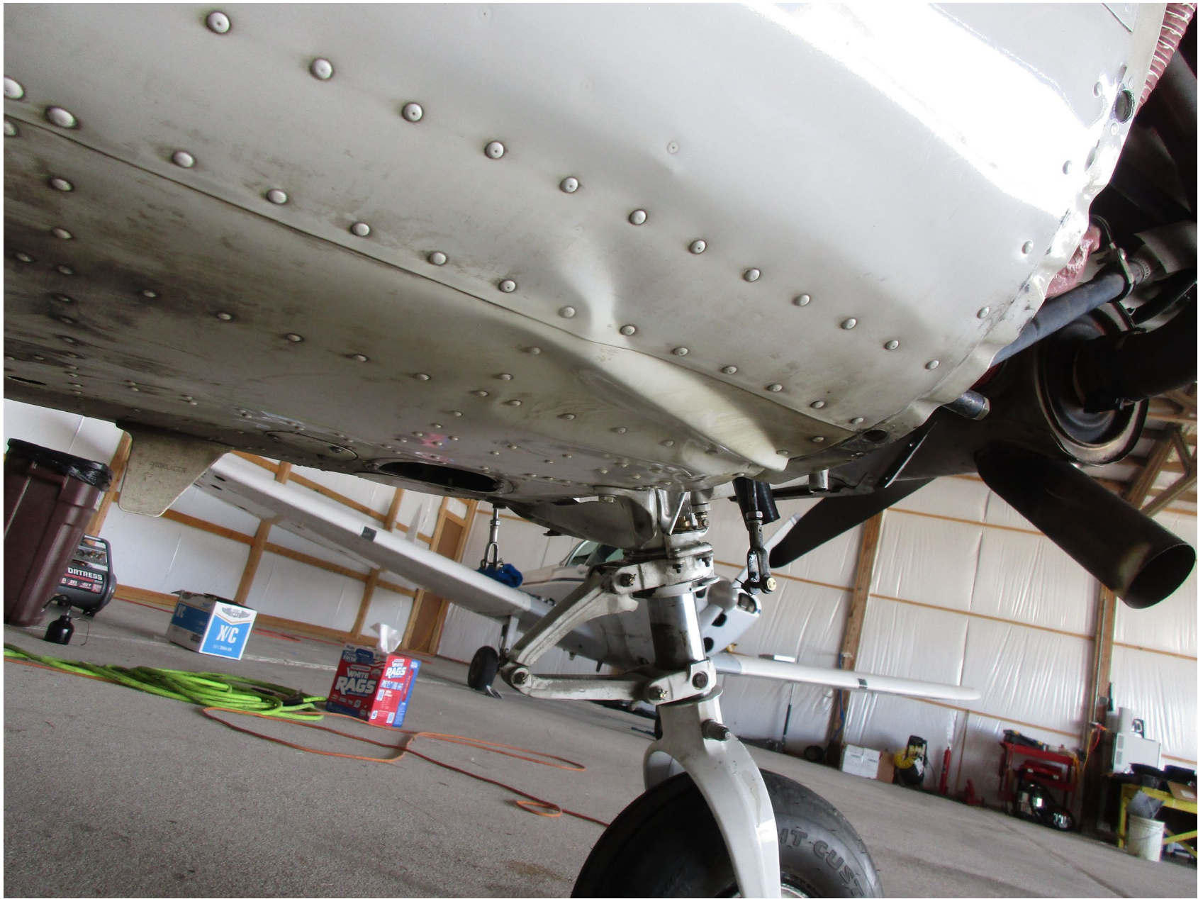
Photo 3 – View of the right side of the fuselage (courtesy of the Federal Aviation Administration).
