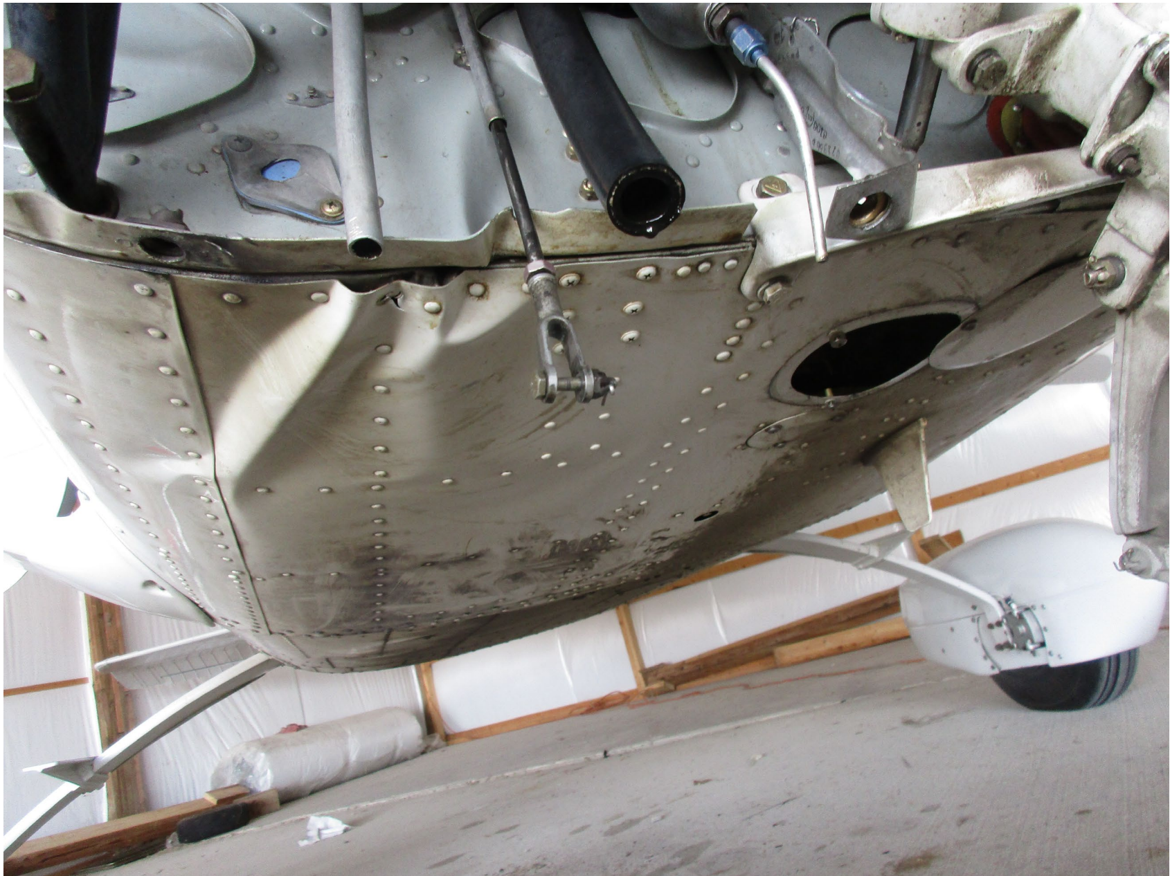
Photo 4 – View of the underside of the fuselage (courtesy of the Federal Aviation Administration).
